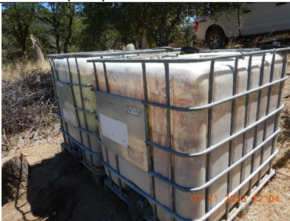
Photo 5 – Water storage tanks at WQ2
