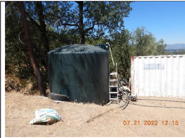
Photo 7 – Water storage tank at WQ9
