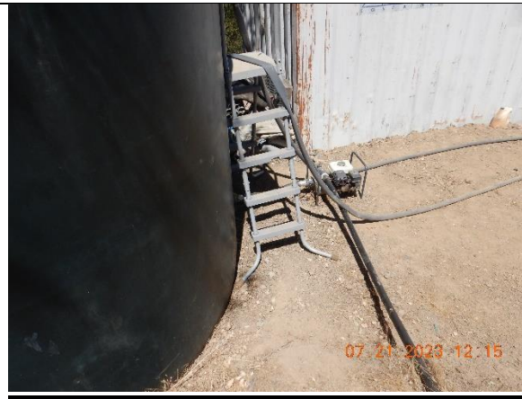
Photo 8 – uncontained pump at around WQ9
