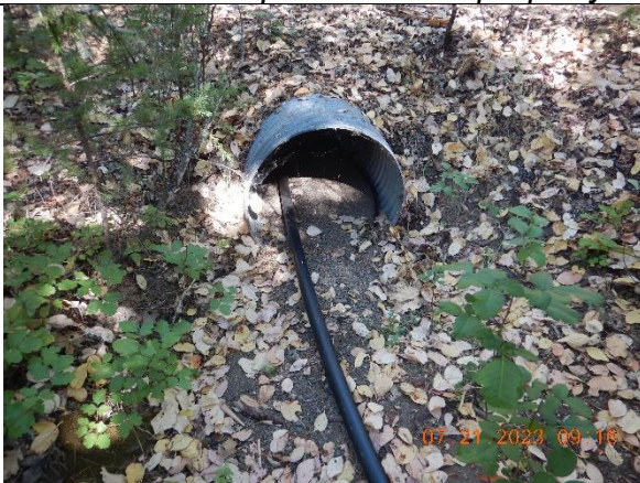
Photo 5 - partially clogged with sediment
