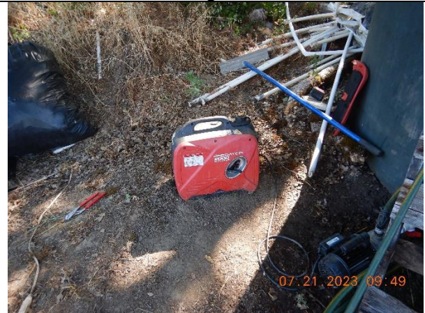
Photo 16 – uncontained battery powered generator near WQ14
