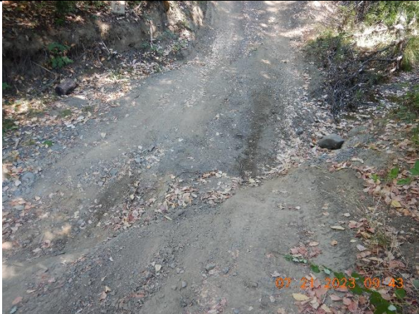
Photo 7 – A watercourse course crossing without any conveying structure at WQ12
