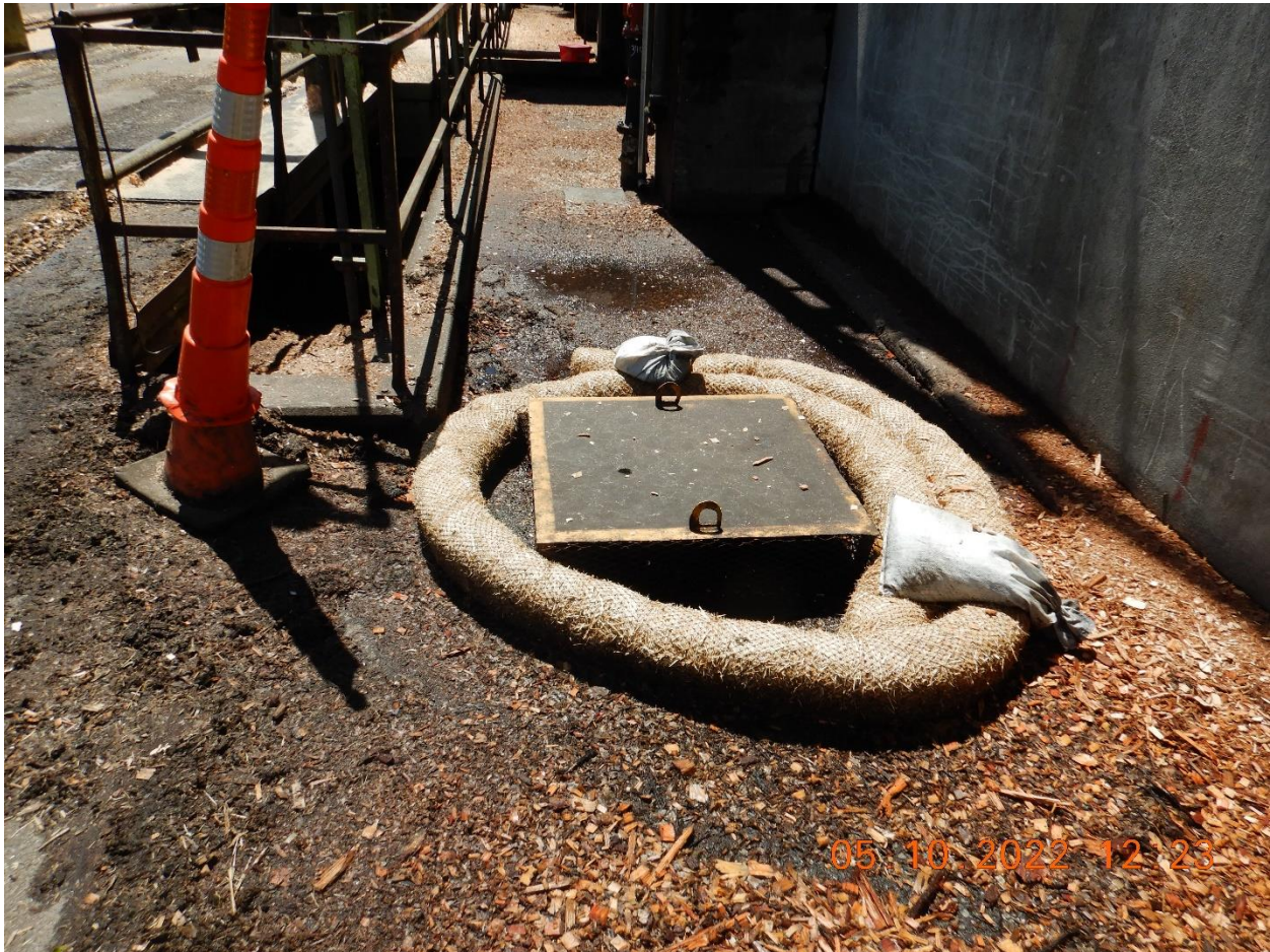
Picture 20d: Numerous storm drain inlets along the Planer Building that were not mapped on the site map. Picture taken by Farzad Kasmaei.
