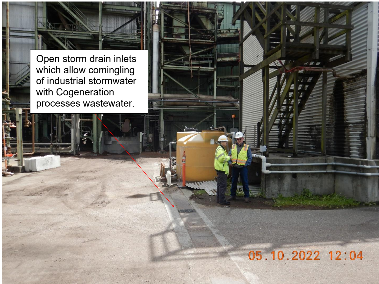
Picture 18b: Open storm drain inlets which allow comingling of industrial stormwater with Cogeneration processes wastewater. Picture taken by Farzad Kasmaei.
