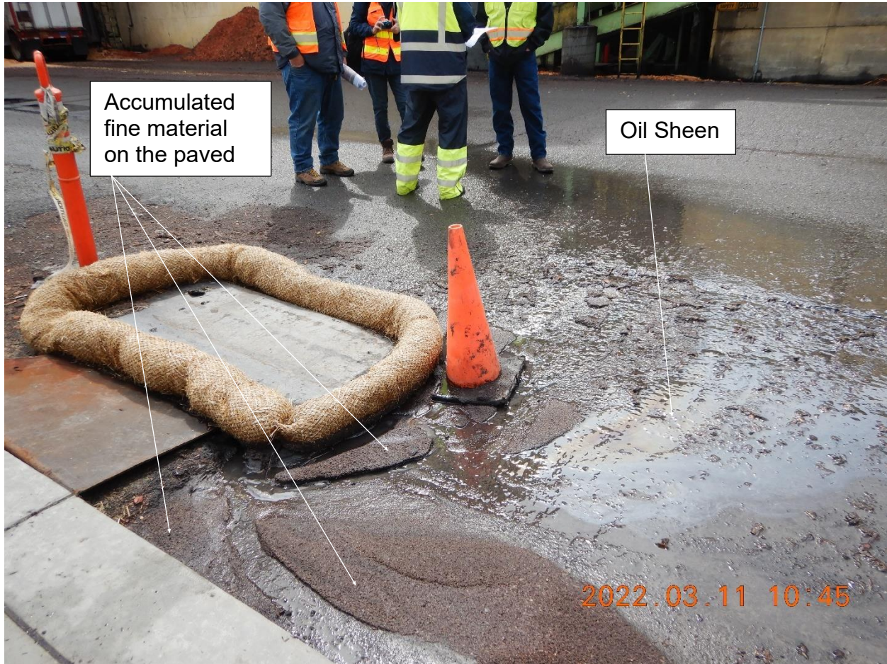
Picture 1e: Storm drain inlets within drainage area 1, with straw wattles incorrectly installed on pavement. Note the accumulated material on the paved surface that is so deep that erosion rills can be seen that demonstrated discharge is going under the straw wattle. Oil sheen be seen as well. Picture taken by Heaven Moore.
