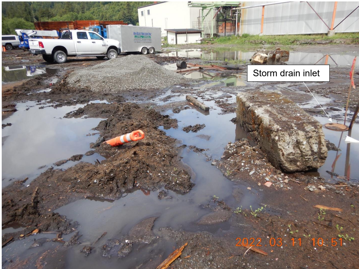
Picture 1h: A storm drain inlet is located within this area in drainage area 1. The storm drain inlet and the adjacent area is covered with many inches to feet of debris, mud, wood fiber, and unprotected stockpiled material. No housekeeping BMPs or inlet protection BMPs are present. Picture taken by Heaven Moore.
