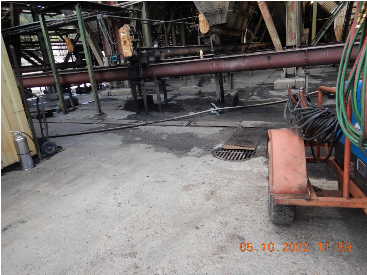
Picture 17b: View of the cogeneration operational area and a storm drain drop inlet within the paved area that drains to the Log Pond. Oil and hydrocarbons can be seen around and on top of the inlet. The area had a strong smell of hydrocarbons. This storm drain inlet discharges into the Log Pond. Picture taken by Farzad Kasmaei.
