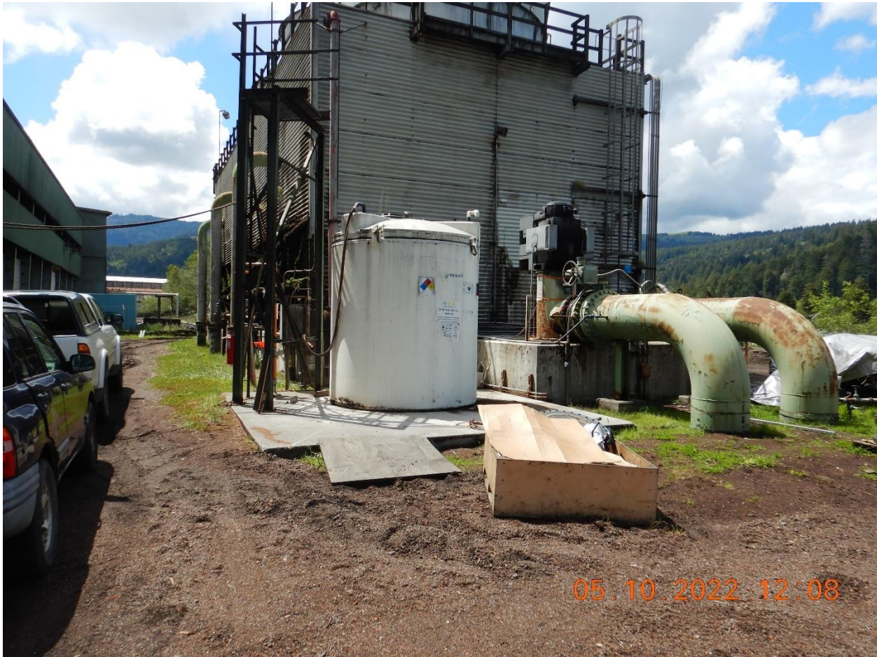
Picture 19c: Large hypochlorite chemical storage tank without secondary containment or any other BMPs. Located in the Cogeneration area adjacent to the Log Pond. Picture taken by Farzad Kasmaei.
