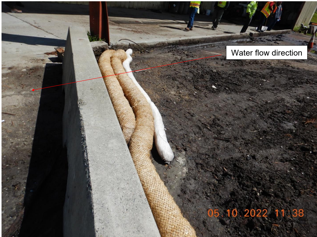
Picture 14c: Material that is washed from the equipment and vehicles on the pavement both within the designated area, as well as beyond the BMPs and concrete k-rail. Straw wattles and oil absorbing booms appear recently placed and are ineffective at containing the material. Water flow directions are shown with red arrows on the photo. Picture taken by Farzad Kasmaei.
