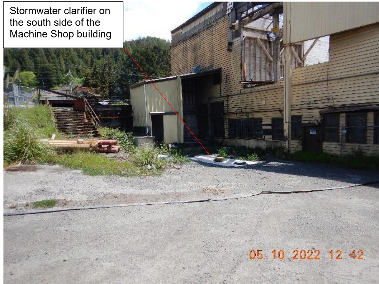
Picture 21a: Newly installed clarifier on the south side of the Machine Shop building where the samples are collected (SWDB 3B). Picture taken by Farzad Kasmaei.
