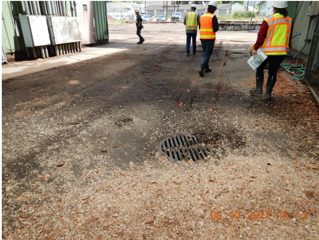
Picture 19d: View of unprotected storm drain inlet within Cogeneration area and significant amount of woodchips all around the inlet. Poor housekeeping is implemented within this area. Picture taken by Farzad Kasmaei.
