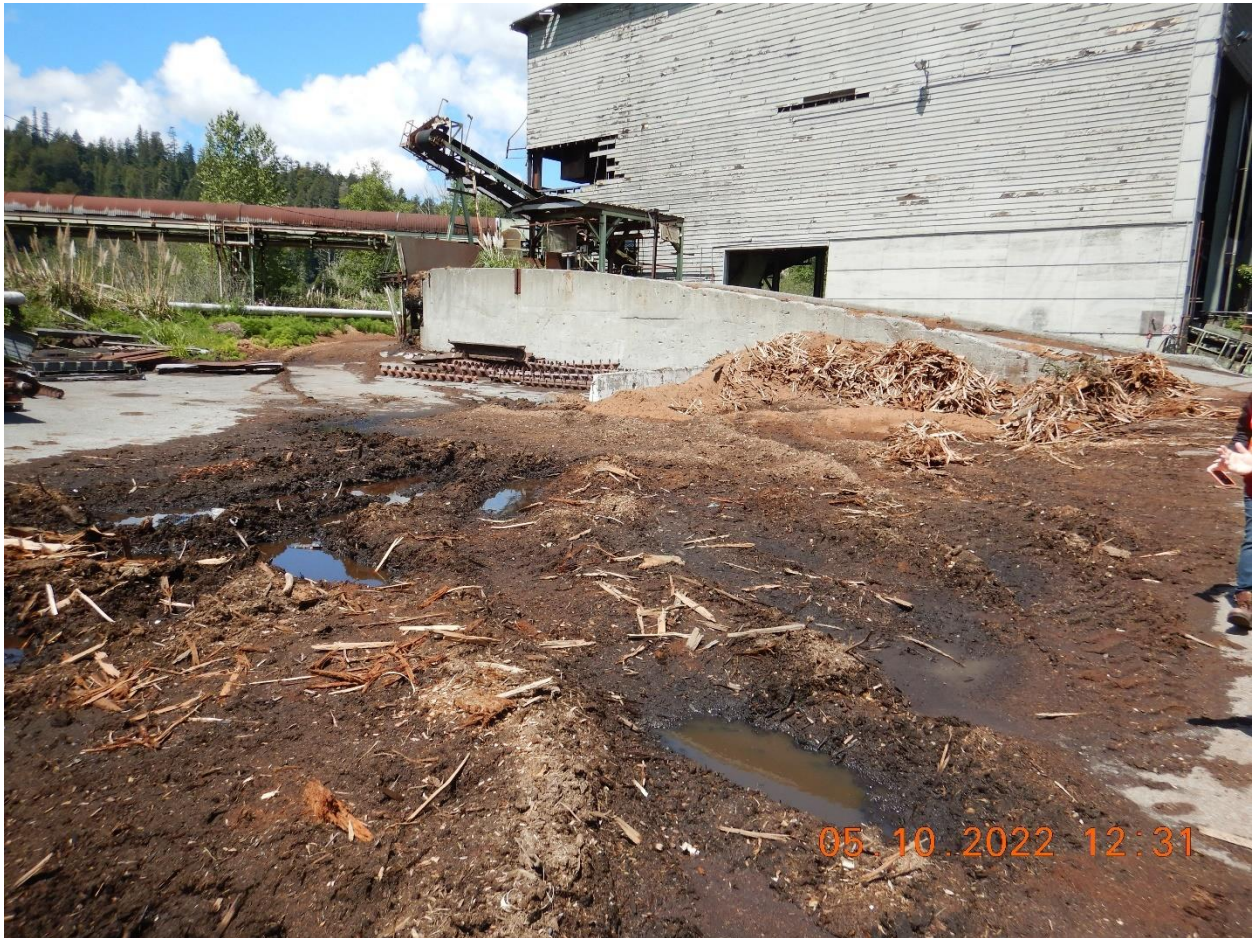
Picture 20b: Portion of Drainage Area 2. Wood chips and sawdust accumulations were observed outside throughout the yard as well as unprotected stockpiles. Picture taken by Farzad Kasmaei.
