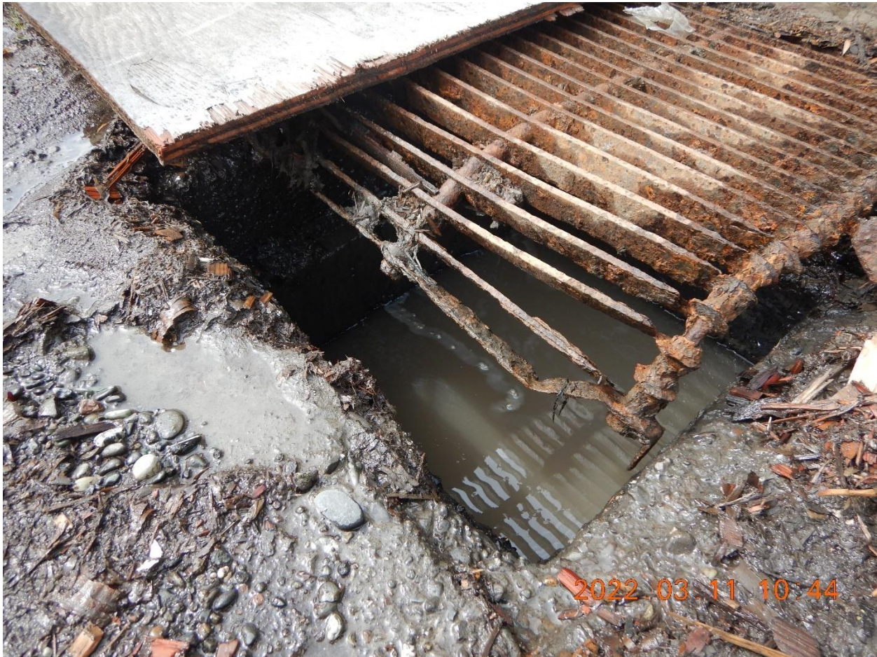
Picture 1c: Storm drain inlet within drainage area 1 observed receiving very muddy discharge, many with observable oil sheen and had no inlet protection BMPs. Picture taken by Heaven Moore.
