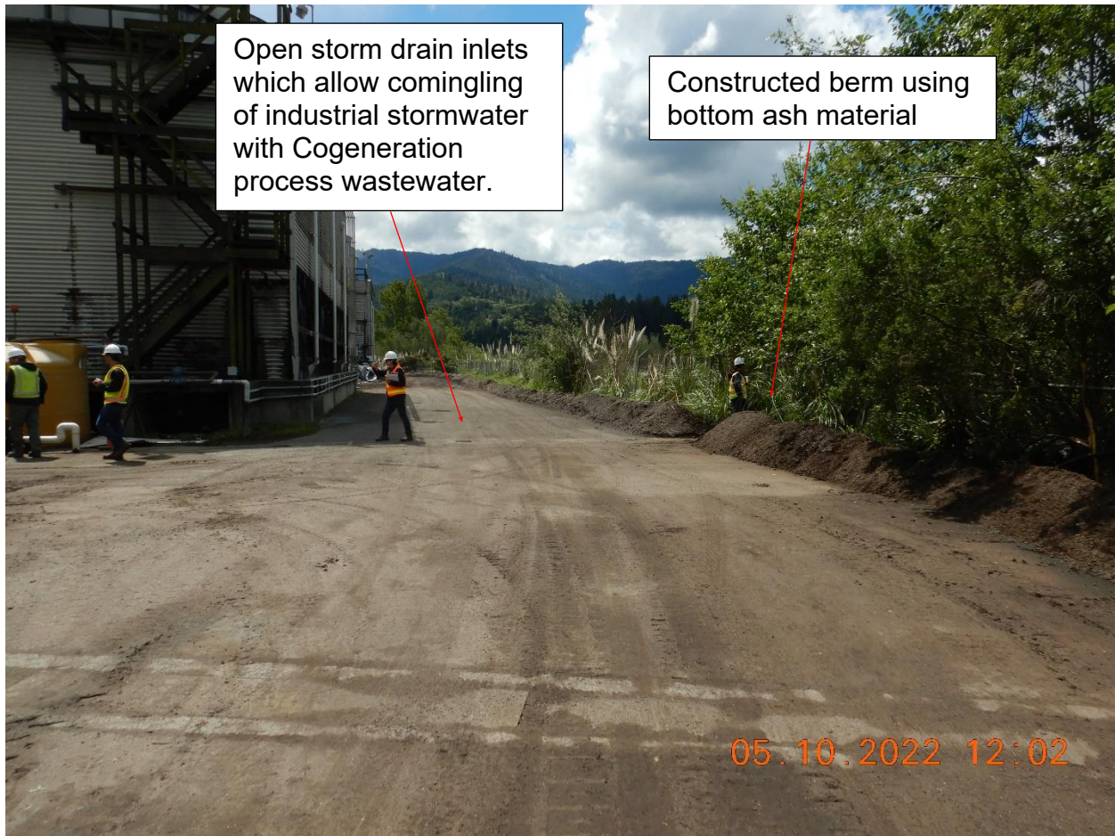
Picture 18c: Open storm drain inlets which allow comingling of industrial stormwater with Cogeneration processes wastewater. Berm constructed from bottom ash material the edge of the Log Pond. Picture taken by Farzad Kasmaei.
