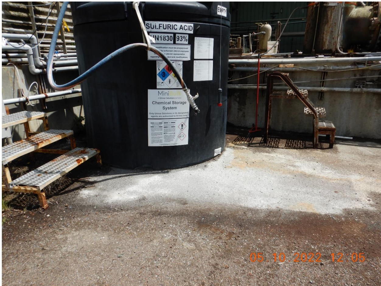
Picture 19a: Large sulfuric acid chemical storage tank without secondary containment or any other BMPs. Located in the Cogeneration area adjacent to the Log Pond. Picture taken by Farzad Kasmaei.
