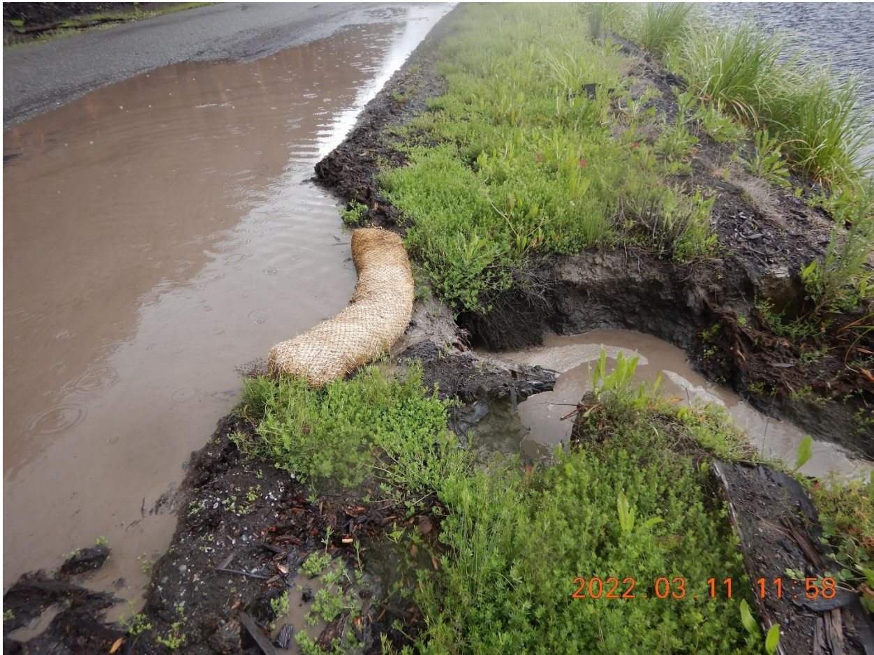
Picture 5f: View of runoff discharging into the retention pond from the access road along the north edge. The water appeared to be highly turbid, the bank was significantly incised, and the small piece of straw wattle appeared to be ineffective. Picture taken by Heaven Moore.
