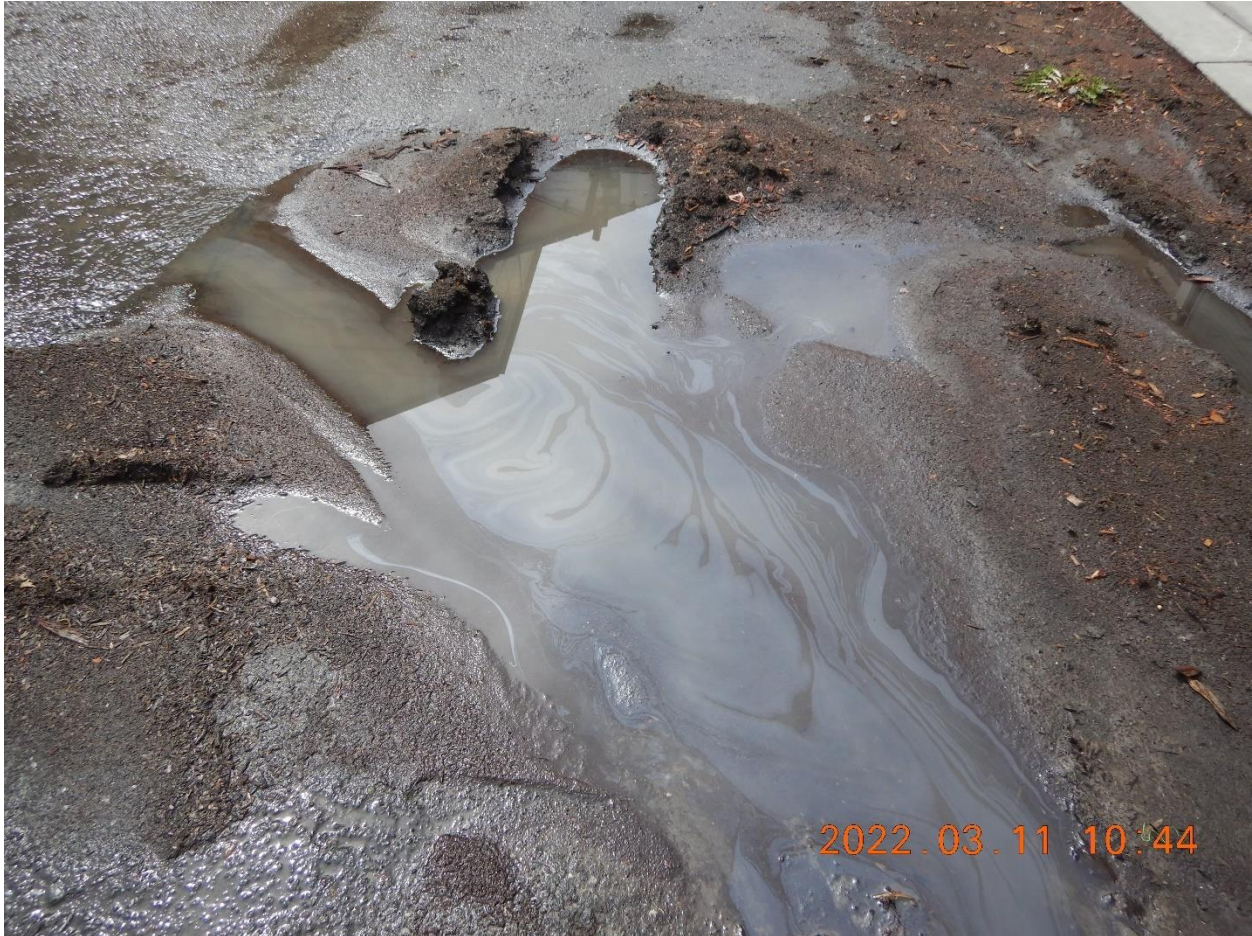
Picture 1d: Oil sheen upstream of storm drain inlet shown in Picture 1c above, which had no inlet protection BMPs. Picture taken by Heaven Moore.
