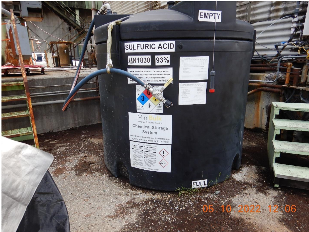
Picture 19b: Large sulfuric acid chemical storage tank without secondary containment or any other BMPs. Located in the Cogeneration area adjacent to the Log Pond. Picture taken by Farzad Kasmaei.
