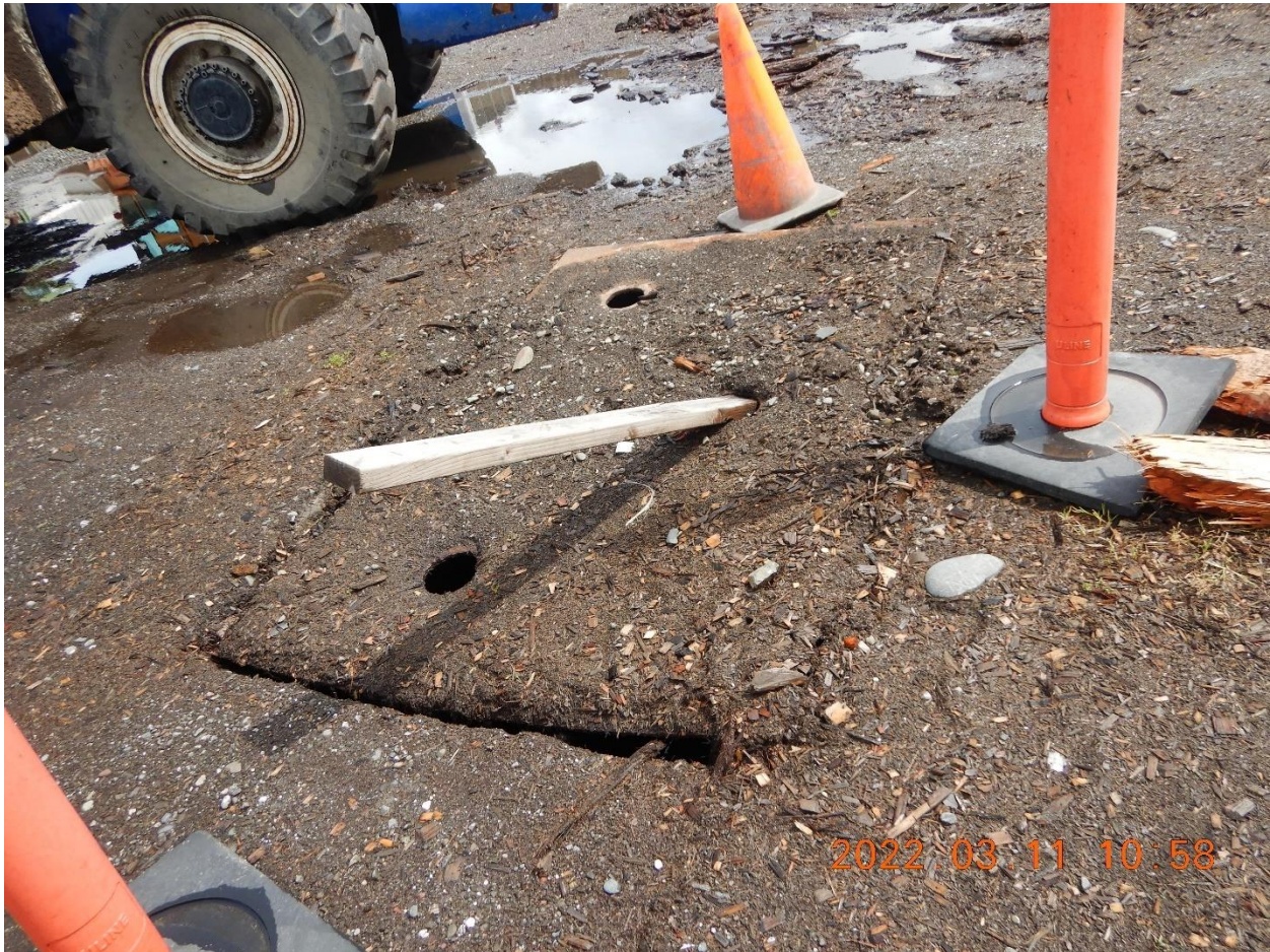
Picture 1i: Storm drain inlet within drainage area 1 observed with many inches of debris, mud, and wood fiber accumulated over the lid and adjacent to the inlet with no inlet protection BMPs. Note the piece of lumber inserted into the storm drain lid and that the lid is askew. Picture taken by Heaven Moore.
