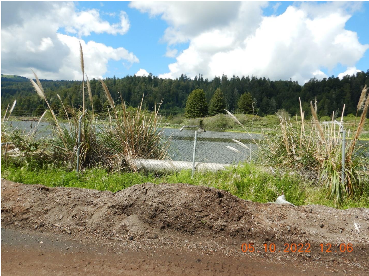
Picture 18e: Constructed berm made of bottom ash materials along the edge of the Log Pond. Picture taken by Farzad Kasmaei.
