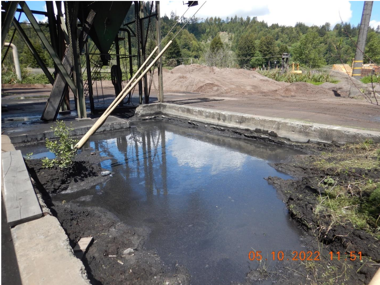
Picture 17a: Poned stormwater in the northeast side of the Cogeneration area. This area receives stormwater runoff from Cogen and outdoor vehicle wash areas shown in photos 14a-c. Thick dark mud and oil sheen was visible and the water had a strong hydrocarbon smell. This area discharges to downstream storm drain inlets and then into the Log Pond. The bottom ash stockpiles in the background are unprotected and would also discharge into the Log Pond. Picture taken by Farzad Kasmaei.
