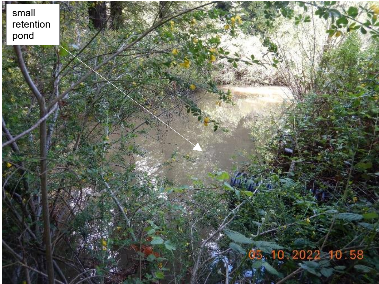
Picture 9c: Looking south at small retention pond in boneyard that receives runoff from upstream sediment traps via corrugated pipe shown on the photo. Picture taken by Farzad Kasmaei.
