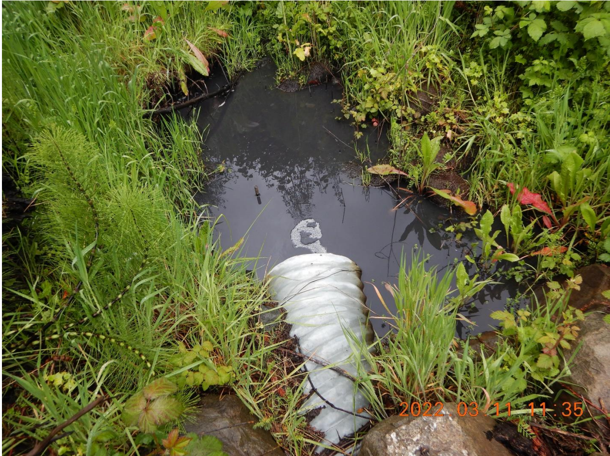
Picture 6e: Picture of the outlet pipe from the retention pond to the Eel River. The corrugated metal pipe is connected to the outlet structure controlled by the pulley suspended by the green cantilever structure and was open and discharging. The discharge appeared to be highly turbid, dark, and had gray hue. Foam was observed on the surface. Picture taken by Heaven Moore.
