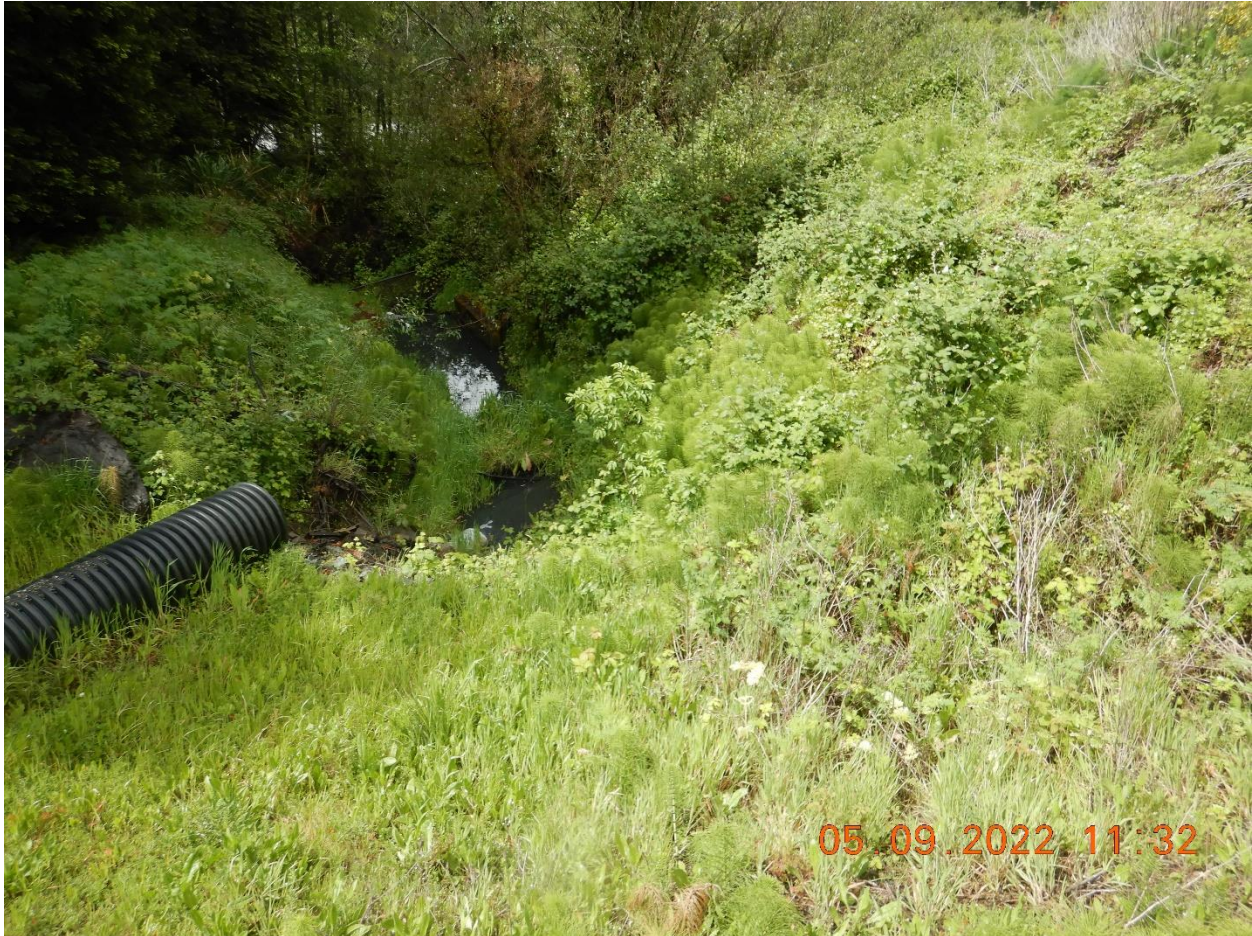
Picture 6c: Picture of the outlet pipes from the retention pond to the Eel River, which is visible in the background. The black corrugated plastic pipe is connected to the overflow with the red gate valve was closed at the time of inspection. The smaller corrugated metal pipe is connected to the outlet structure controlled by the pully suspended by the green cantilever structure and was open and discharging. Picture taken by Farzad Kasmaei.
