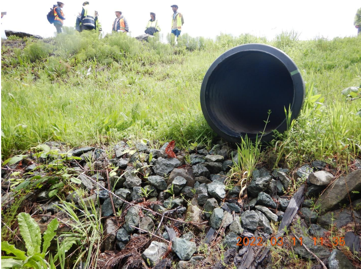
Picture 6d: Picture of the black corrugated plastic pipe that is connected to the overflow with the red gate valve was closed at the time of inspection. Picture taken by Heaven Moore.
