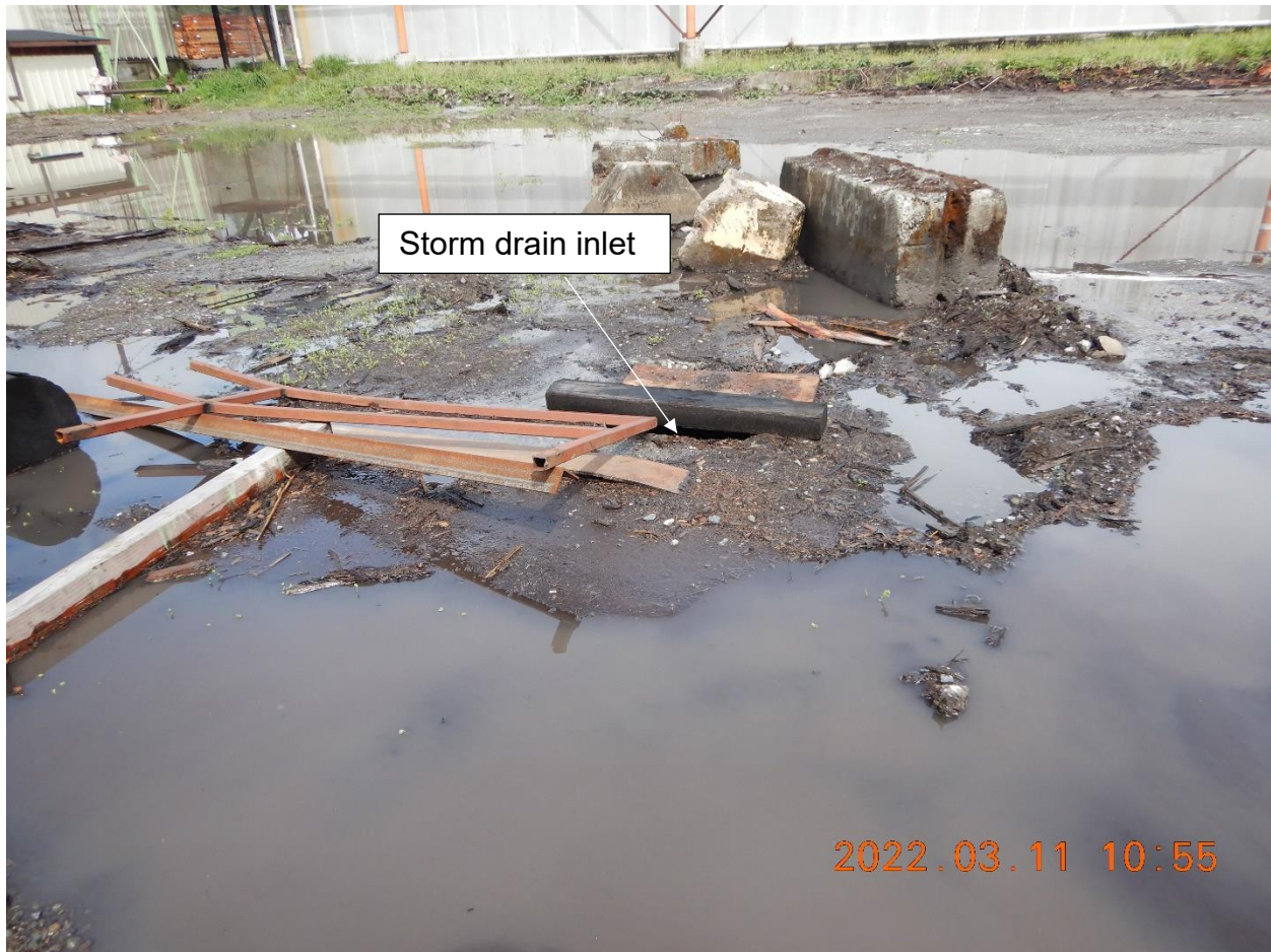
Picture 1j: A storm drain inlet is located within drainage area 1. The storm drain inlet and the adjacent area is covered with many inches to feet of debris, mud, wood fiber, and unprotected stockpiled material. No housekeeping BMPs or inlet protection BMPs are present. Picture taken by Heaven Moore.
