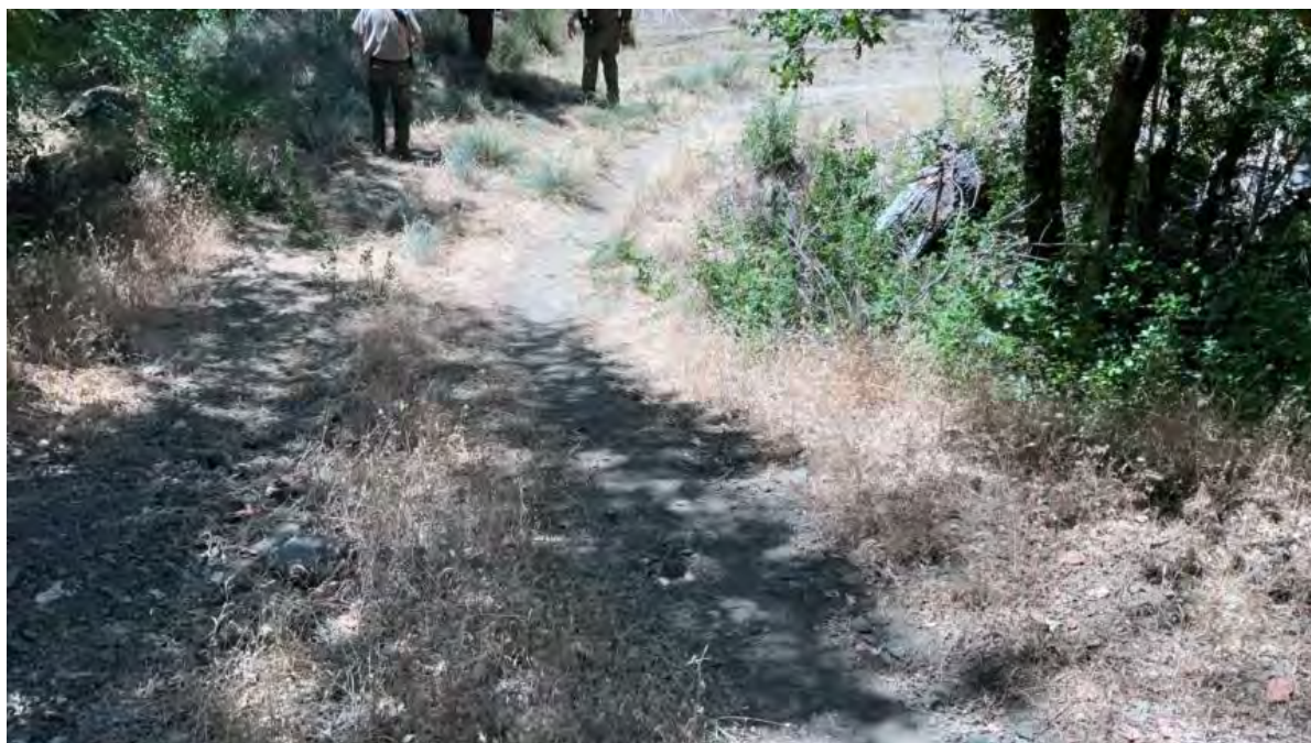
Figure 20. Point 5. Watercourse crossing on access road to west side of blue line watercourse used to access cannabis cultivation areas. The road approach concentrates runoff to the watercourse at the crossing and is a threatened discharge of waste.
