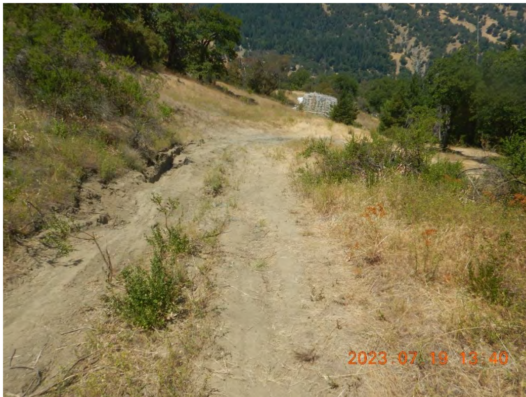
Figure 24. Road to western cultivation areas is rutted and has not been maintained.
