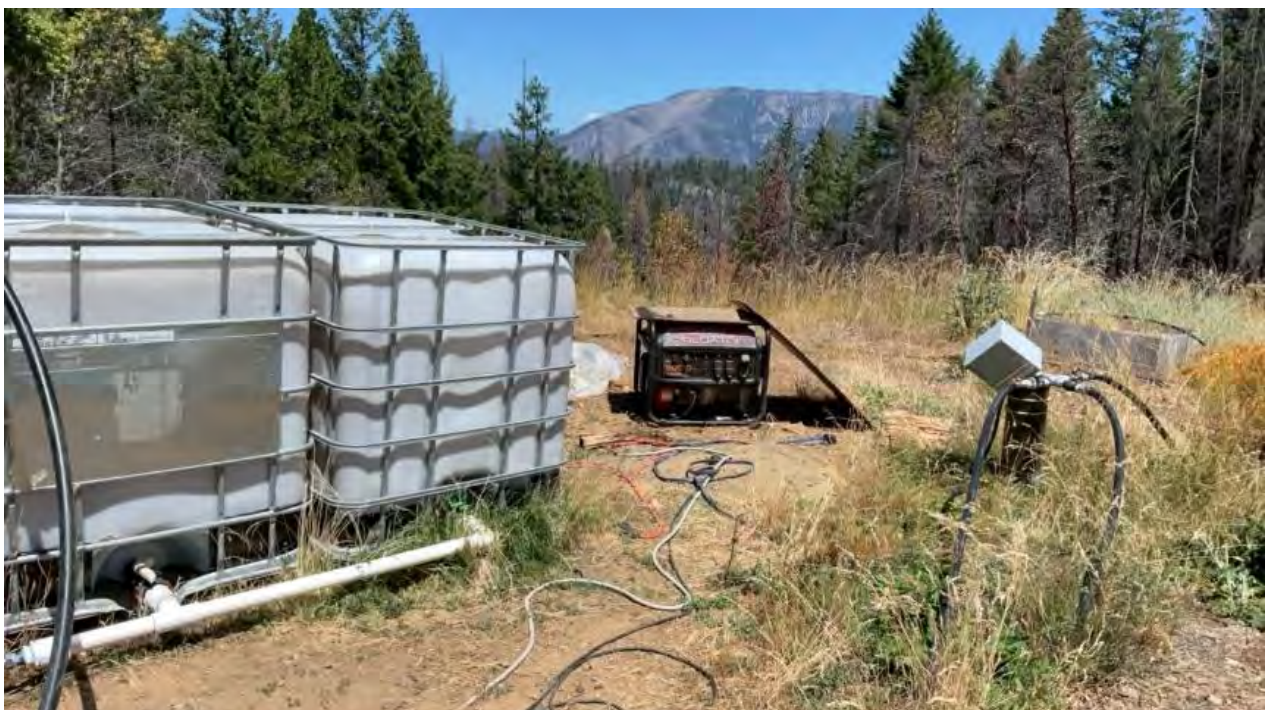
Figure 9. Polygon Feature 2 – Well, generator for pump and feed tanks located at the edge of the cultivation area flat.
