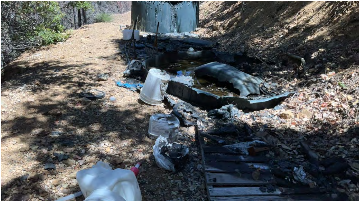
Figure 21. Polygon Feature 11 – water tanks melted from Monument Fire in 2021.
