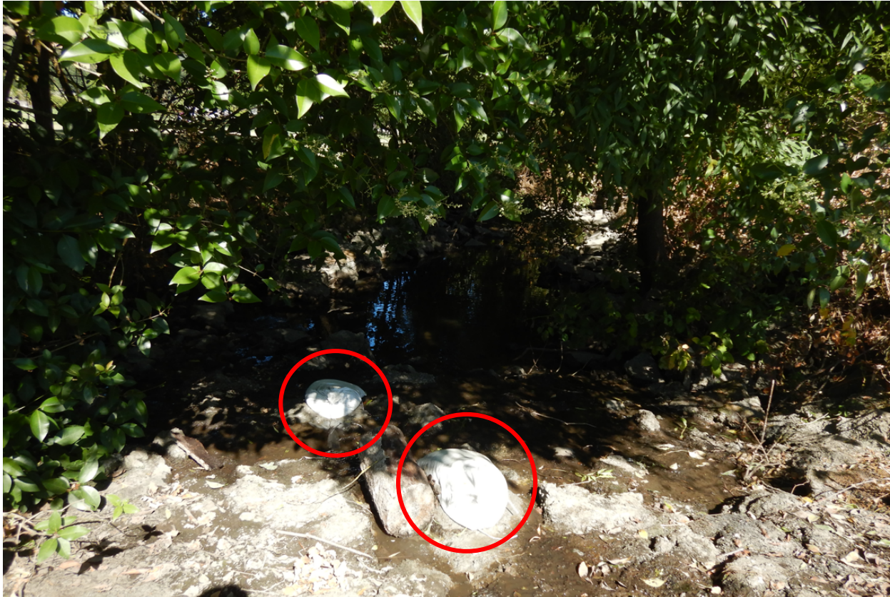
Photograph 3: Two holes in the dam apron that leaked a large quantity of water were plugged with pre-mix Sakrete concrete. White plastic sandbags were placed over the curing concrete (circled in red). Residual moisture is shown adjacent to the curing concrete.
