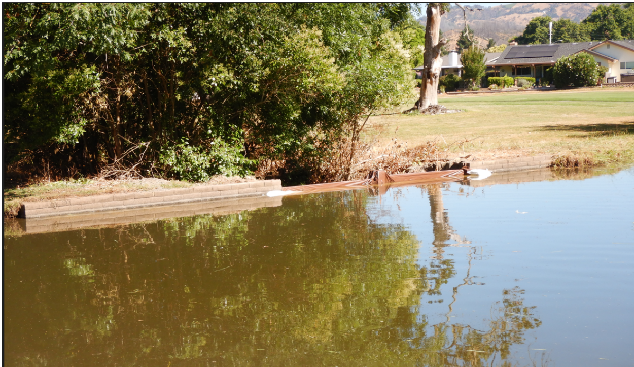
Photograph 1: Photographer is looking downstream at the flashboard dam. The photograph shows the irrigation pond, the two wing walls, and wooden flashboard dam. The flashboards have been recently covered with a brown tarp to help prevent water leakage.
