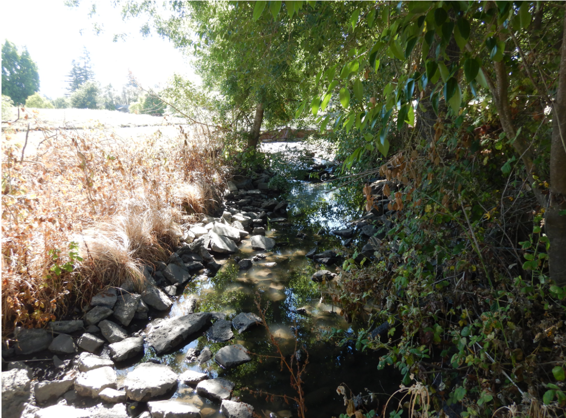
Photograph 5: Photographer is standing on the Santa Rosa Creek bank and looking upstream at Santa Rosa Creek channel hardened with broken concrete.
