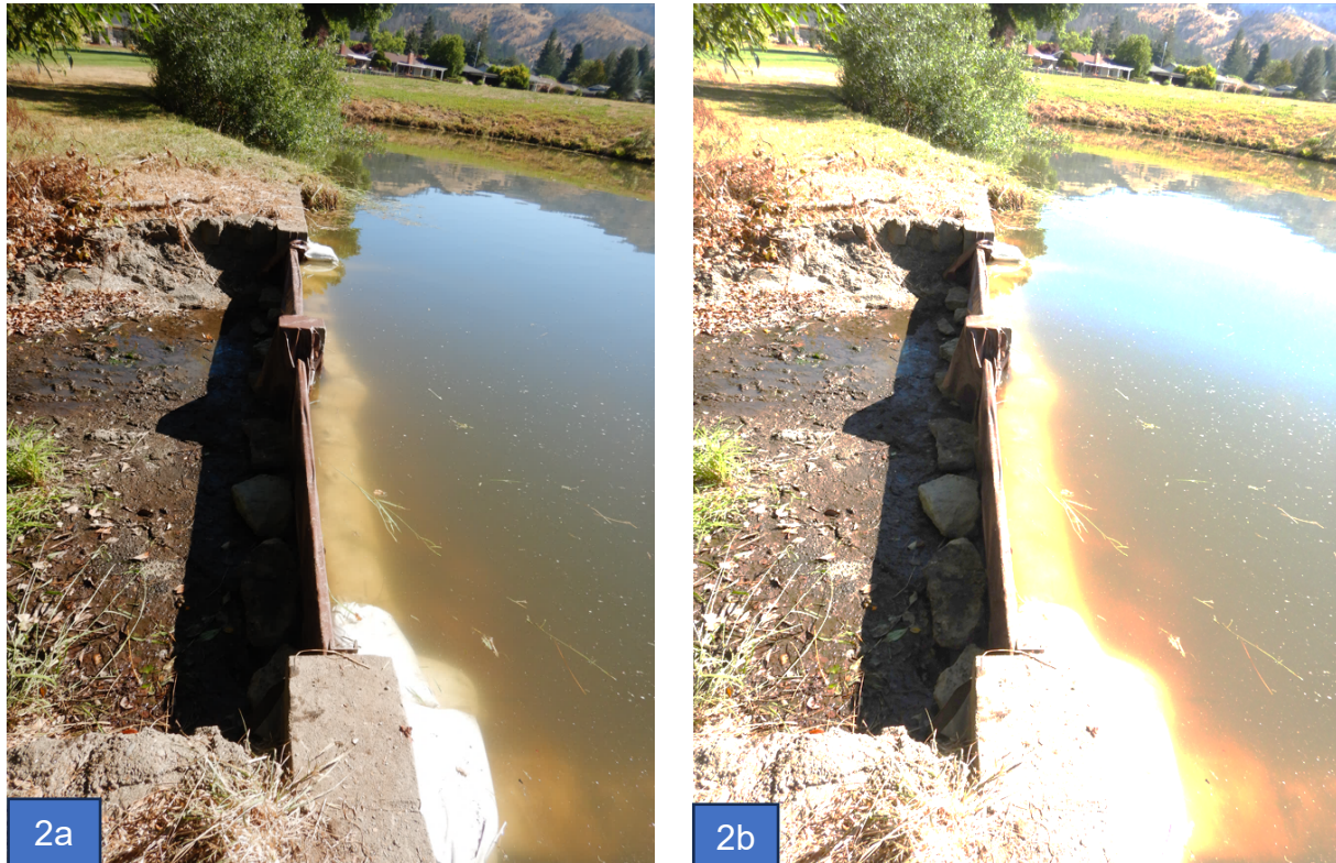
Photographs 2a and 2b: Brown plastic tarp is placed over the flashboard dam and concrete foundation and weighted down using 60 sandbags along the interior and broken concrete along the exterior of the dam. The photograph on the left (Photograph 2a) does not show the broken concrete because it is the dark shadow of the dam. The significantly lightened photograph on the right (Photograph 2b) shows the broken concrete along the dam's exterior and sandbags on the interior of the dam.
