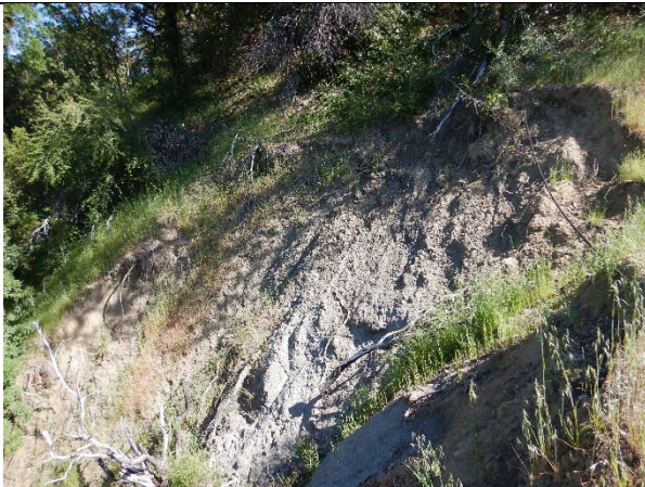
Photo 43 – Slope failure at WQ17
