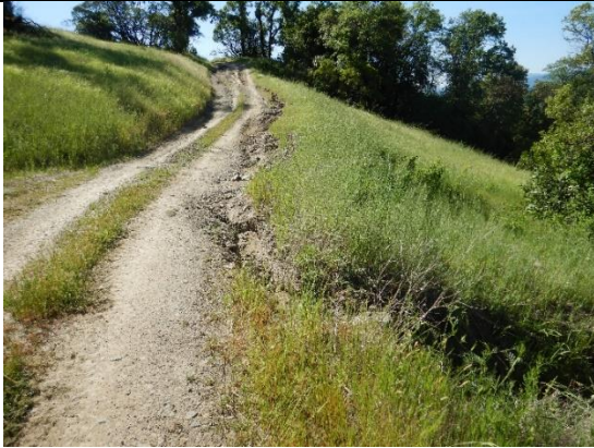
Photo 13- Hydrologically connected and eroded road section at WQ13
