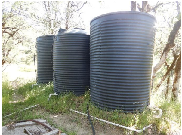
Photo 28 - Water storage tanks at WQ22
