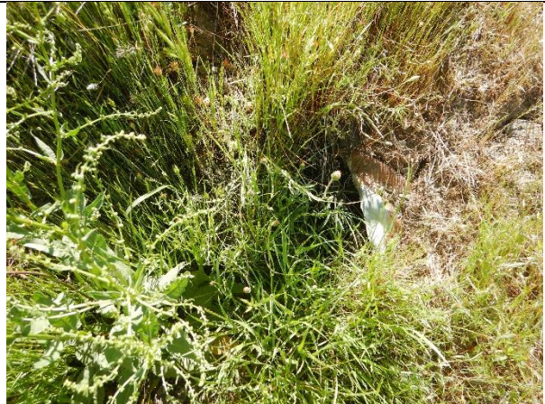
Photo 18 – Inlet of a culverted stream crossing at WQ13
