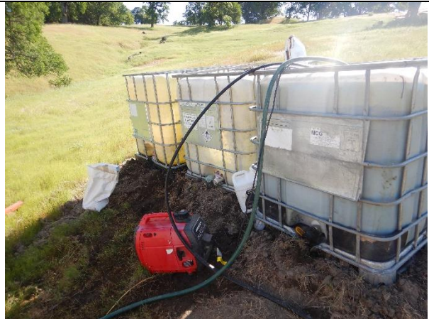
Photo 26 - Water storage tank at WQ6
