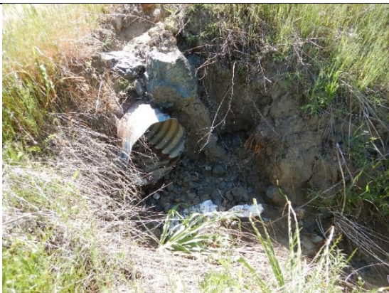
Photo 21– Outlet of the culvert at WQ14, installed high in the fill and eroding the stream bank
