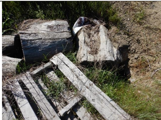
Photo 16 – Wood covering the inlet of a culverted stream crossing at WQ12
