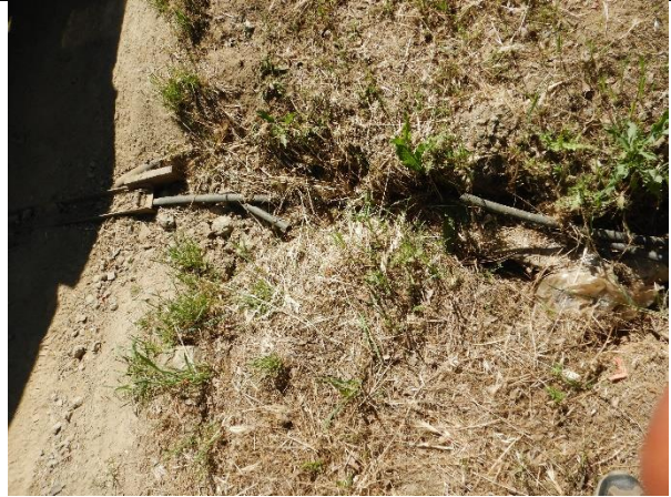
Photo 24 - Outlet of the culvert at WQ28, buried
