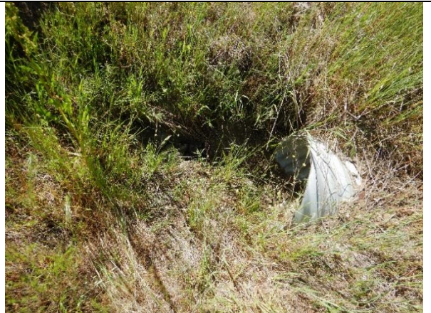
Photo 20 – Inlet of a culverted stream crossing at WQ14, partially clogged
