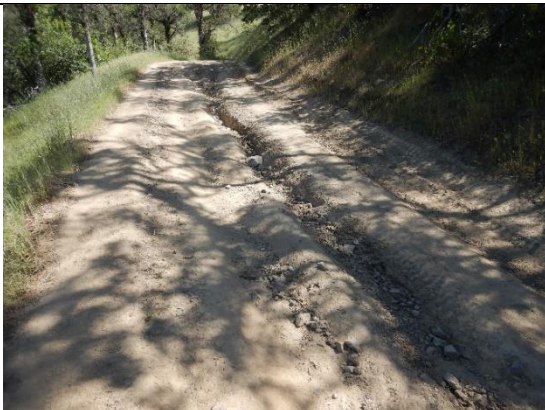
Photo 15 – Road erosion at WQ19
