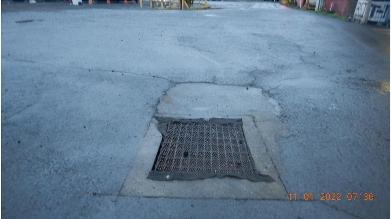
Picture 3 – View of Drop inlet that receives runoff from the metal bin storage areas shown on the previous pictures. Picture taken by Farzad Kasmaei.
