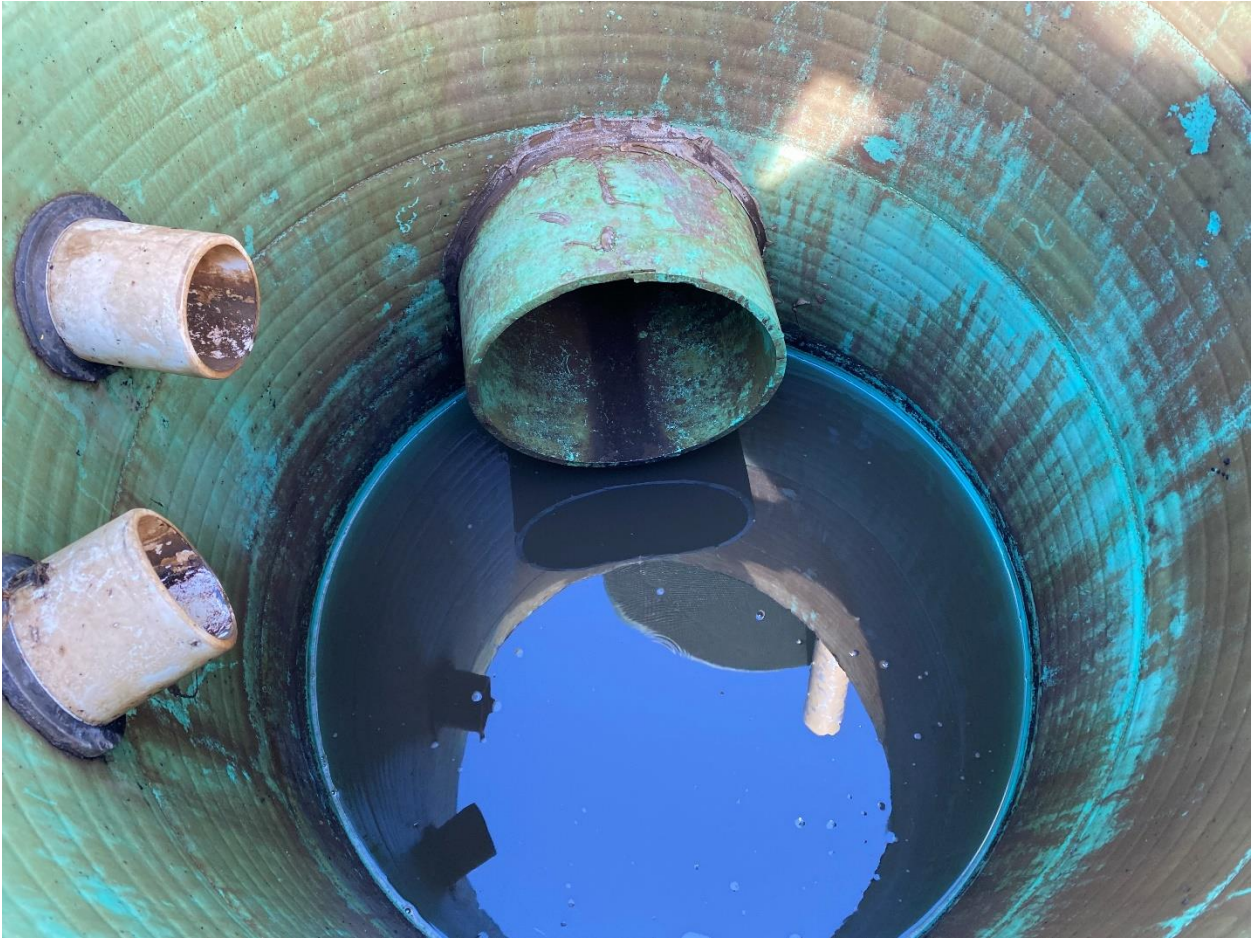
Picture 16: The two small pipes are where the auto-pumped water from the storage vault enters the outlet area. Post inspection picture taken by Facility's consultant (Greg Puccioni)
