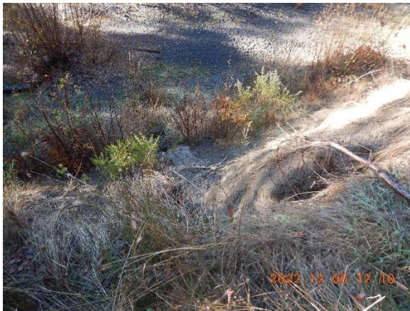
Figure 10. WQ2, slip-out and discharge into side-channel of Little Larabee Creek.
