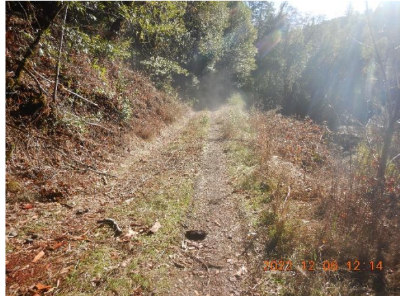
Figure 7. WQ2. North approach of access road with vertical unstable area on outboard edge of road.
