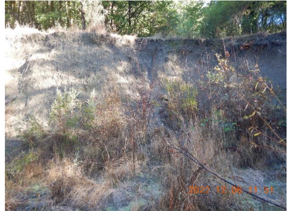
Figure 11. WQ2, vertical face has eroded road prism.
