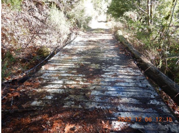
Figure 5. WQ1, Class II bridge was to be removed but is still in-place.
