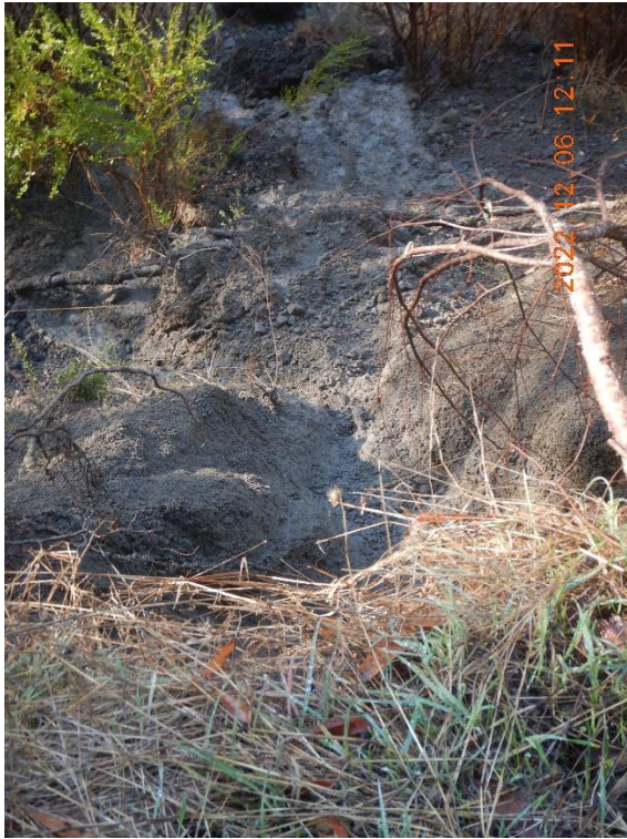
Figure 9. WQ2, slip-out and discharge into side-channel of Little Larabee Creek.
