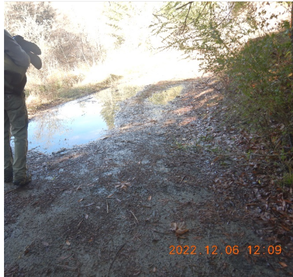
Figure 8. WQ2, puddled water on south approach of road above vertical unstable outboard slope.
