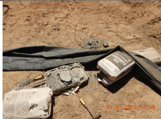
Photo 14- uncontained cement near WQ1
