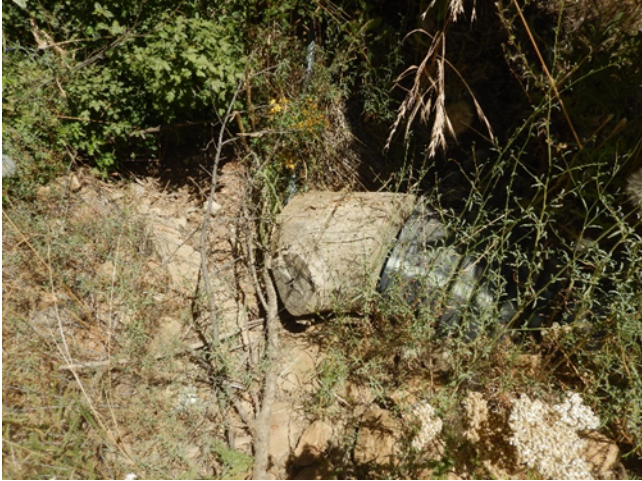
Photo 3: Culvert stream crossing with blocked inlet
