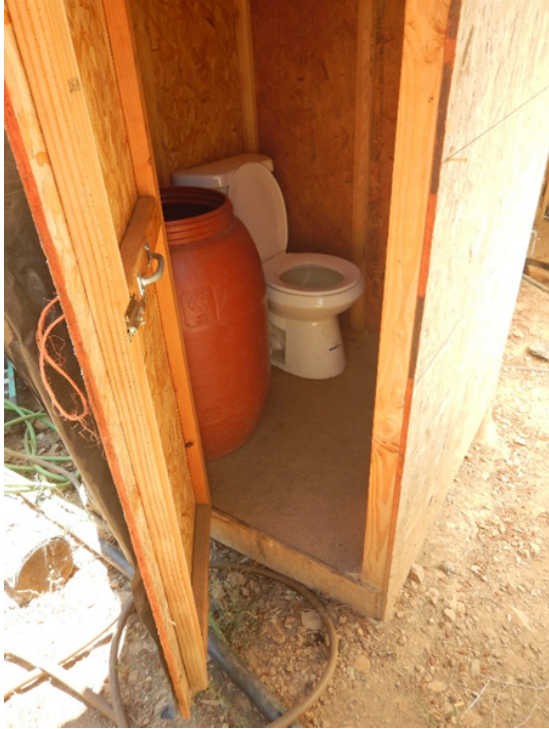
Photo 9: Outhouse with black pipe discharging human waste to land
