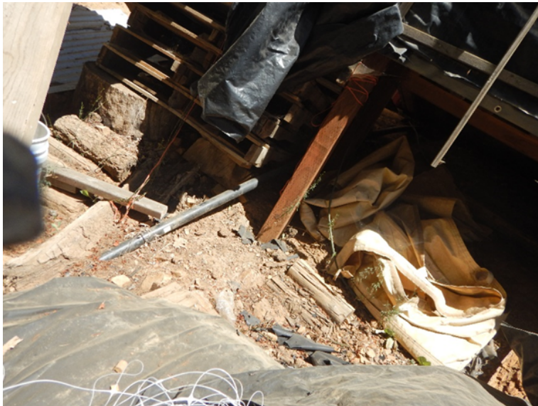
Photo 10: Outhouse with black pipe discharging human waste to land
