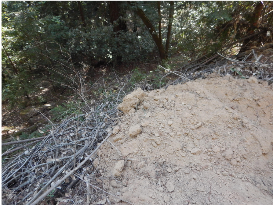
Photo Point 4.3 - Mineral soil lying on dead vegetation blocking outlet of waterbar.
