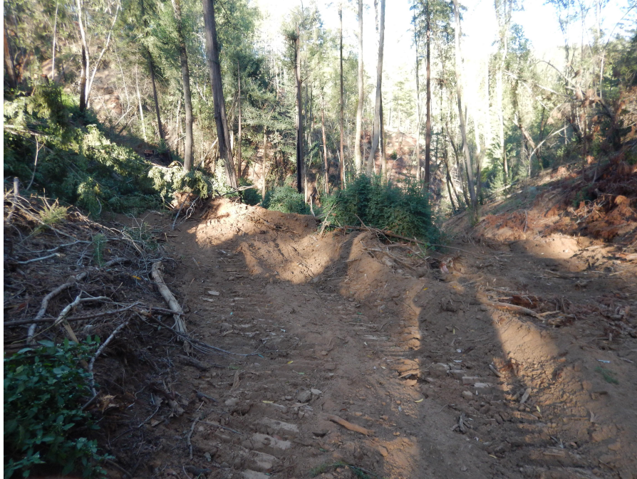
Photo Point 2.2 - Midway down skid trail, showing ineffective water bar.
