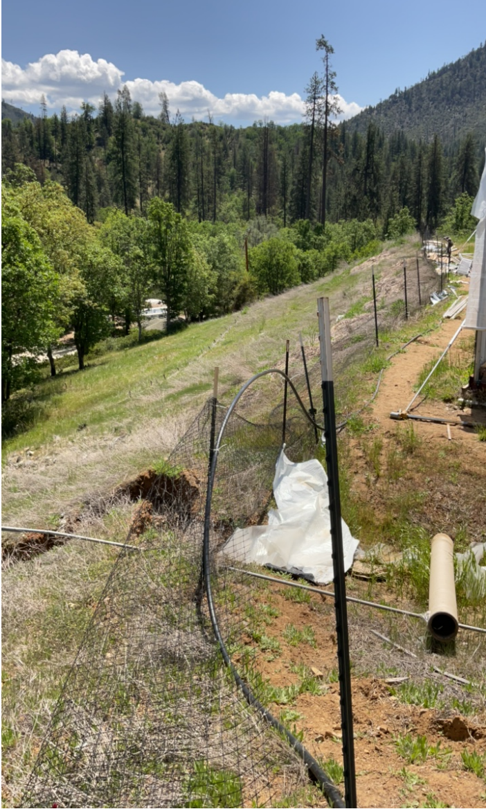
Photo 7: Eroded drainage channel on back edge of cultivation flat.
