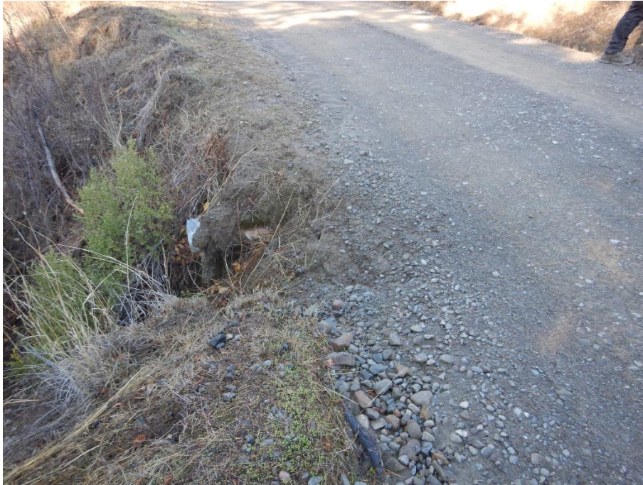
Photo 3—Looking west at culvert outlet located at WQ 3. The culvert is perched, and the channel has incised below the outlet.
