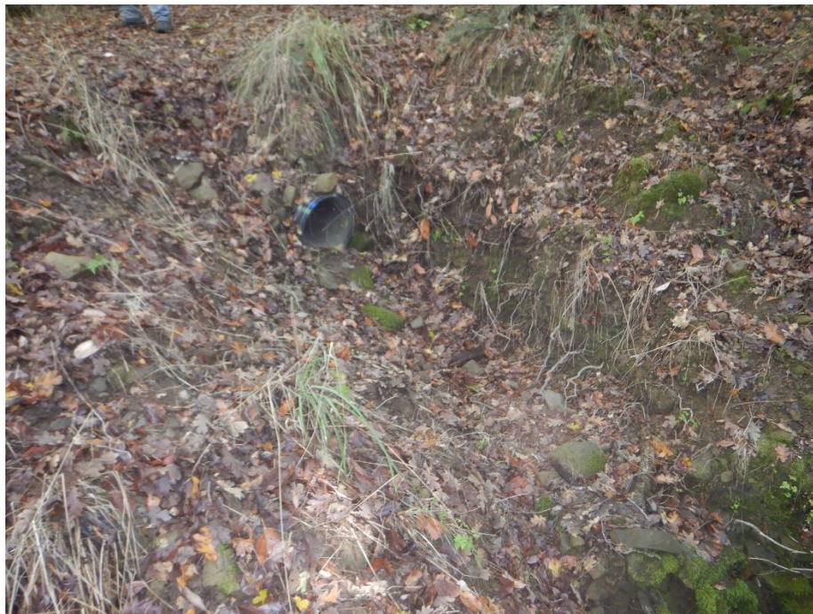
Photo 35—Looking north at culvert outlet in the vicinity of WQ 21. The culvert is aligned with the stream bottom.
