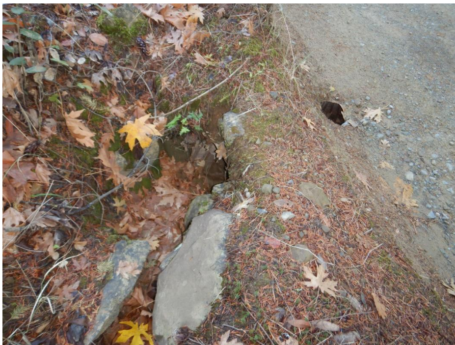
Photo 13—A hole in the road surface connecting to ditch relief culvert below the road located north of WQ 10.
