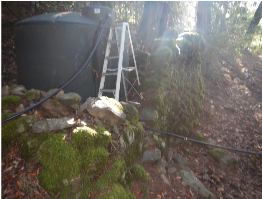
Photo 19—Tank collecting spring water at WQ 12.
