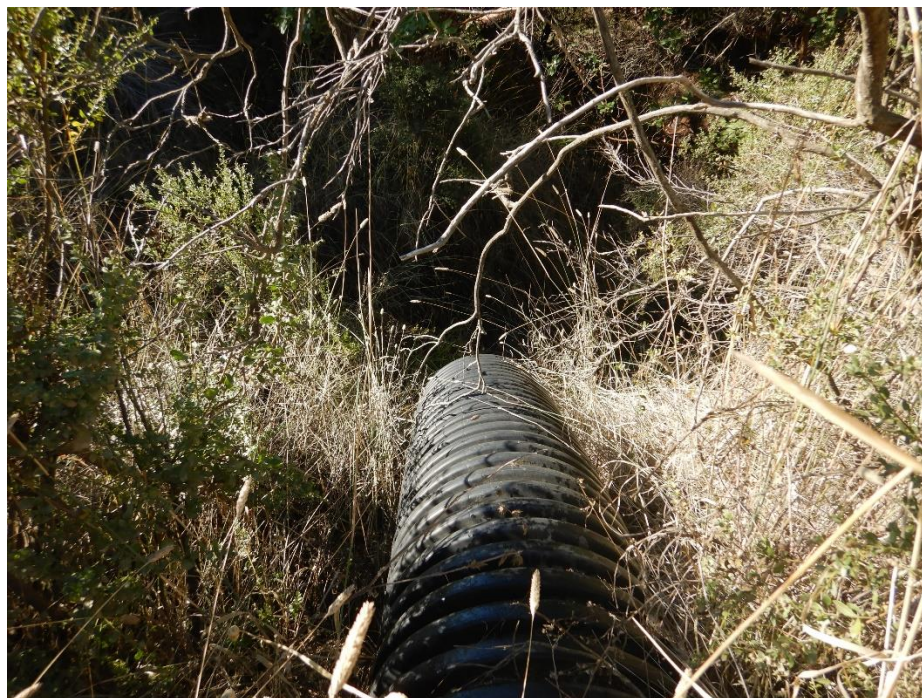
Photo 12 Looking west towards incising watercourse downstream from pipe at WQ 9.
