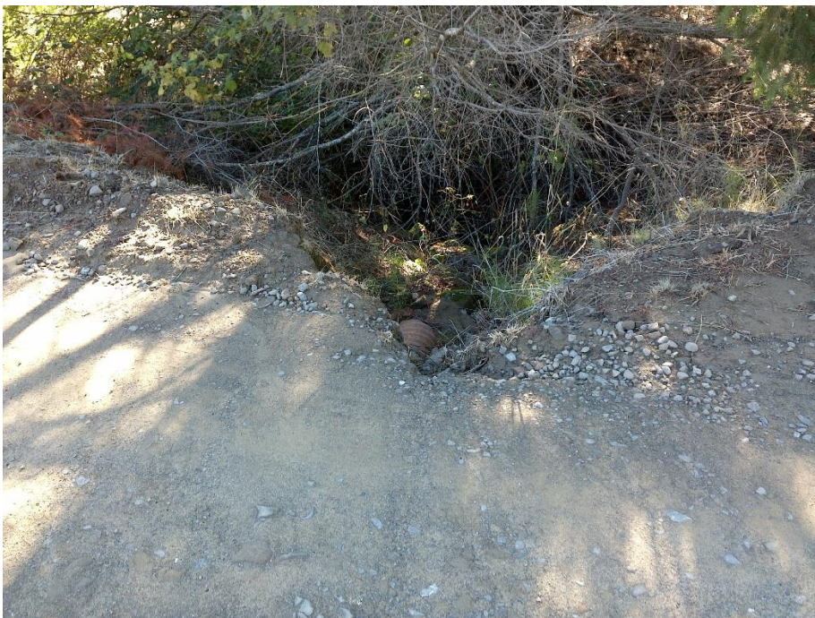
Photo 10—Looking south at culvert outlet at WQ 8. The road prism has failed above the culvert outlet.
