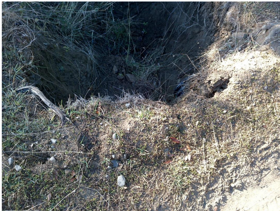
Photo 7—Looking south at culvert outlet at WQ 5. The top of the culvert is visible to the center-right of the image.
