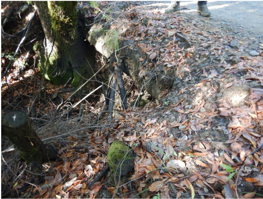
Photo 9—Looking west in the vicinity of the expected culvert outlet located at WQ 7.
