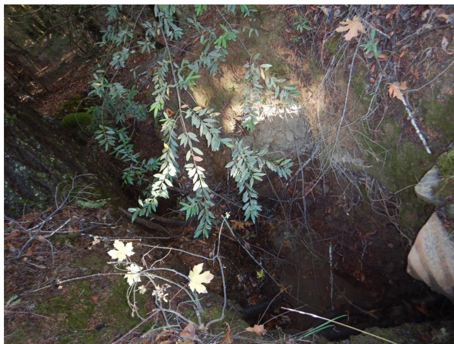
Photo 14—A 12inch diameter culvert perched above a scoured watercourse at WQ10.
