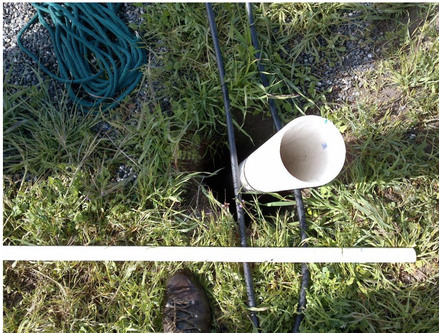
Figure 7—Looking down at a four-inch diameter plastic pipe in a twelve-inch diameter hole at WQ2. The well hole does not have a casing or cap to protect groundwater from any pollutants that could be introduced at the surface.
