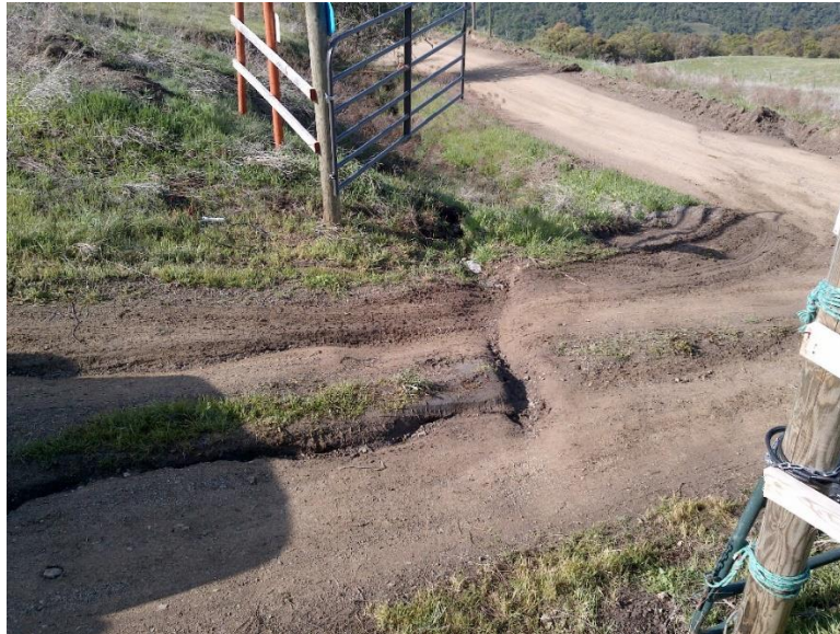
Figure 5—Looking southwest across the gated access to the Property at WQ1. Ruts have eroded into the road-surface.
