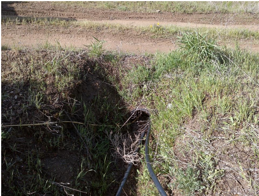
Figure 9—Looking southwest at a ten-inch diameter culverted watercourse crossing at WQ4. The watercourse upstream and to the back of the photographer is approximately three-feet wide.
