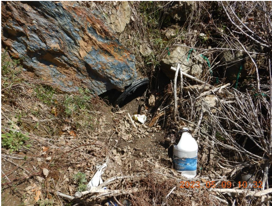
Figure 18—Partially buried culvert outlet at WQ6 among cultivation waste including plant stalks and plastic containers.
