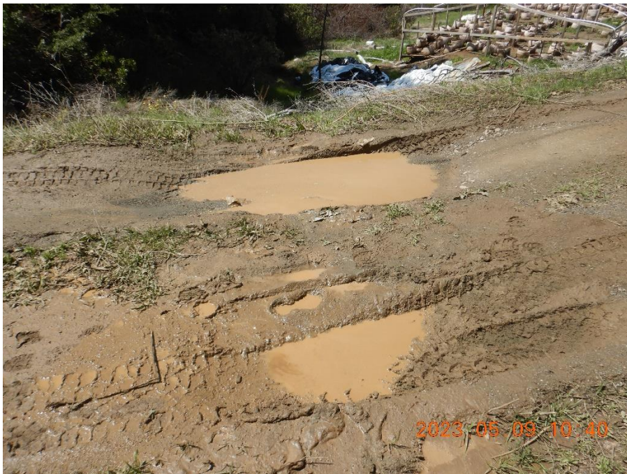
Figure 23—Water on top of the reservoir's impounding berm. The topography is shaped such that the stream channel approaching the reservoir from the northwest would bypass the reservoir and flow over the road at this location.
