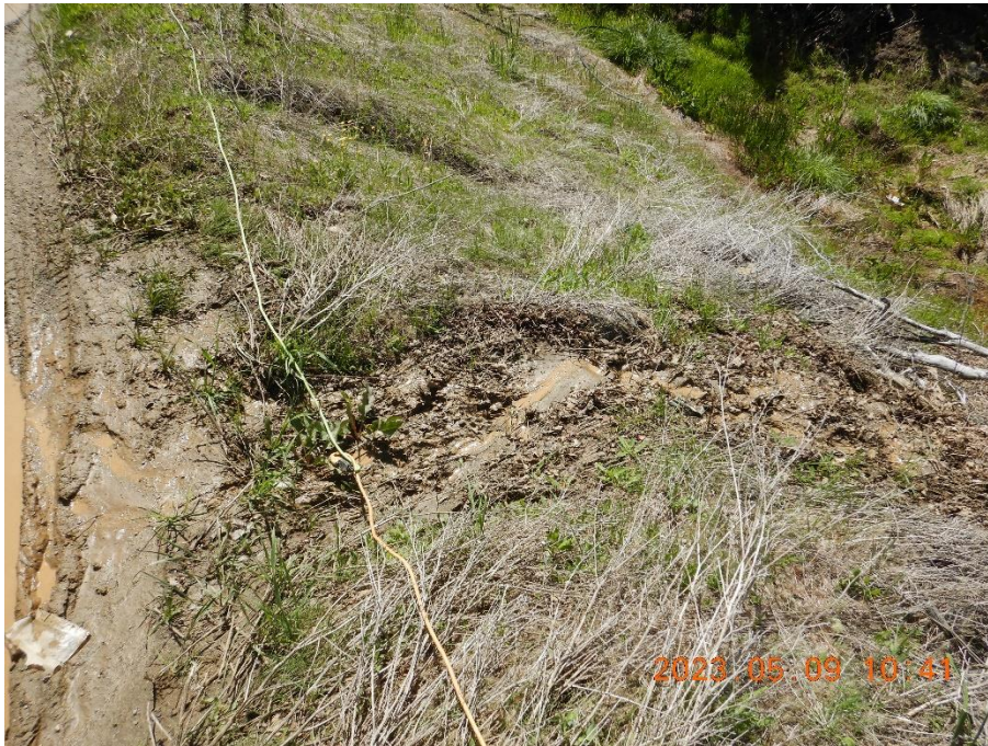
Figure 24—Sediment laden water from road surface pictured in previous image, flowing towards the USGS mapped blueline stream out of view to the right of the image.
