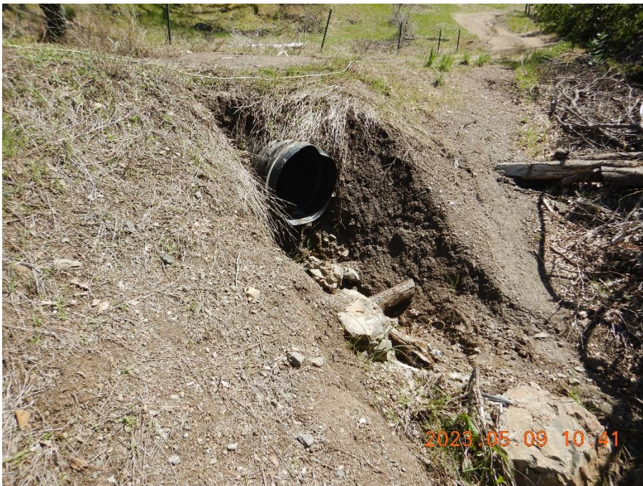
Figure 25—Reservoir outlet drain at WQ9 directed toward USGS mapped blueline stream out of view to the right of the image. The outlet pipe is 20-inches in diameter and lacks armor which has resulted in erosion and downstream transport of the earthen fill.
