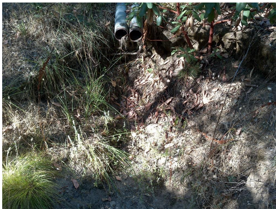
Figure 11—Photo looking at the drainpipe outlets located WQ3. A void has formed in the unarmored buttress at the discharge location.
