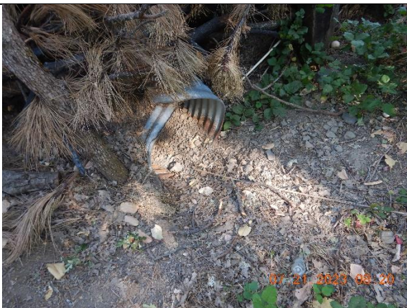
Photo 11 – A partially rusted and clogged outlet of a culverted watercourse crossing at WQ10
