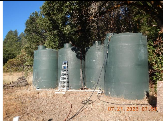
Photo 14- Water storage tanks at WQ6 and nearby what appears an inactive Groundwater well on the left bottom corner of the photo
