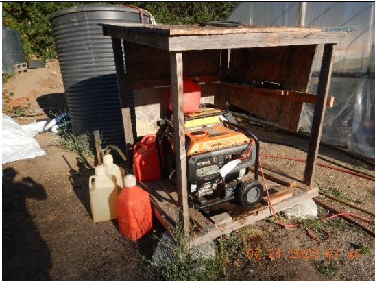
Photo 15 – water storage tank and an improperly contained generator and gasoline at WQ3
