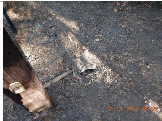
Photo 10 – completely buried and clogged inlet of a culverted watercourse crossing at WQ10
