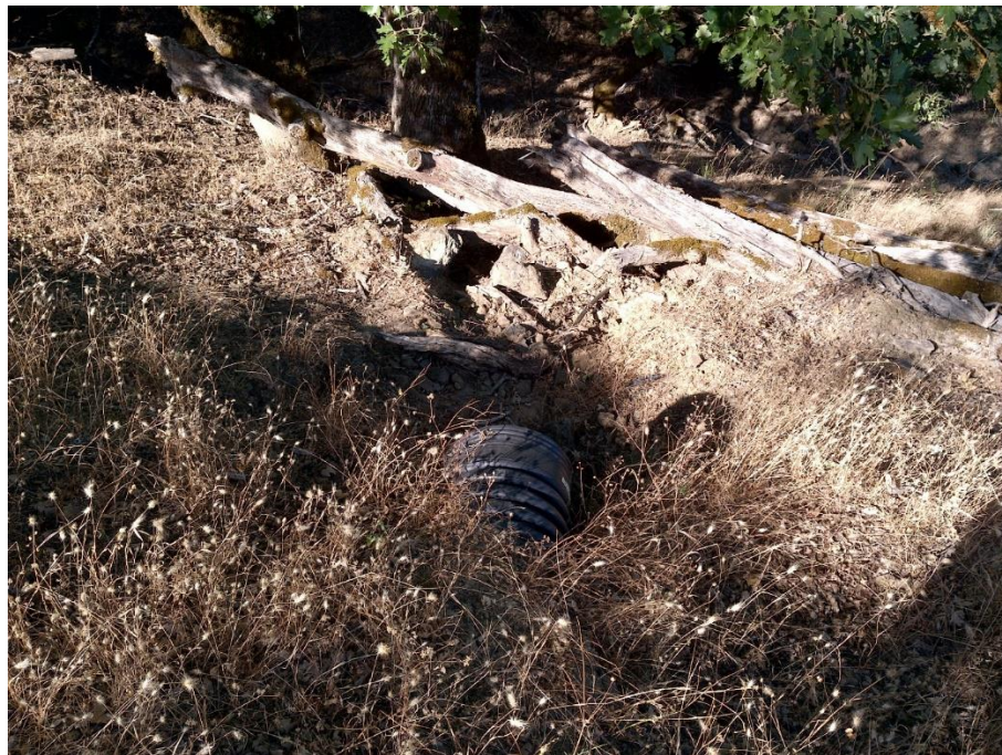
Figure 13—Photo looking west at pond outlet at WQ7. The Pipe drains onto a pile of woody debris.
