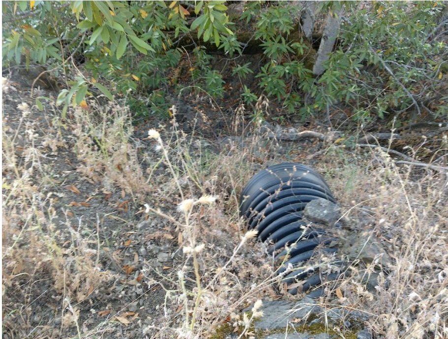
Figure 6—Photo showing the outlet of the 18-inch diameter culvert at WQ3, the inlet of which is pictured in the previous image. A receiving watercourse, tributary to Feliz Creek, is visible in the top of the image.
