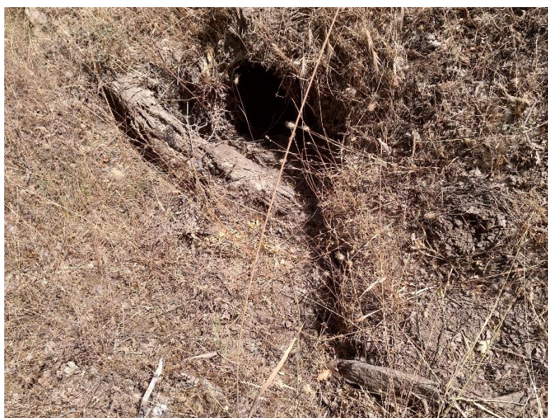
Figure 3—Photo showing inlet to 18-inch diameter culvert at WQ2. The inlet is partially blocked by woody debris and dry vegetation.
