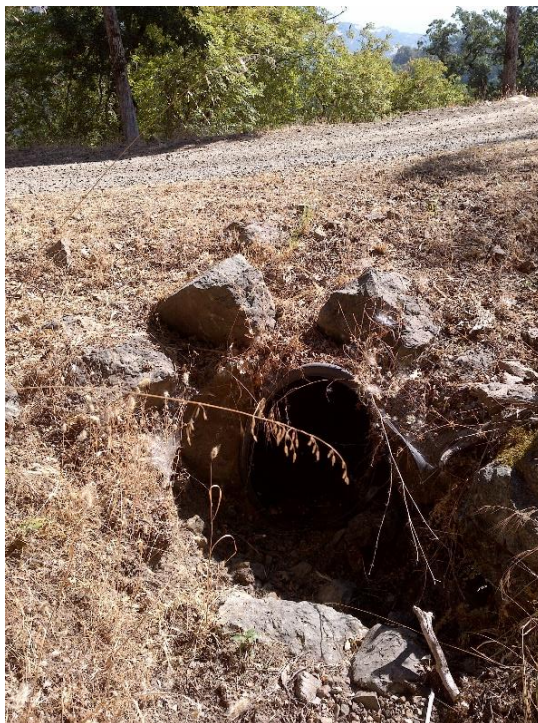
Figure 2—Photo showing the inlet to a 24-inch diameter culverted stream crossing at WQ1.
