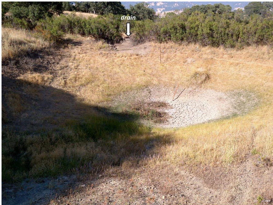
Figure 10—Looking east across reservoir from WQ4. The reservoir drain is visible at the top of the image. The reservoir’s outboard face is densely vegetated with woody brush.
