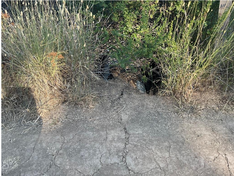
Figure 9—Photo looking at the reservoir’s outlet, located at WQ3, from the road passing over the reservoir’s berm. The outlet pipe is shallowly buried and there are voids in the dam berm surrounding the outlet pipe.
