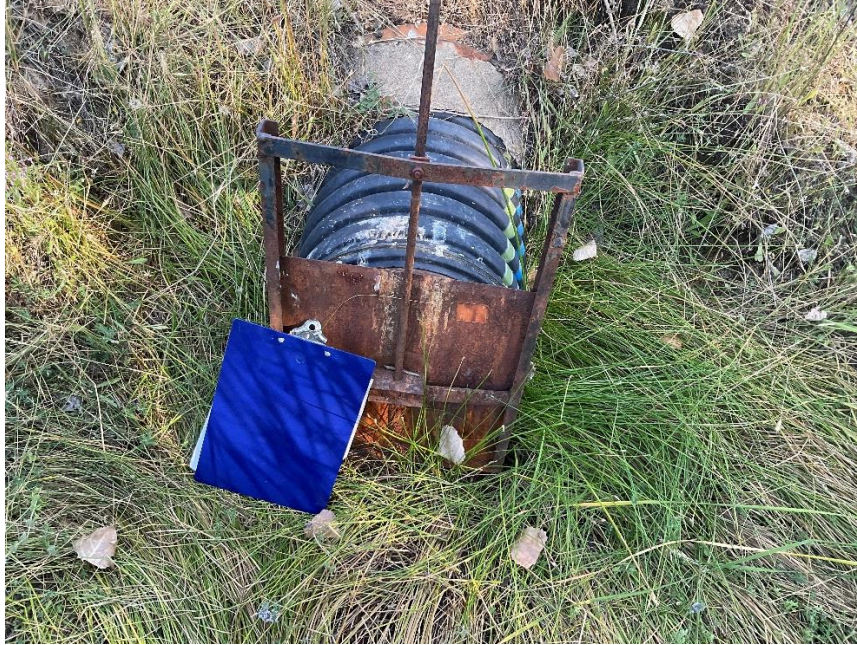
Figure 11—Looking at the inlet for the reservoir drain at WQ5 from within the reservoir’s berm. The drainpipe is eighteen inches in diameter and the top of the drainpipe is approximately eighteen inches below the dam crest. The drainpipe is blocked by a rusted gate valve.
