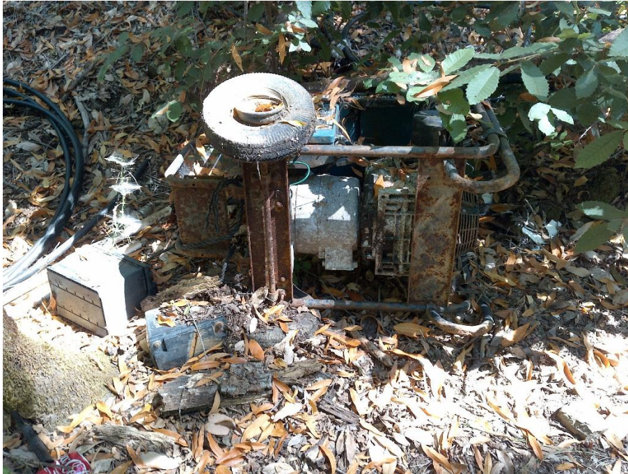
Figure 18—Photo showing a petroleum powered generator and two lead-acid batteries in the vicinity of WQ8. The generator is tilted on its side and does not have a drip pan nor other form of secondary containment to protect against the discharge of petroleum products to land.
