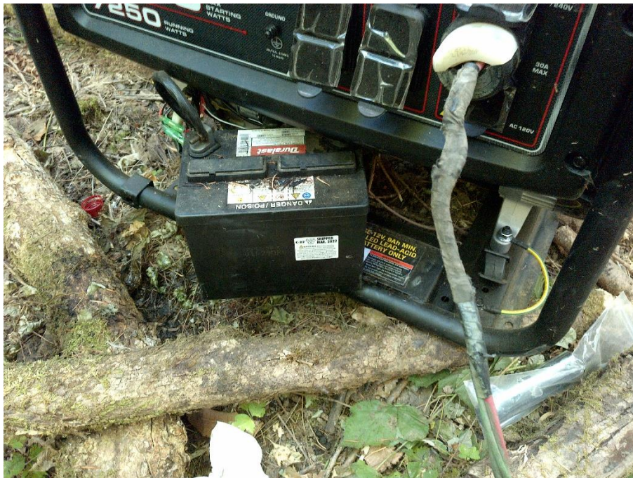
Figure 9—Photo showing a petroleum powered generator and lead-acid battery in the vicinity of WQ6. The generator does not have a drip pan nor other form of secondary containment to protect against the discharge of petroleum products to land.
