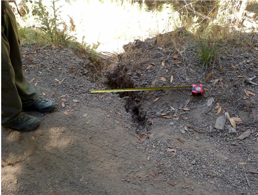
Figure 4—Photo showing a rill scoured into the edge of a road east of WQ2.
