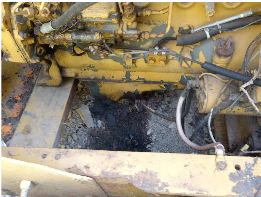
Figure 7—Photo showing spilled motor oil below a piece of heavy equipment at WQ5. The equipment does not have a drip pan nor other form of secondary containment and the oil has spilled onto the permeable earthen land.
