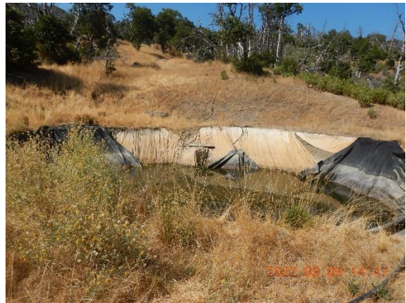
Figure 11. Pond1 is located at WP 940 (40.372367°, -123.449754°) and has over steepened interior slopes, has no outlet, tarps are falling into the excavation.
