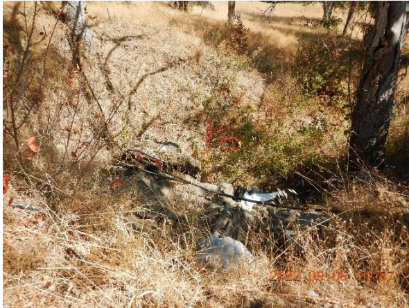
Figure 13. Culvert inlet at Crossing X1 at WP 921 (40.371095°, -123.449291°) is a culvert with road runoff delivery.
