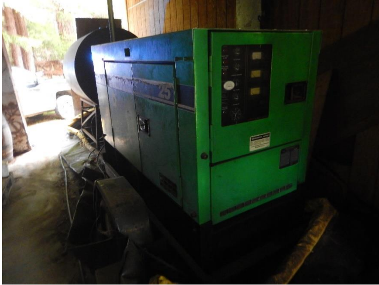
Photo 5: Generator stored on concrete floor under permanent roof with secondary containment.
