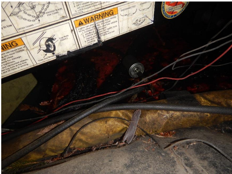
Photo 6: Diesel fuel beneath generator captured by secondary containment.
