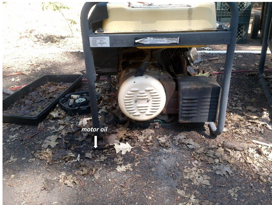
Figure 7—Photo looking at a petroleum-fueled generator located at WQ1. The generator does not have secondary containment. The permeable earthen ground below the generator is dark where motor oil has discharged to land.
