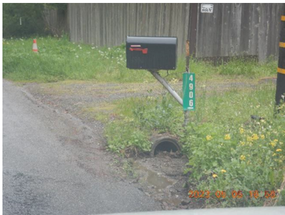
Figure 30. The ditch goes under the next driveway associated with 4906 Greenwood Heights (APN 404-061- 004).
