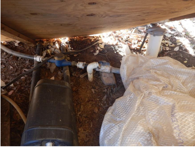
Photo 8: Groundwater well under wooden boards.
