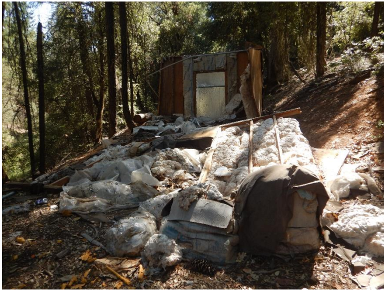
Photo 4: Structure with insulation pulled out.
