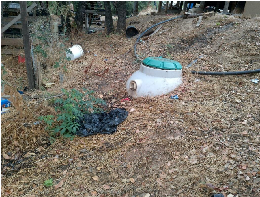
Figure 8—Photo of sewage tank at WQ2. Sewage pipes from the structure in background of image flow into tank. A pipe exiting the tank is open and human waste is visible on the pipe and on the ground next to the tank.
