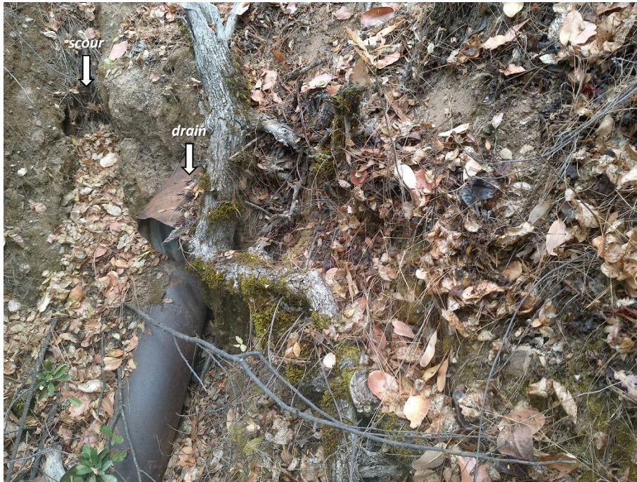
Figure 18—Photo looking upstream from the left bank at the culvert outlet at WQ7. The picture shows the same drain and scour marks as in the other image but from a different angle.
