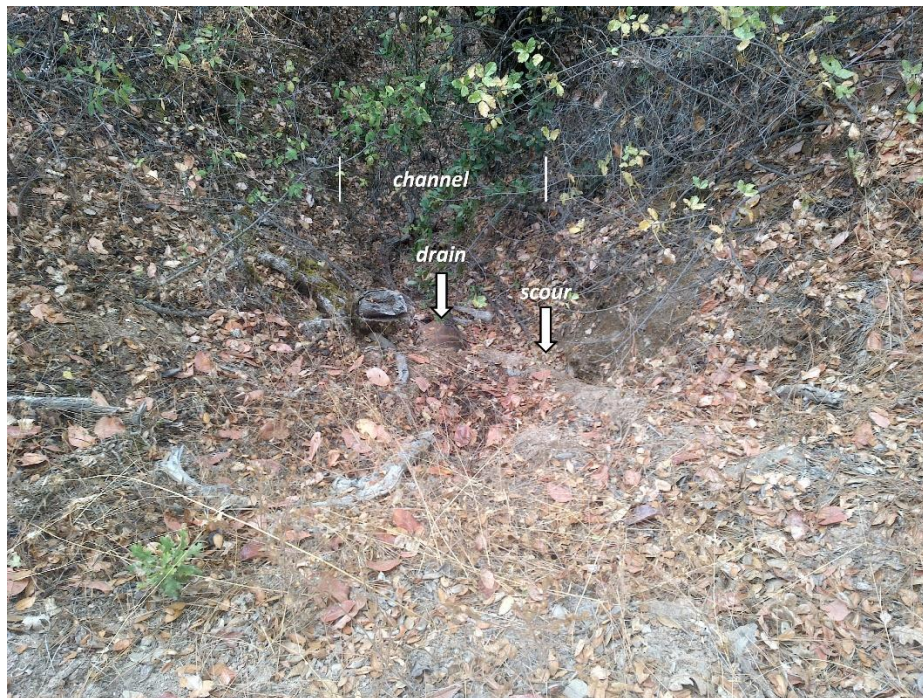
Figure 17—Photo looking downstream at a watercourse crossing located at WQ7. A rusted 12-inch diameter corrugated metal pipe is identified as the drain in the middle of the image. The pipe is significantly narrower than the channel downstream and scour marks are visible on the road prism above the pipe.
