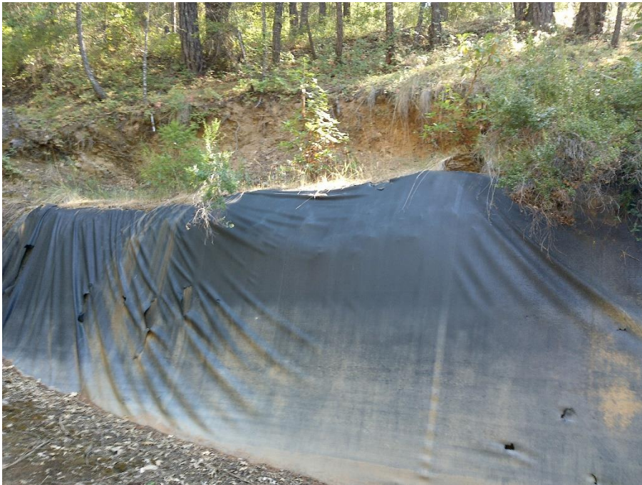
Figure 7—Photo looking at the west bank of the reservoir located at WQ1. The reservoir wall appears to be excavated into a hillslope and is nearly vertical.
