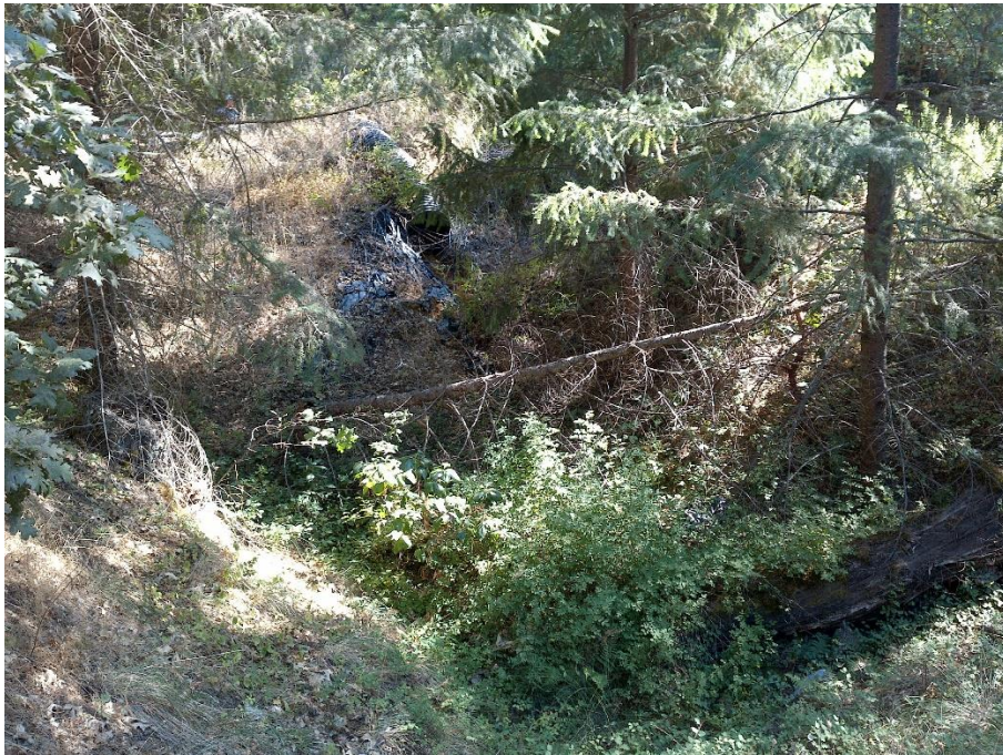
Figure 9—Photo looking south at reservoir outlet at WQ1. The outlet pipe discharges onto the earthen dam embankment.
