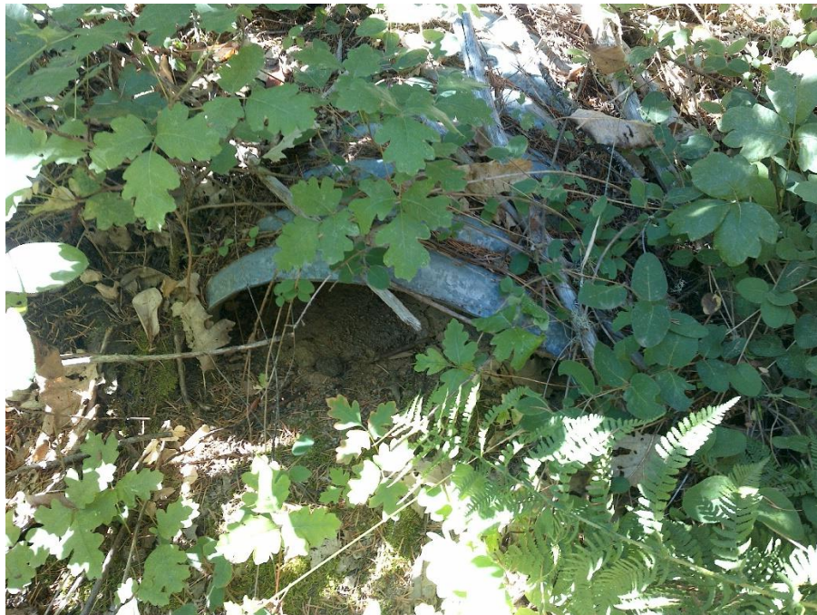
Figure 11—Photo looking south and upstream at a corrugate metal pipe outlet. Sediment has deposited in the bottom of the pipe decreasing its capacity for transporting water by approximately 80 percent.
