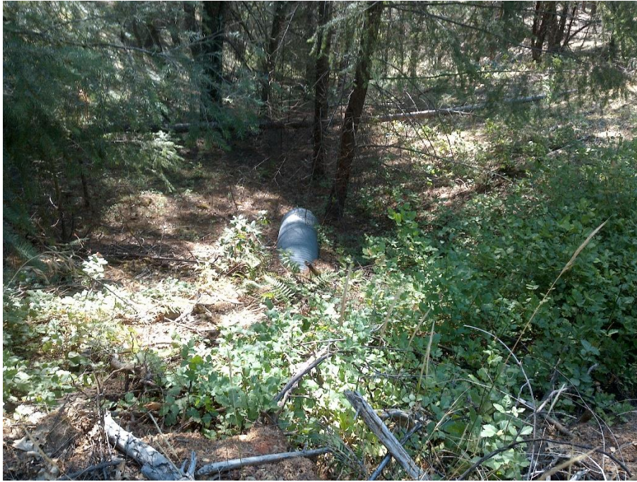
Figure 14—Photo looking west and down gradient at a corrugated metal pipe located at WQ4. The presence of vegetation and the accrual of overlying leaf litter suggests that the culvert was installed years earlier.
