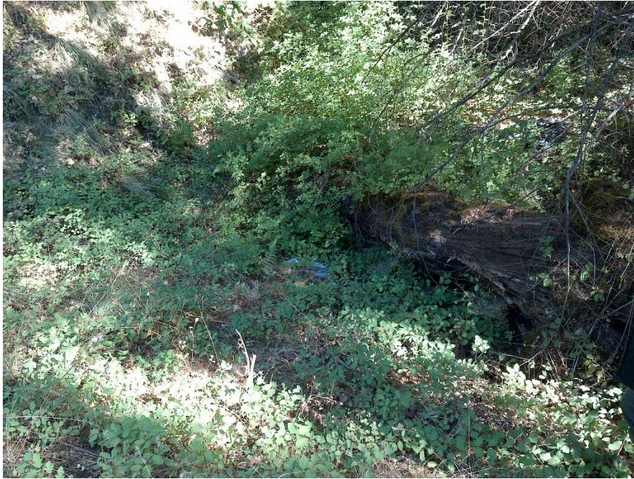
Figure 10— Photo looking south and upstream at a corrugated metal pipe inlet visible in the middle of the image. The reservoir outlet, pictured in the previous figure, is out of view in the back right of this image. The culvert inlet is blocked by a fallen tree.
