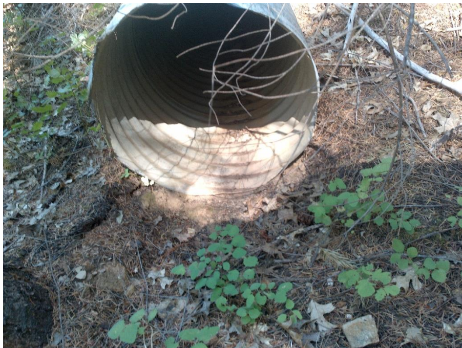
Figure 15—Photo looking up-gradient at the outlet of a 24-inch diameter corrugated metal pipe at WQ4. The pipe discharges onto the forest floor and there is no sign of erosion or channel formation suggesting the culvert is only subjected to relatively small flowrates.
