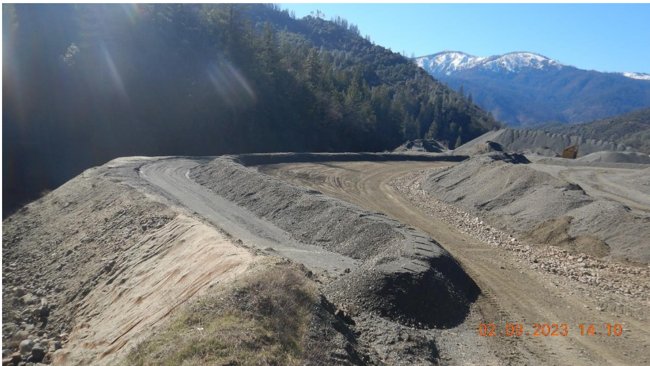
Picture 7 – Looking west at stabilized area adjacent to Oregon Gulch. This area has been recently improved in accordance with emergency CAO. The newly constructed access road, installed berm and netting are shown on the picture. Picture taken by Farzad Kasmaei.
