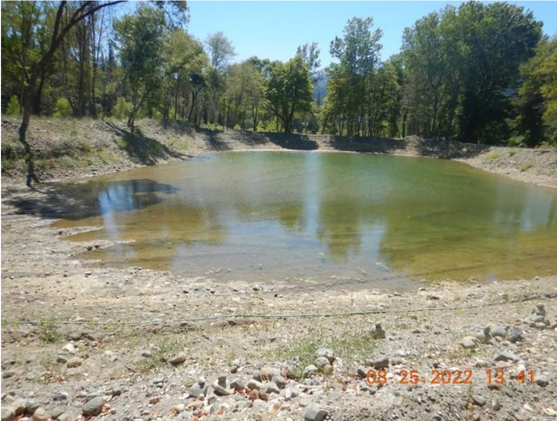
Photo 15a: Pond installed off channel, filled with water piped from Oregon Gulch.
