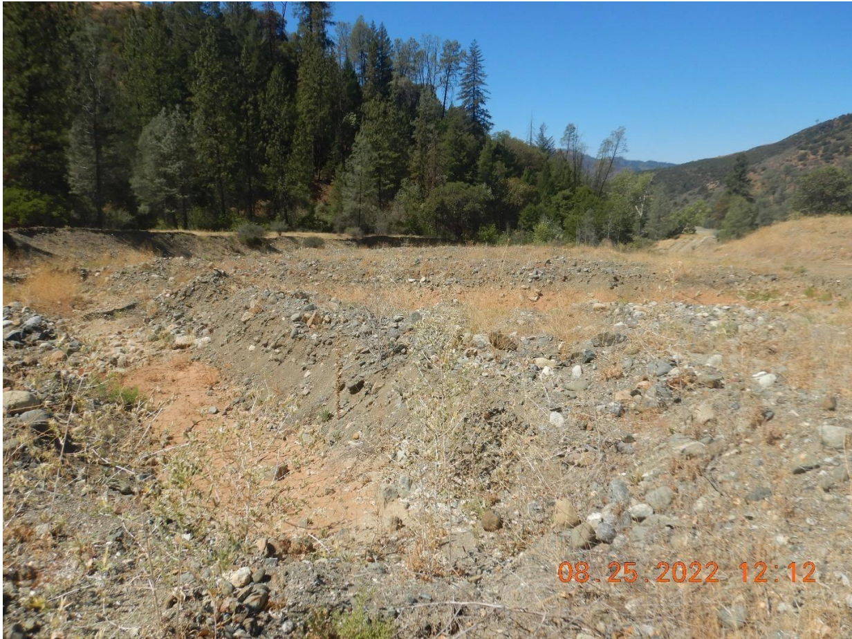
Photo 9: View of the installed wide berms in Oregon Gulch. Picture taken by Amanda Piscitelli.
