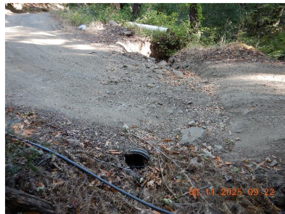
Photo 8 Partially blocked culverted watercourse crossing outlet and eroded road fill prism at WQ2
