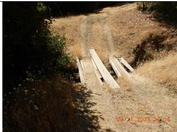
Photo 21 Wooden bridge with sediment discharge and threatening failure at WQ23
