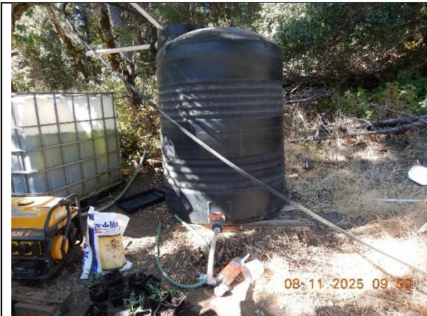
Photo 37 Showing water storage tanks, fertilizer, and a generator without secondary containment near WQ7
