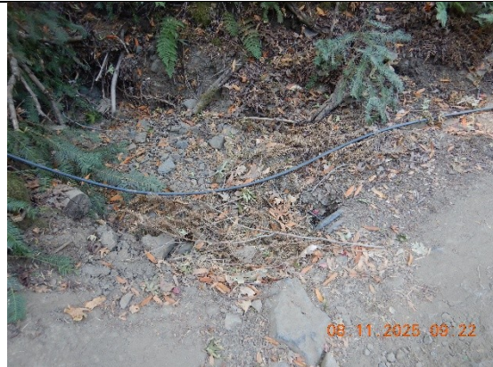
Photo 7 Partially blocked culverted watercourse crossing inlet at WQ2
