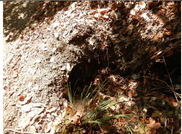
Photo 20 Concrete culverted watercourse crossing inlet at WQ17, partially blocked and without rock protection
