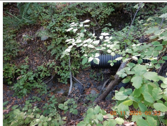
Photo 10 Shot-gunned outlet of a double culverted watercourse crossing at WQ2
