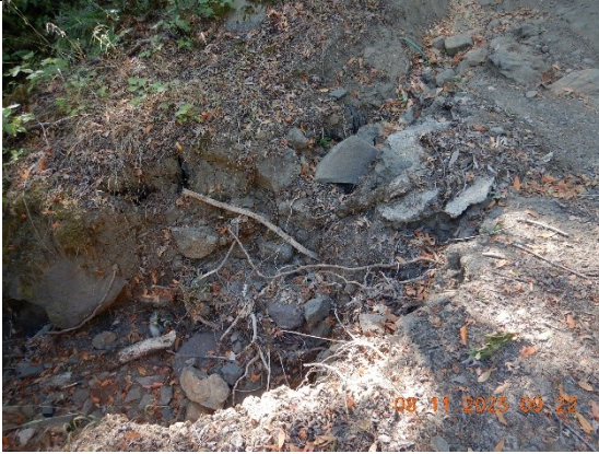
Photo 9 Eroded road fill prism at the outlet of the watercourse crossing at WQ2
