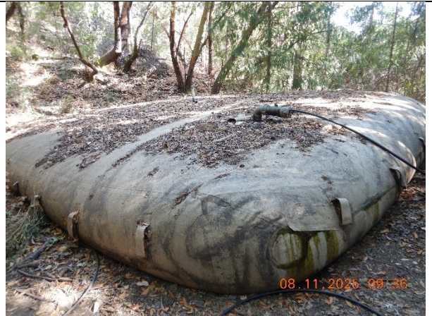
Photo 34 Water storage bladder without secondary containment and within riparian setback at WQ4
