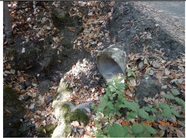
Photo 12 Concrete culverted watercourse crossing outlet at WQ3, installed slightly high in the fill
