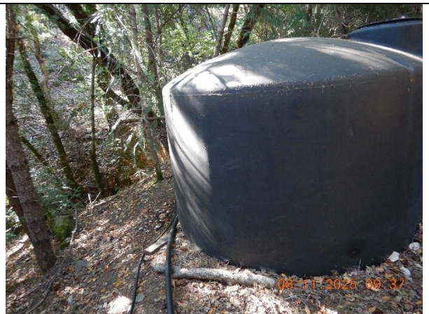
Photo 36 Showing water storage tanks and the nearby watercourse in the vicinity of WQ5
