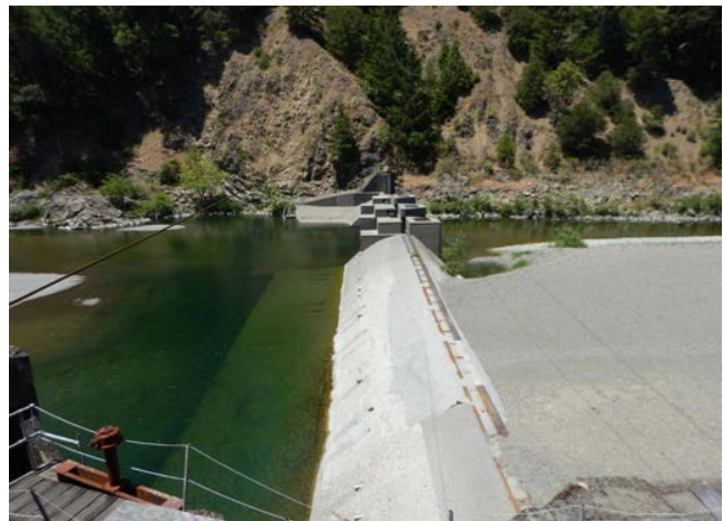
A view of the dam looking north towards fish passage columns and right bank fishway; upstream is to the right. Photo by Brendan Thompson.
