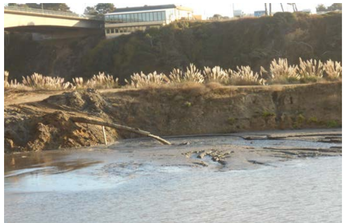
Water placement of dredge material. Photo by Erik Nielson, SHN Engineers & Geologists
