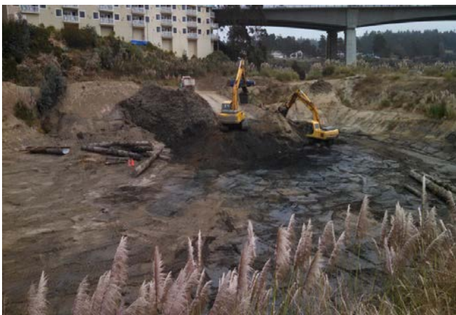
Upland dredge piles. Photo by Photo by Erik Nielson, SHN Engineers & Geologists.
