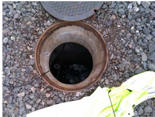
Manhole where the equipment is mounted
