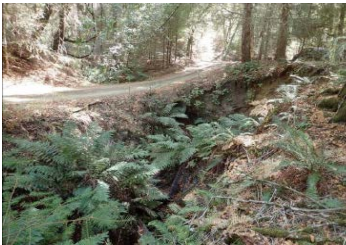
Pre-construction photo of a road crossing that blocks salmonid passage in the Navarro River Watershed. September 2, 2015. Photo by Rebecca Fitzgerald, NCRWQCB
