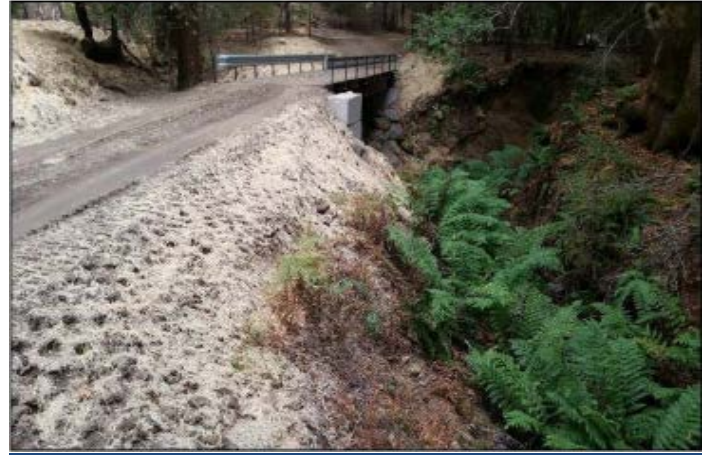
Post-construction photo of the same road with a new bridge and open salmonid passage. September 30, 2015. Photo by Rebecca Fitzgerald, NCRWQCB
