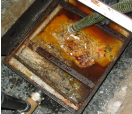
Commercial Grease Trap
