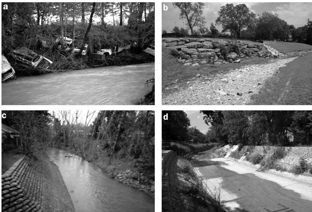
Figure 2. Examples of channel bank structures. Some bank erosion-control structures are not designed or engineered; rather, they are ad hoc attempts to prevent local land loss or damage. (a) Car bodies; (b) riprap; (c) sacrete on left bank, riprap on right bank; and (d) rock-filled gabions along banks of concrete-lined channel. Photographs: Joan L. Florsheim (2a and 2c) and Anne Chin (2b and 2d).
