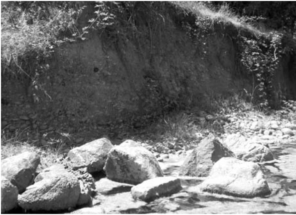
Figure 4. Bank erosion processes continuing behind large rock riprap originally placed at the base of the bank. If left isolated in the channel, riprap may become an impediment to future restoration. Photograph: Joan L. Florsheim.
