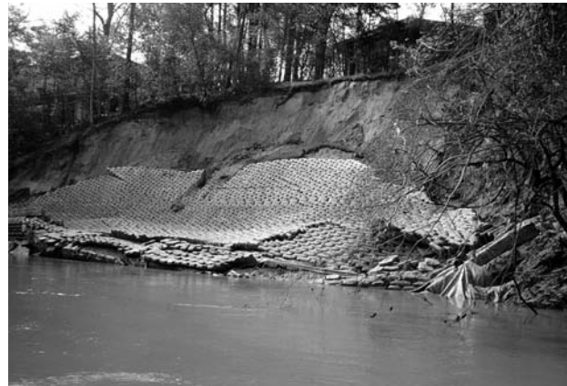
Figure 3. Failure of sacrete bank erosion control structure because of high pore-water pressure in the bank behind the structure. Photograph: Joan L. Florsheim.
