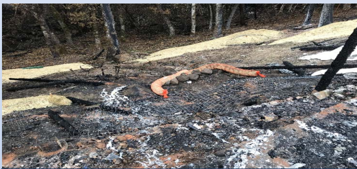
Figure 2. BMP controls installed downslope of a burned structure.
