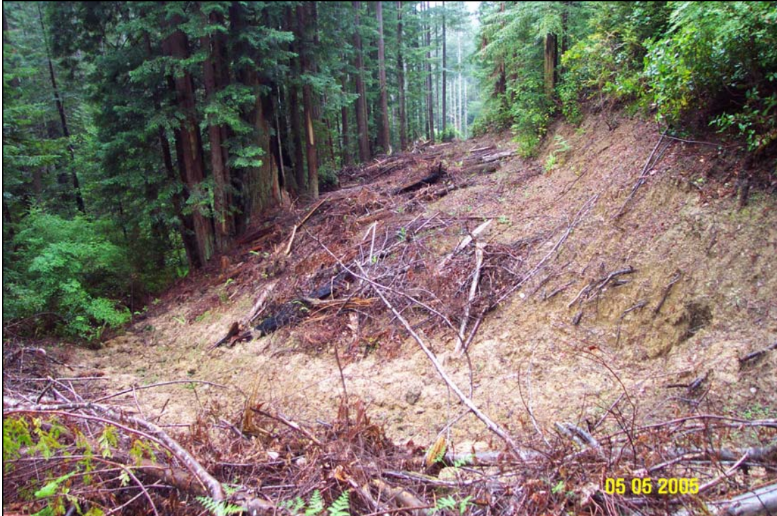
Photo 2. U06.6966 Spur 1 Road, Site #19, stream crossing, post-treatment almost one year later. The view is similar to the above photo, except taken from closer to what used to be the inboard edge of the road. Straw mulch was placed on the excavated side slopes near the channel bottom and slash placed on disturbed road surfaces to protect them from rainsplash.
