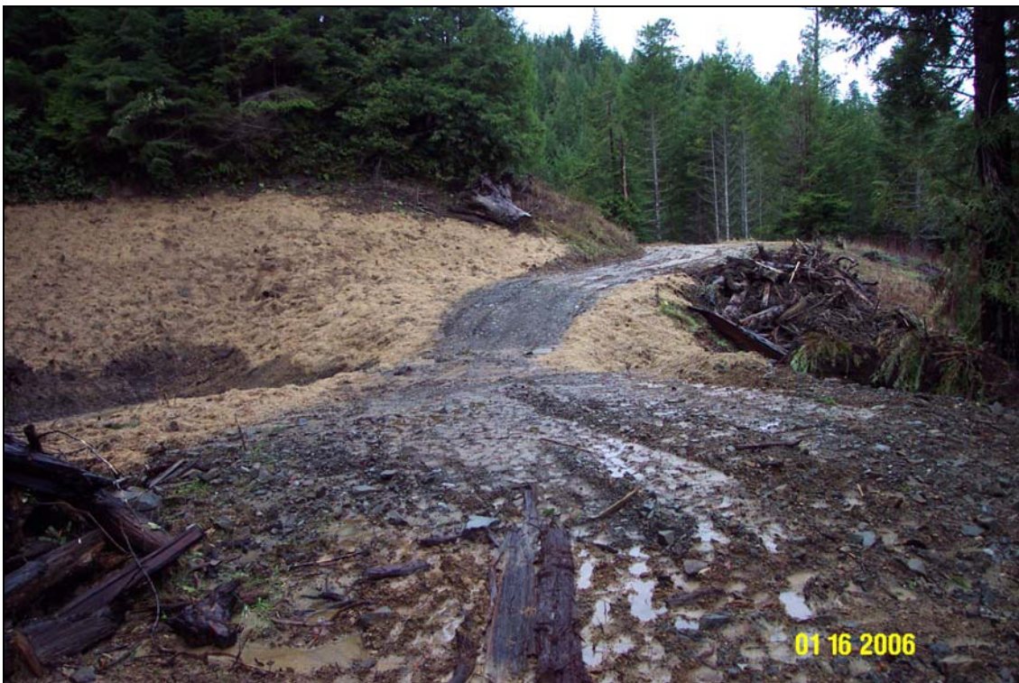
Photos 2A and 2B. R8 Road, site #121.1, a stream crossing, pre- and post-treatment. The picture was taken from the right road approach looking across the crossing. A culvert was installed at this site to pass flow for the winter. This was the last site treated on this road, before the onset of wet weather conditions closed down heavy equipment operations. Most of the work on this site took place above the road.
