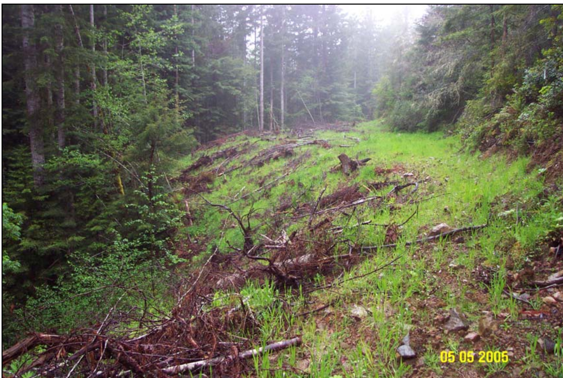
Photo #18B. Site #7, almost one year after treatment. View is similar to the above photo. The edge of the road was pulled back and some of the material was stockpiled upon the cutbank to create a complete outslope.
