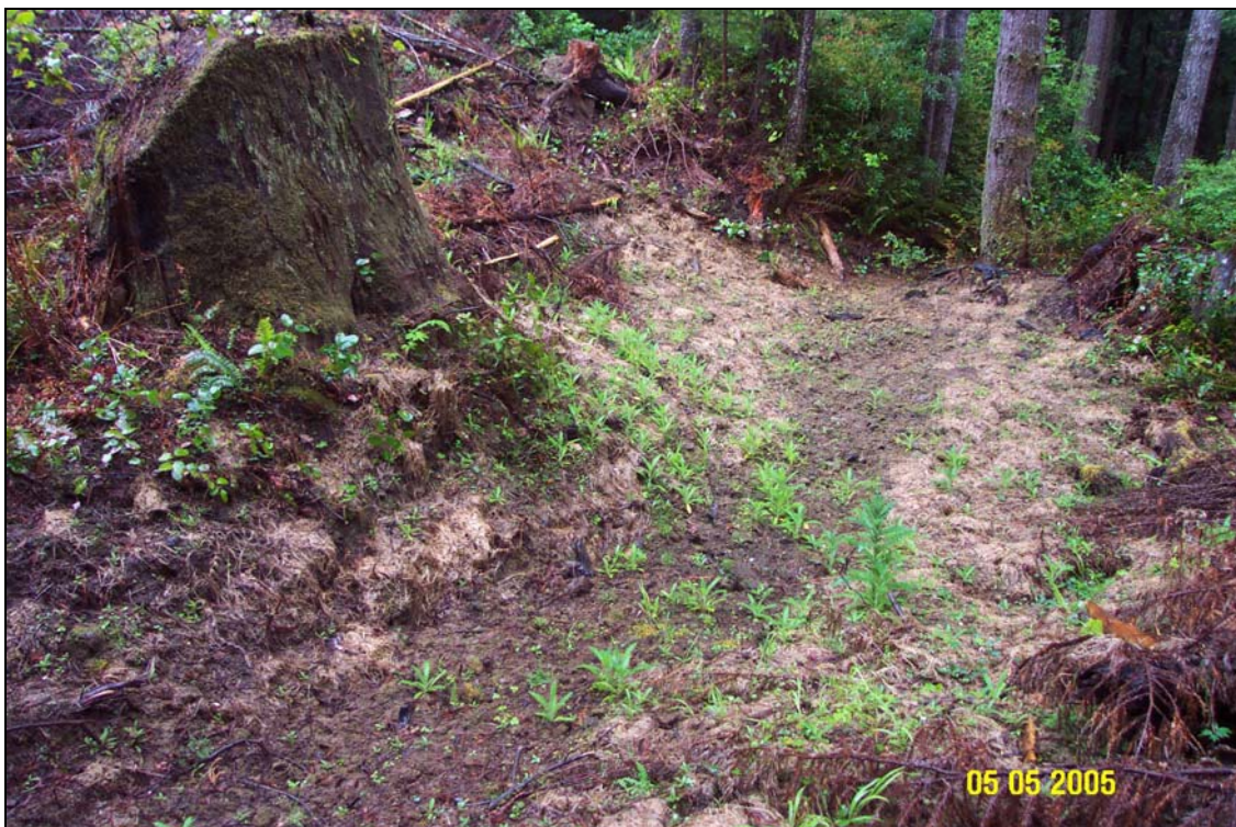
Photos 8A and 8B. U06.6966 Spur 1 Road, Site #16, stream crossing, pre- and post-treatment. The picture was taken from approximately the top, looking downstream. The bottom photo was taken after the site had gone through its first winter post-excavation.
