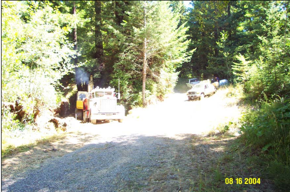
Photo 1. U06 Road, Site #1129, stream crossing, during its upgrade. The picture was taken from the left road approach looking across the crossing toward the right road approach. The excavator is removing fill from the stream valley upstream of the inlet and loading the spoils into dump trucks to be endhauled to a stable spoil disposal area nearby.
