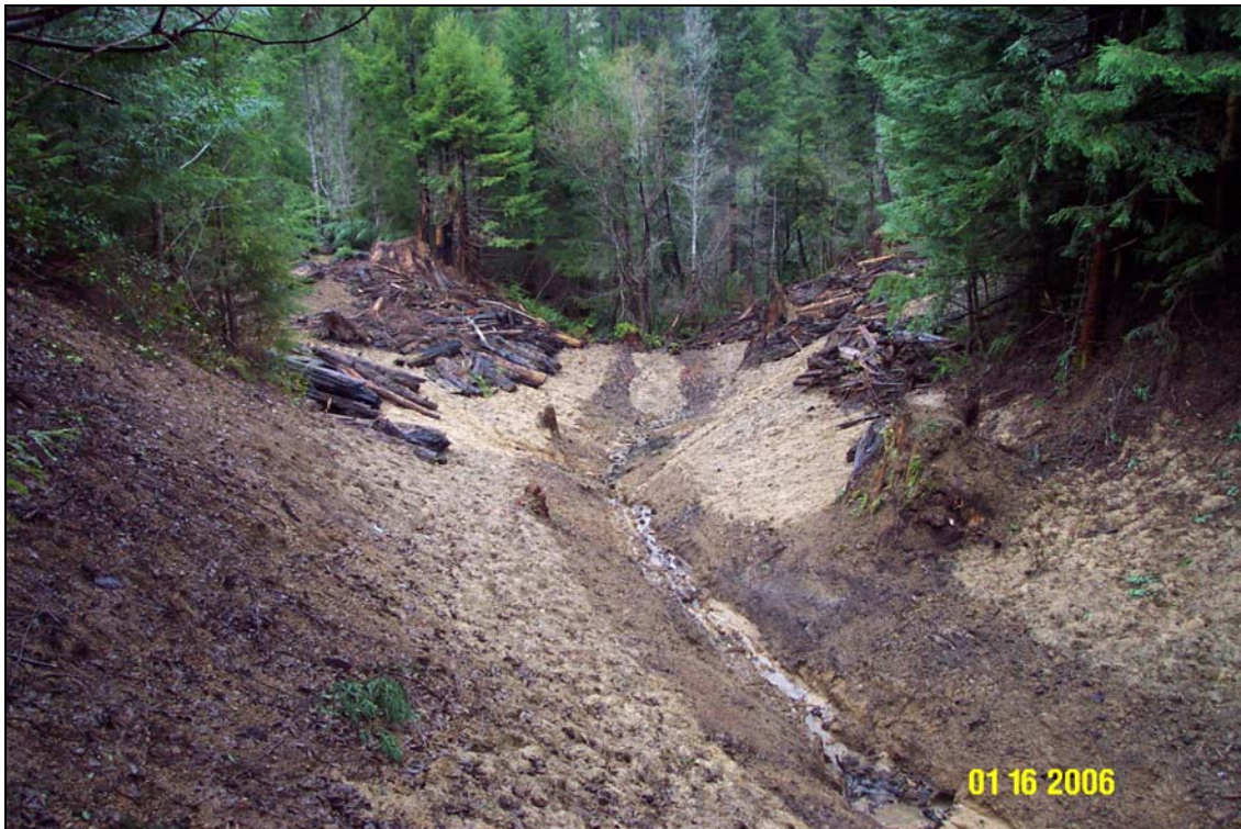
Photo 7A and 7B. R8 Road, site #121.1, during- and post-treatment. The view is from near the top of the excavation looking down to the road.
