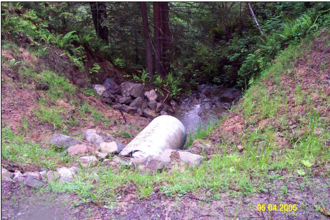
Photo 7. Site #1129, stream crossing, post-treatment. The picture was taken from the outboard edge of the road at the crossing looking downstream toward the outlet. Note how the culvert outlet extends beyond the base of the fillslope to reduce the potential for any material that might slough off the fillslope to come to a rest before reaching the stream. The outlet discharges flow onto bedrock.
