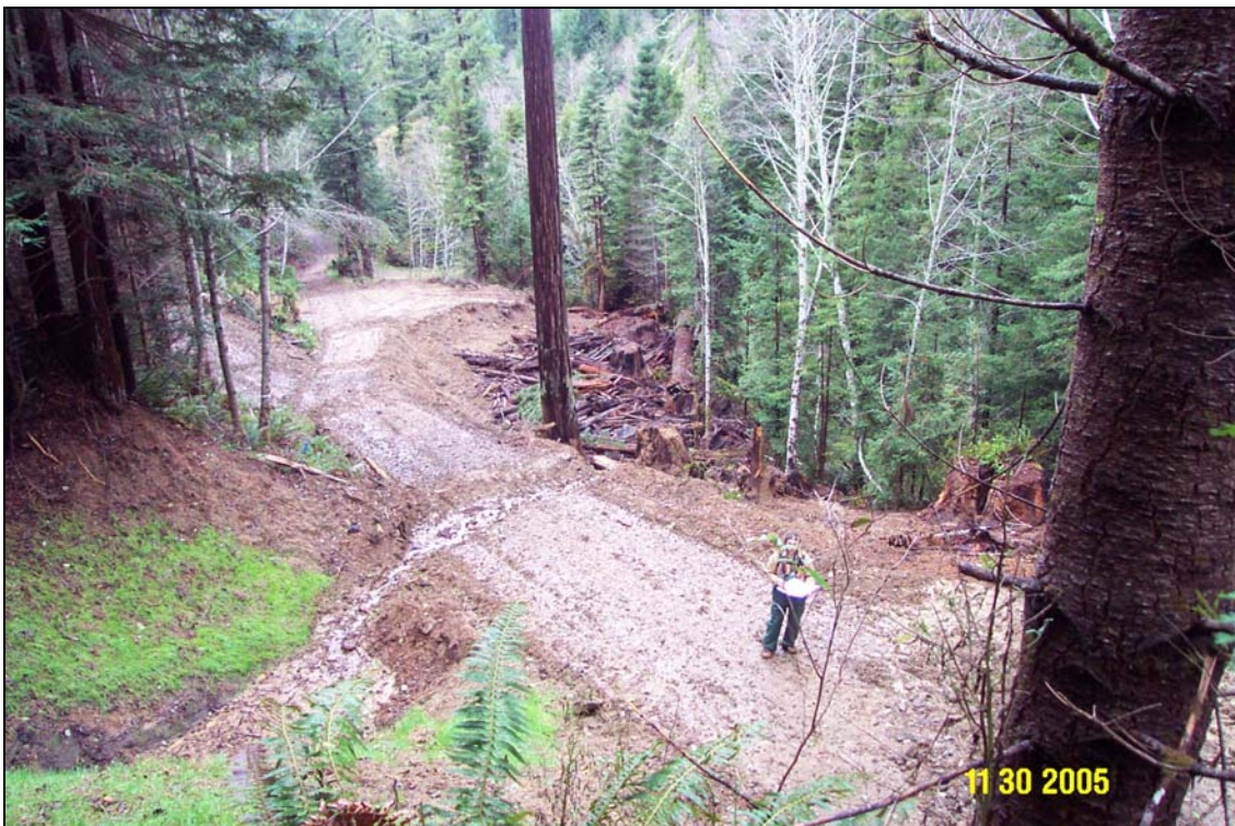
Photos 2A and 2B. R14 Road, site # 143 stream crossing, pre- and post-treatment. The picture was taken from above cutbank immediately to the right of the crossing. Note the lower and upper portions of the stream crossing have been excavated in the lower photo. A small road prism remains to allow future equipment access beyond this site. The remainder of this road is slated for decommissioning in summer 2006. Road fill, sidecast during road construction activities, was slumping and threatening to deliver to a large Class 2 stream directly down-slope. Site #142.9 is visible to the left of the Redwood tree in the top-center of the photo.
