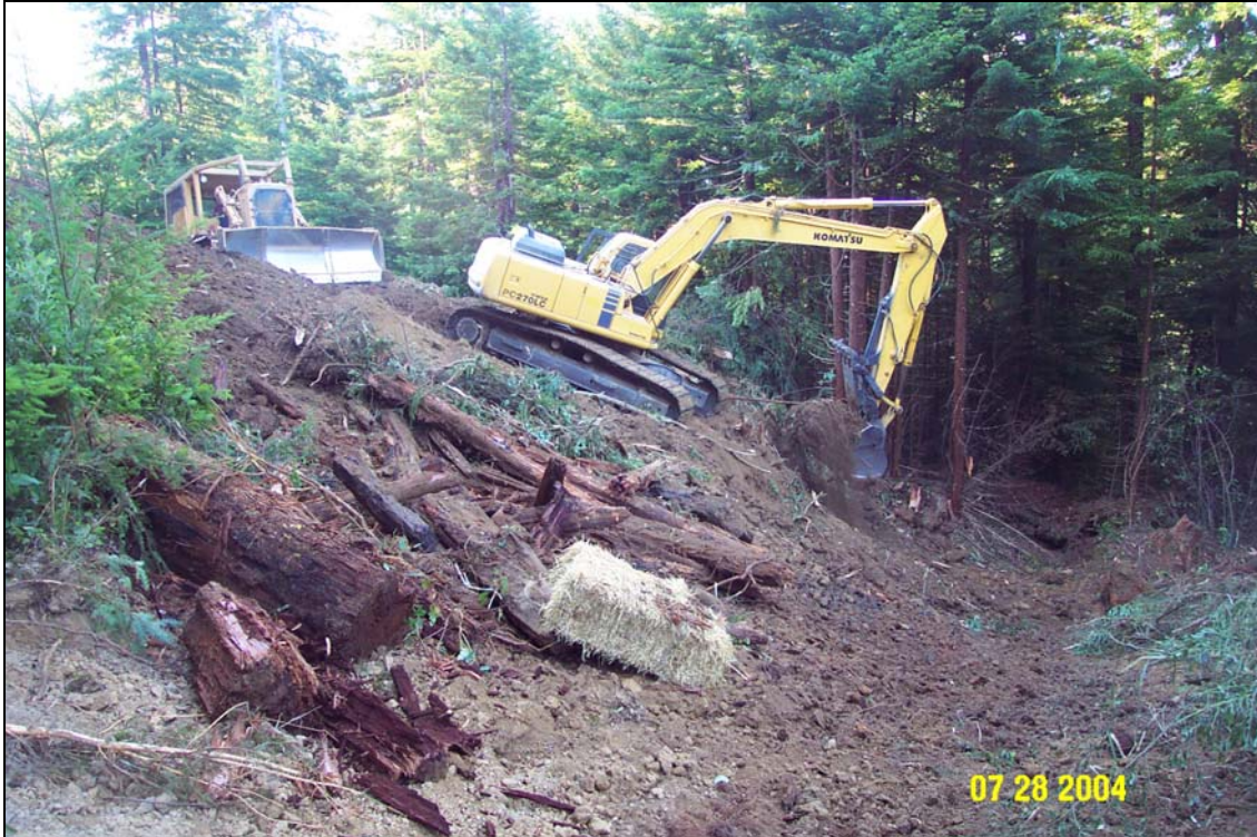
Photo #3. Site #2, U06.6966 Road, a near origin stream crossing in progress. The view is from the top of the crossing looking downstream. The excavator, digging out the fill burying the stream valley, is placing the spoils approximately at the location of the dozer, which then back bladed the material down the road off the to the left of the picture in a stable location.
