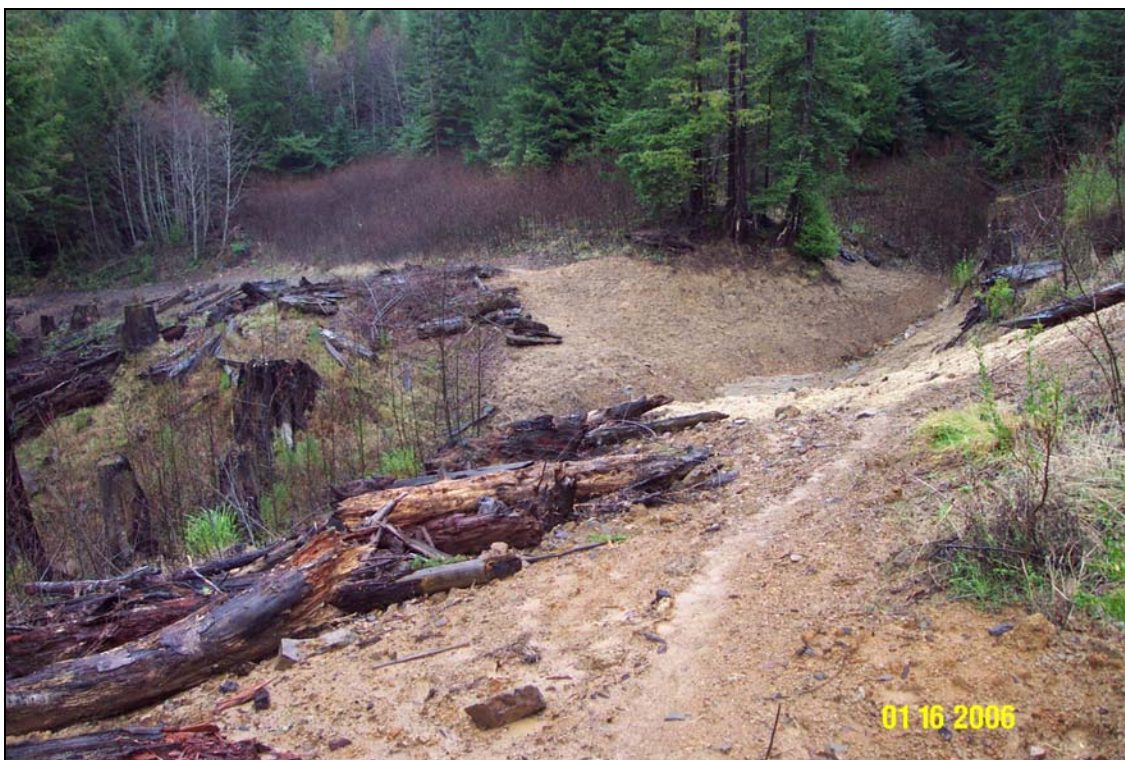
Photo 10A and 10B. R8 Road, site #122, a stream crossing, pre- and post-treatment. The view is from just above a low cutbank on the left road approach near the crossing. Upstream is to the right in the photos.
