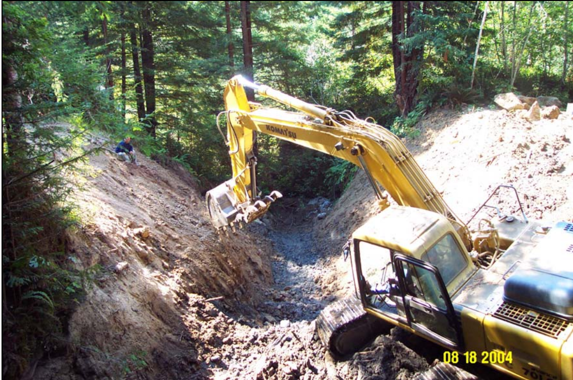
Photo 3. U06 Road, Site #1129, stream crossing, during-treatment. The picture was taken from a stump on the right sideslope of the stream valley upstream of the crossing. The view is looking downstream through the excavated road prism during the last stages of excavating the trench that the culvert was placed in. Note again the gray material in the center of the photo indicating the operator has reached natural bedrock in this area.
