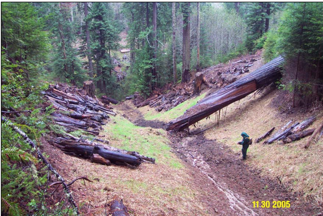
Photos 8A and 8B. R14 Road, site #145, pre and post treatment. View is approximately from the top of the excavation. Note the large woody debris, unearthed during the excavation, was placed upon the side slopes both as a protective layer as well as to catch any material that might slough off. Note the old growth stumps in the lower photo. The previously buried stumps provide guidance to the excavator operator to help locate the original ground surface.
