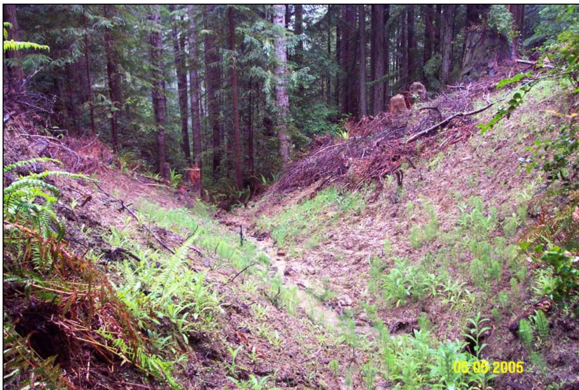
Photo #23. Site #9, almost one year after treatment. Picture taken from the top end of the excavation, looking downstream to the bottom end (bot) of the excavation.
