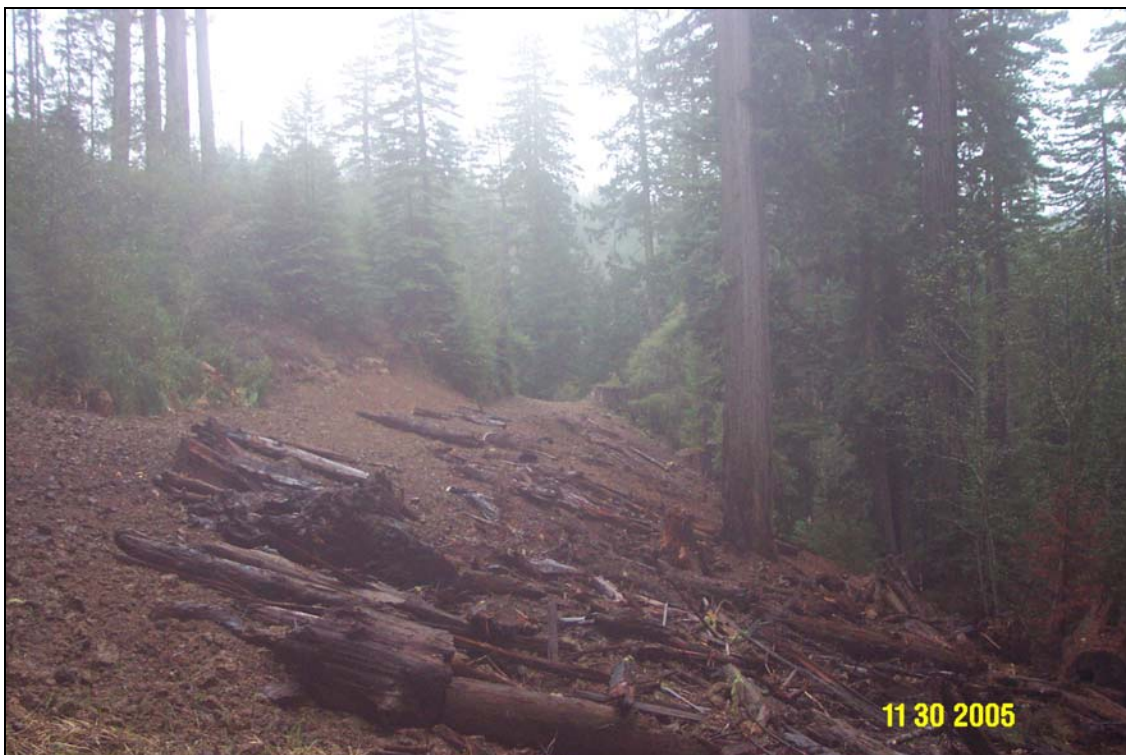
Photos 10A and 10B. R14 Road, site #145.1, another landslide site, pre- and post-treatment. View is from the right end of the site. Again, note the site has been completely outsloped.
