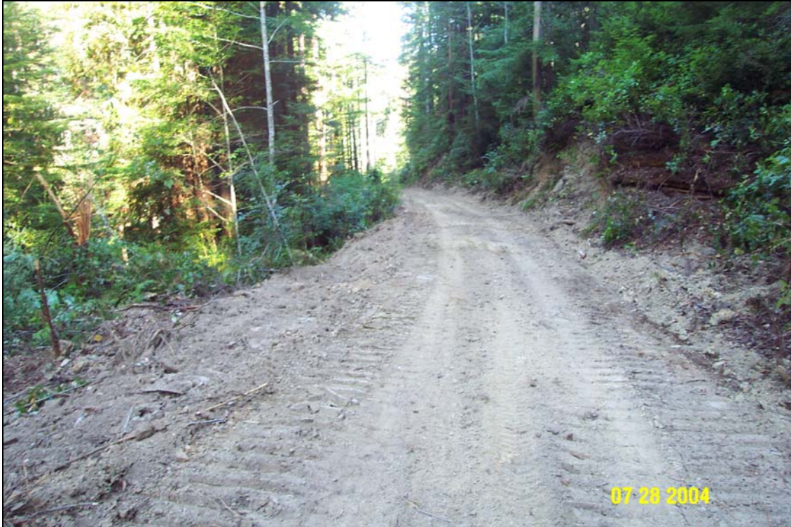
Photo 1. U06.6966 Spur 1 Road, Site #19, stream crossing, pre-treatment. The picture was taken from the left road approach looking across the crossing down the right road approach.
