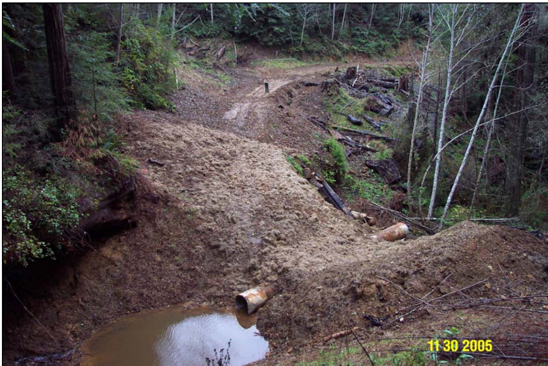
Photos 5A and 5B. R14 Road, site #144, pre and post treatment. This site had also been partially excavated as part of an earlier decommissioning project the previous year. Additional fill was excavated from the crossing and a temporary culvert and downspout installed to pass flow through the crossing. Site #144.2, a small stream crossing site, located in the top center of the photos (where the person is standing in the lower photo) was likewise partially treated with additional fill excavated from the road prism itself through the crossing.
