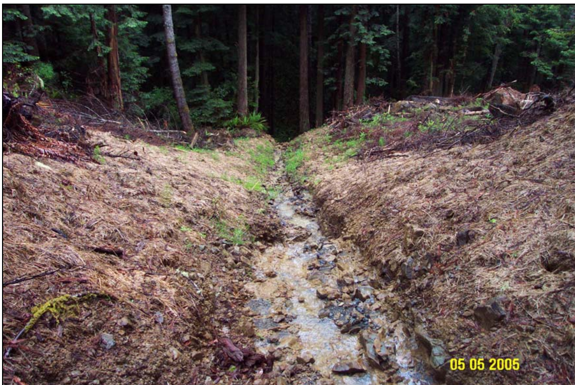
Photos 7A and 7B. U06.6966 Spur 1 Road, Site #17, stream crossing, pre- and post-treatment. The picture was taken from approximately the middle of the original landing surface, looking downstream. The bottom photo was taken after the site had gone through its first winter post-excavation.
