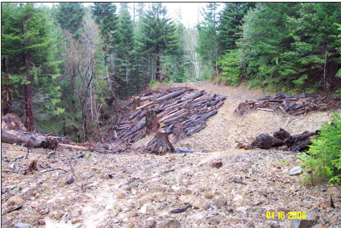
Photo 6A and 6B. R8 Road, site #121.5, a stream crossing, pre- and post-treatment. The picture was taken from the left road approach looking across the crossing. Note the abundance of large woody debris unearthed during the excavation, placed on the newly excavated side slopes.
