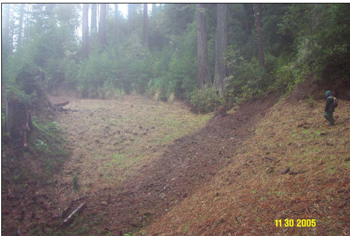
Photos 14A and 14B. R14 Road, site #145.3, pre and post treatment. This was the farthest site out the road, located a short distance before the terminal landing. The lower portion of this site had been partially excavated as part of an earlier decommissioning project the previous year.
