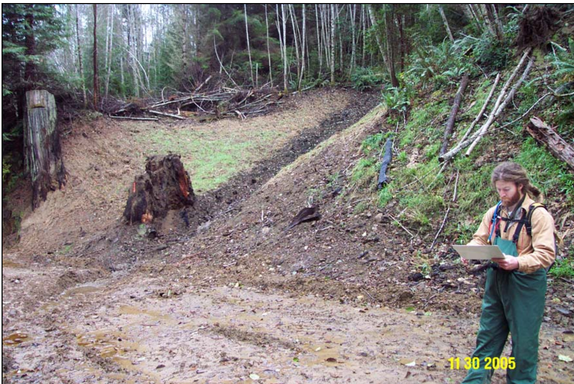
Photos 3 and 4. R14 Road, site #143.2, pre and post treatment. The lower portion of this site had been excavated treated as part of an earlier decommissioning project the previous year. The upper portion of this site had a large break-in-slope with fill over-steepened and saturated above the road. The upstream portion of this site was excavated to the natural channel grade.
