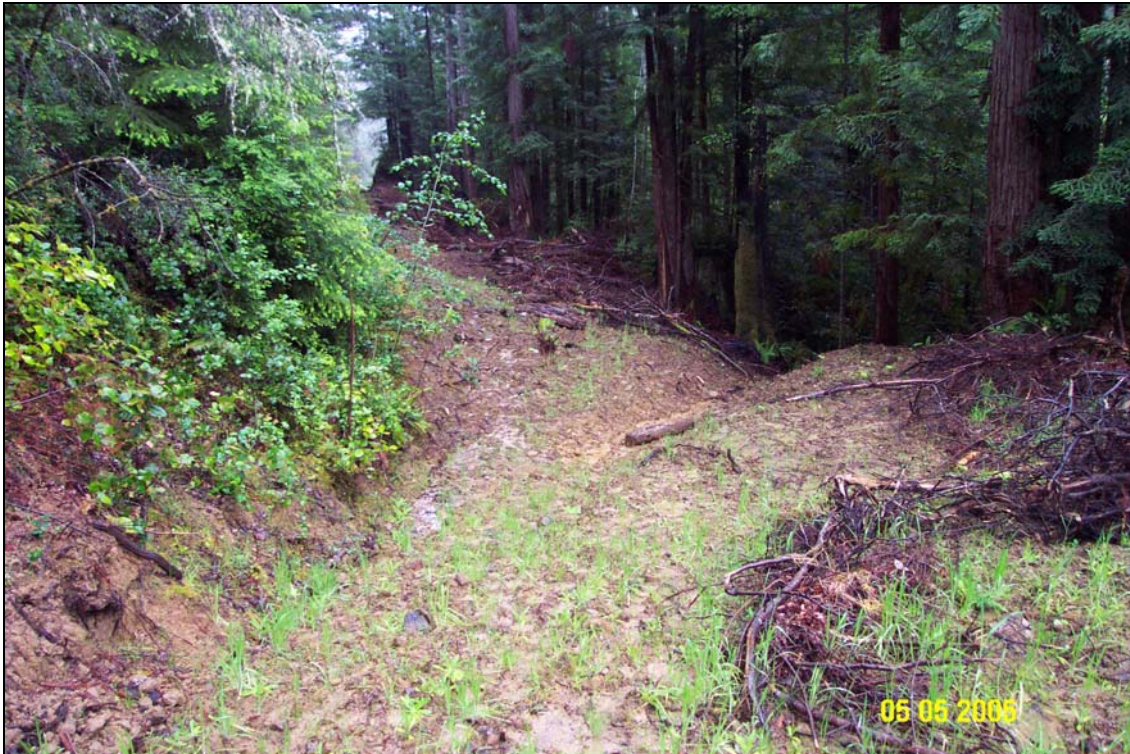
Photo #22. Excavated swale catching spring flow on right approach to site #8., approximately one year after treatment. Site #8 is obscured just beyond the slash pile in the top-center of the photo.
