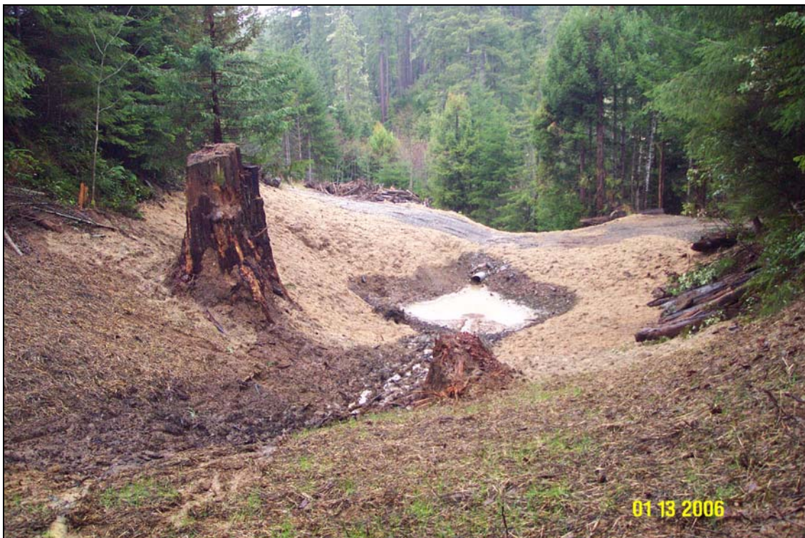
Photos 4A and 4B. R8 Road, site #121.1 during, and post-treatment. The view is from near the top of the excavation looking down to the road. Note the inlet of the new culvert and the large critical dip installed until the crossing can be fully decommissioned
