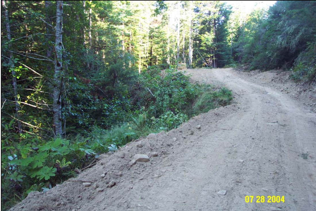
Photo #18A. Site #7, a potential landslide on the U06.6966 Road, pre-treatment. View is from the left side of the site looking beyond across the site toward the right approach. The upper reaches of the north fork of the Little South Fork Elk River is located directly below the site. Note the over-steepened edge of the road at the bend approximately center-right in the photo. A portion of the road bench had already failed and delivered to the creek at the base of the inner-gorge slopes below, but additional unstable material remained perched with potential to deliver additional sediment into the stream.
