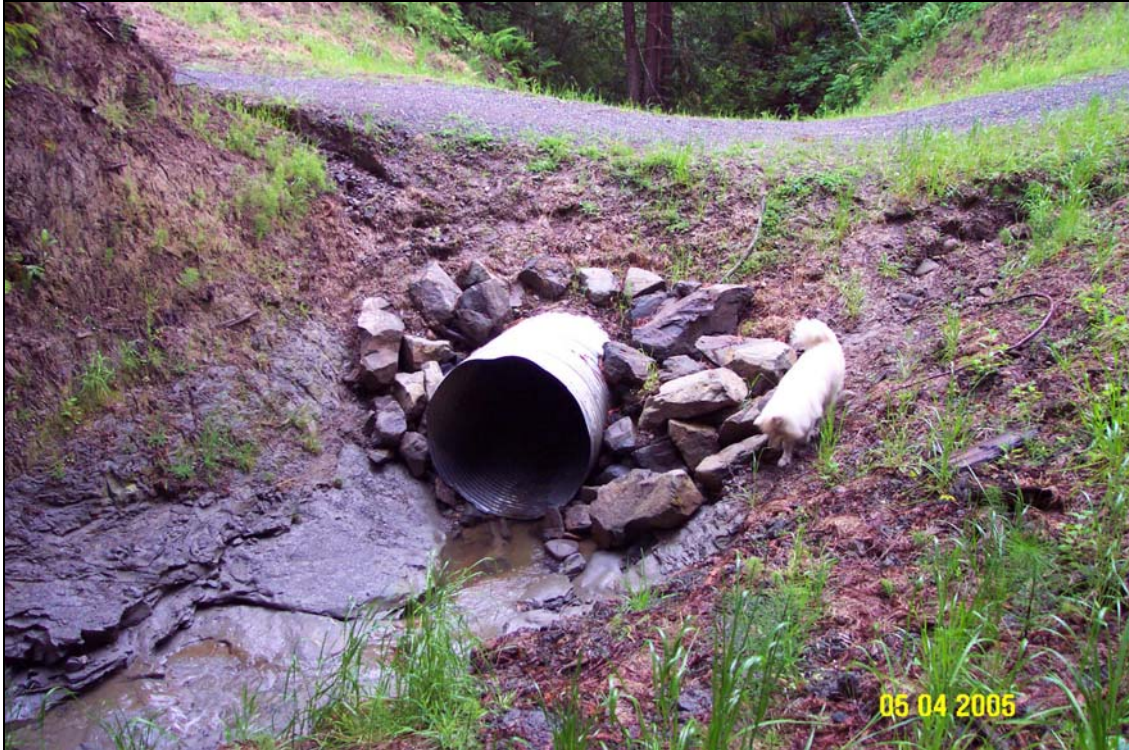
Photo 6. U06 Road, Site #1129, stream crossing, post-treatment. The picture was taken from the right side-slope above the culvert inlet looking downstream toward the inlet in the foreground and the lowered stream crossing. Note the siltstone bedrock surfaces in the channel banks and bottom just upstream of the inlet.
