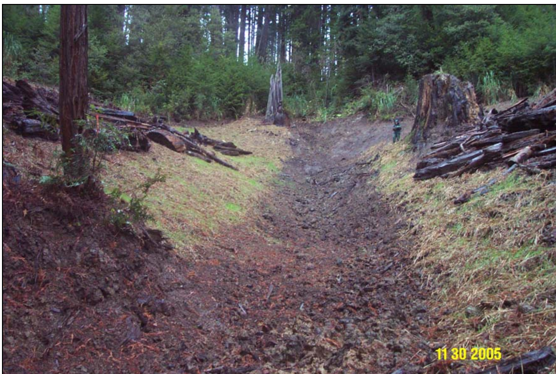
Photos 12 and 13. R14 Road, site #145.2, post treatment. The views are from the lower end of the site, looking up to the top of the excavation.
