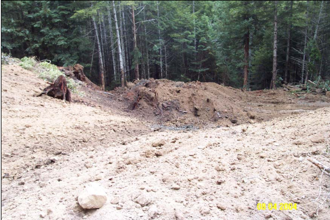
Photo #12. The lower portion of stream crossing #5, U06.6966 Road, in progress. The view is from the upper segment of the old switchback looking downslope toward the bot (hidden from view by the pile of material in the center of the photo). The lower road approach meets the site in the right-center of the photo.
