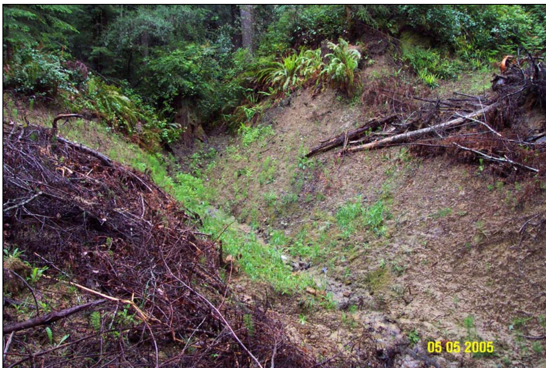
Photo #24. Site #9, almost one year after treatment. Picture taken from the lower end of the excavation above the right side-slope, looking upstream at the top of the excavation.
