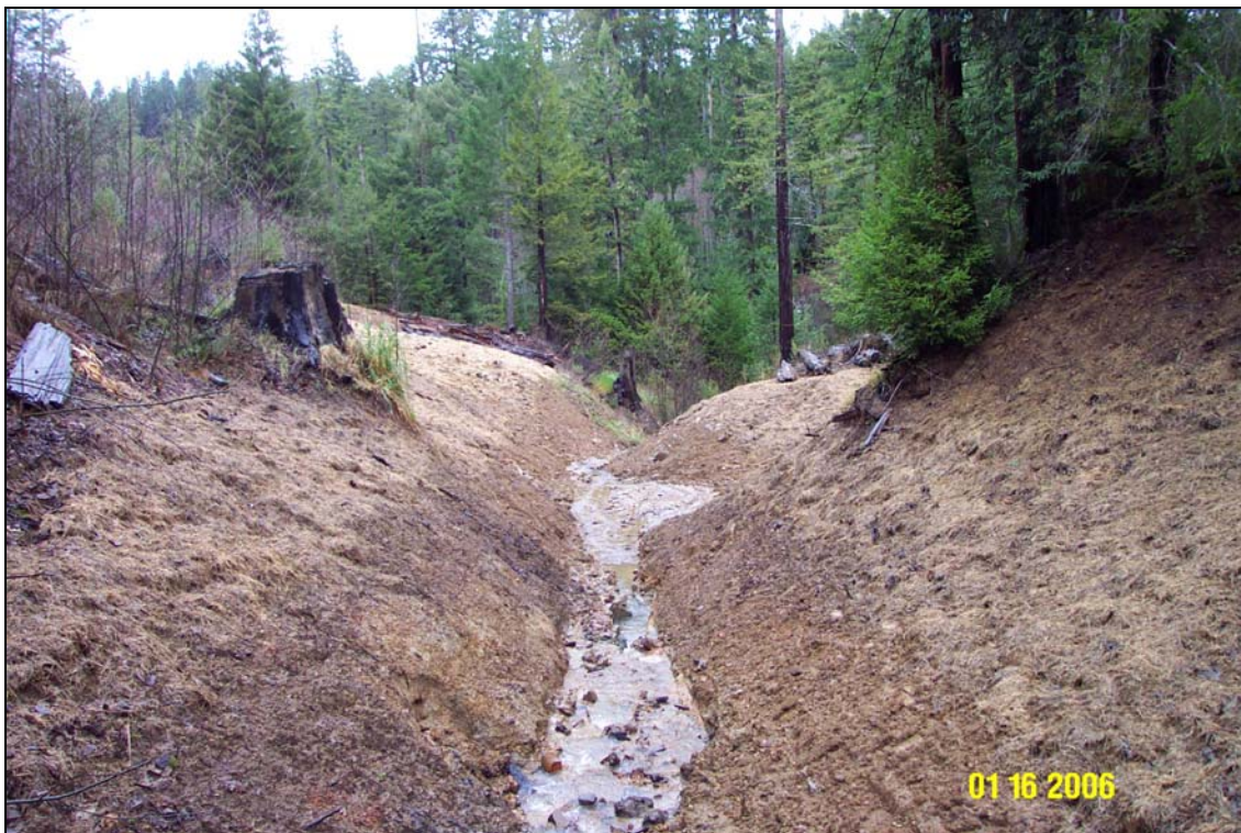
Photo 11A and 11B. R8 Road , site #122, during- and post-treatment. The view looking downstream from just below the top of the excavation. Note the dump truck in the top photo, marking the location of the road prism.
