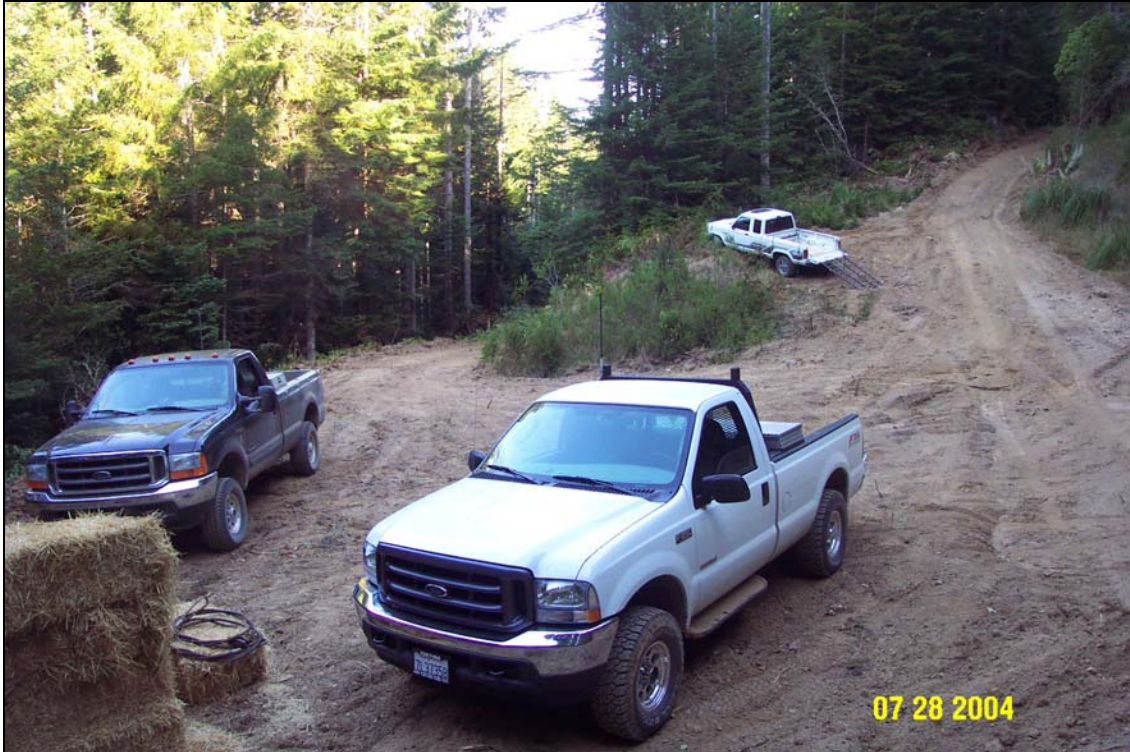
Photo #10. Stream crossing site #5 in the foreground, and stream crossing site #4 in the upper right of the photo, both pre-treatment. Site #5 was located within a tight switchback in the road and involved a long excavation and thousands of cubic yards of road-fill that had to be end-hauled from the work site.
