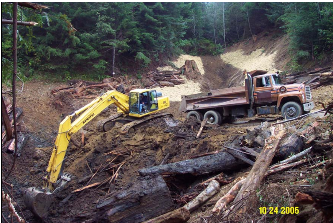
Photos 8 and 9. R8 Road , site #121.5 during-treatment. As the excavation progresses, the excavator gets deeper and more difficult to access by dump truck, so earthen ramps are constructed (top photo) to allow continued access by the dump trucks. On the R8 Road, there was a scarcity of adequate spoil disposal areas on the road itself, so most spoils were endhauled off-site to a stable storage location.
