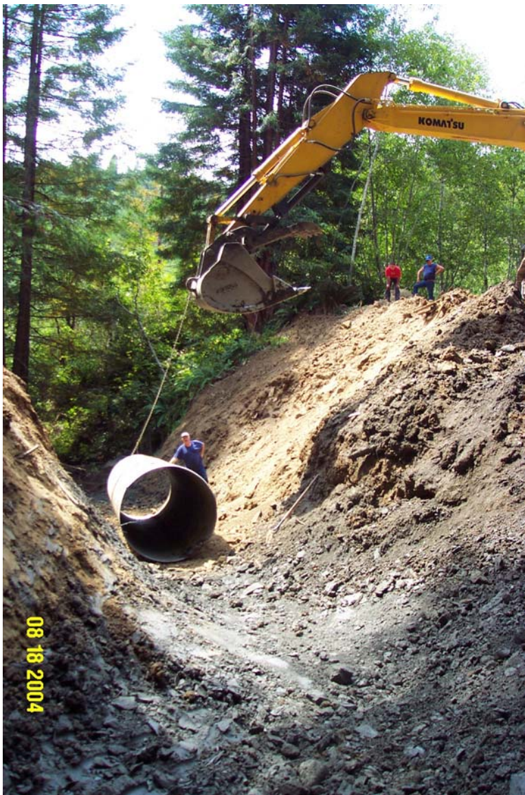
Photo 5. U06 Road, Site #1129 during the crossing upgrade. The excavator is placing the first section of culvert. View looking downstream from approximately the location of the soon to be installed culvert inlet.
