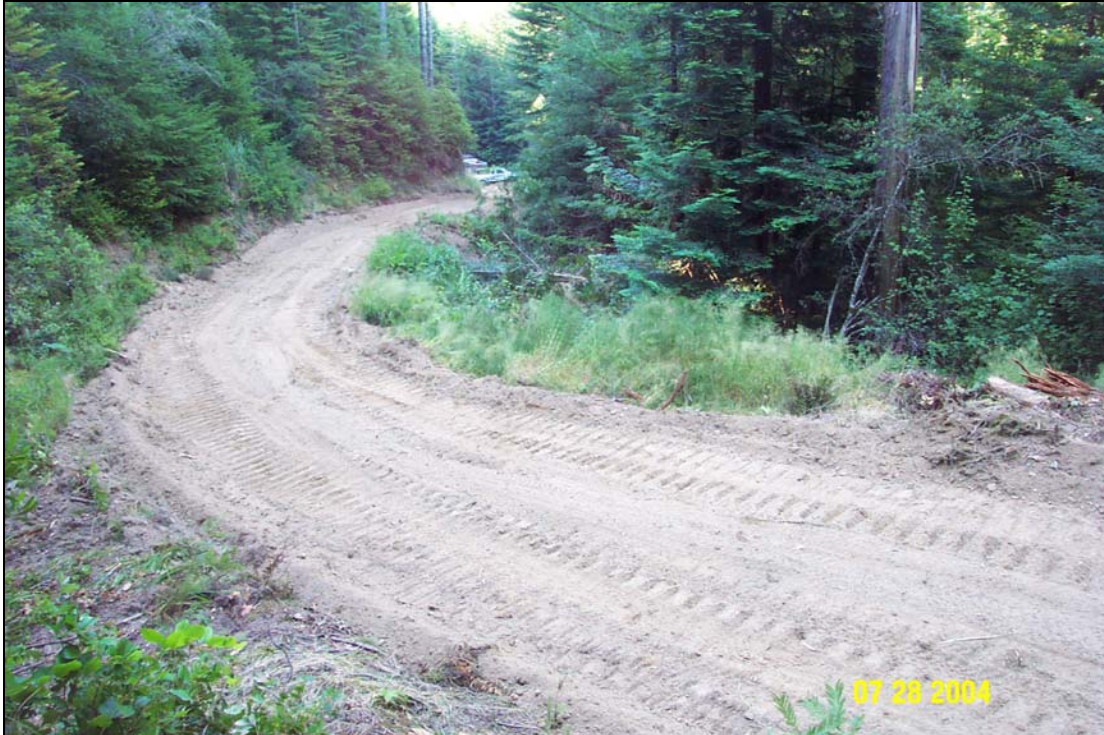
Photo #5A. Site #3, stream crossing on the U06.6966 Road, pre-treatment. View is from the right side of the crossing looking toward the left road approach. Prior to treatment, the stream had been diverting down the left road, causing a long gully down the hillslope below. Note the tree trunk in the upper right corner of the picture for comparison with the photo below.
