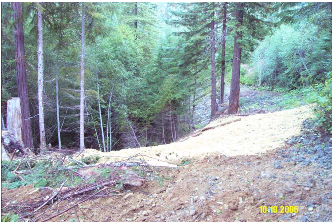
Photo 14A and 14B. R8 Road, site #122.1, a landslide site, pre-, and post-treatment. The view is from the left end of the site looking towards the right end of the site. The site was completely mulched with rice straw due to its proximity to the creek. This site had been partially treated as part of a different project the previous year, but still contained potential to deliver sediment to mainstem Salmon Creek, located immediately below the site. Note the road has been completely outslipped.
