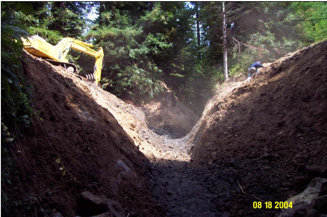
Photo 4. Site #1129 during the crossing upgrade. The excavator has cleaned out the trench to the natural stream grade and is ready for the culvert installation.
