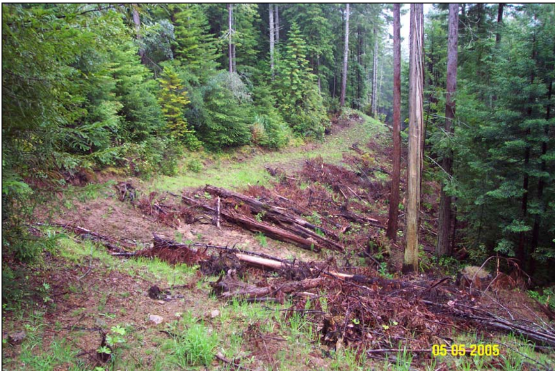
Photo #5B. The same stream crossing, post-excavation. The view is similar to the last photo. Abundant springs along the cutbank of the left road approach forced excavated road fill to be endhauled to a stable spoil disposal area using dump trucks. Note the left road has been completely outslopped, with slash placed on the freshly excavated surfaces except for a small "trail" along the upper most side of the disturbed area.
