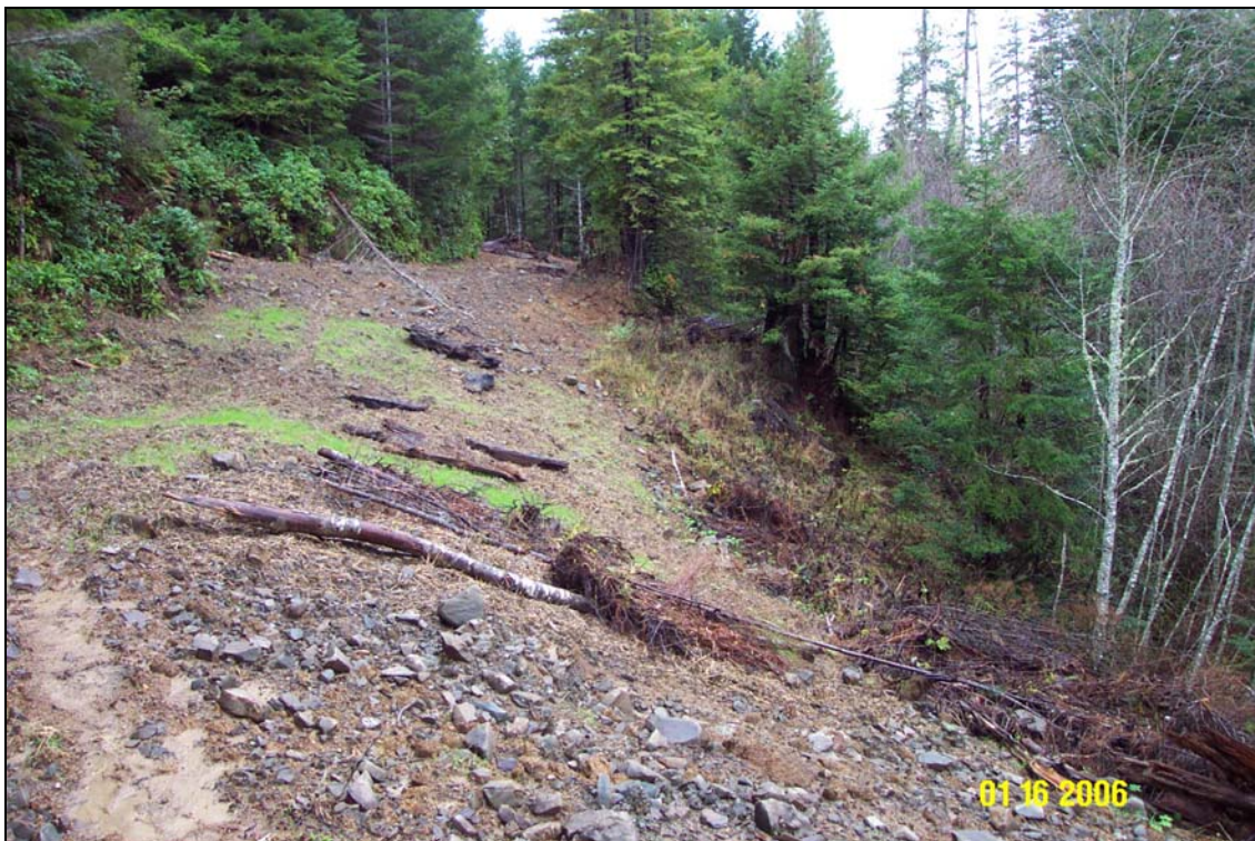
Photos 5A and 5B. R8 Road, site #121.2, a landslide site during, and post-treatment. The view is from near the right end of the site looking back towards the start of the site, located where the quad is sitting in the top photo. This site had been partially treated as part of a different project the previous year. Note the road has been completely outsloped by excavation and endhauling most the material off-site, with a small portion placed upon the cutbank to complete the outslope.
