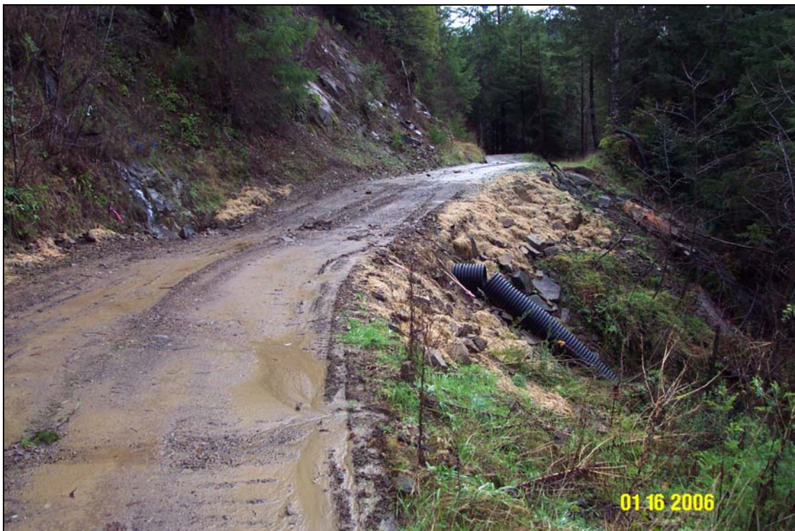
Photos 1A and 1B. R8 Road in the Salmon Creek watershed. Site #121, a stream crossing, pre- and post-treatment. The picture was taken from the right road approach looking across the crossing. Note the new plastic culvert and downspout installed as a temporary crossing until the road can be completed, slated for decommissioning in summer, 2006. This site is located on steep inner-gorge slopes directly above Salmon Creek.
