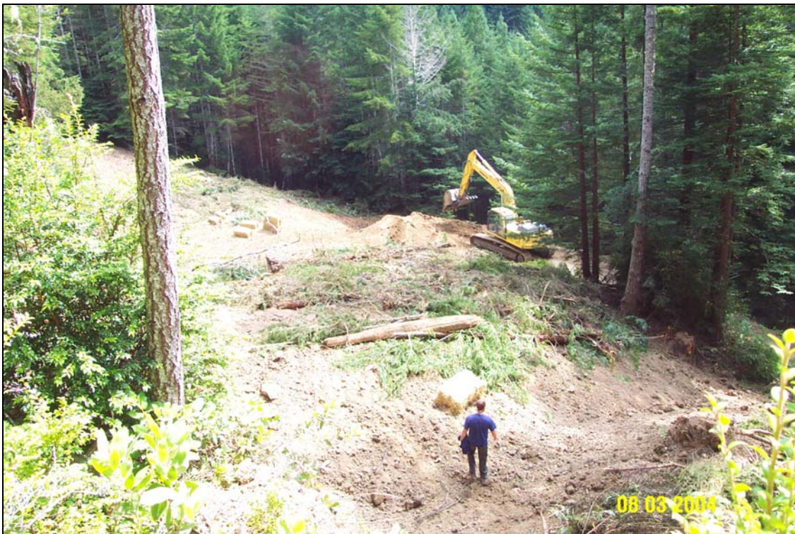
Photo #8. Stream crossing #4, U06.6966 Road, immediately after treatment, located where the man in the photo is standing. The view is from above the top of the excavation looking downstream. Note the excavator working on the lower portion of stream crossing site #5 near the center of the photo.
