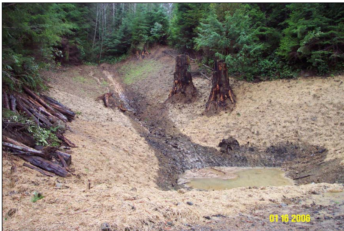
Photos 3A and 3B. R8 Road, site #121.1 during, and post-treatment. The view is from the road looking towards the top of the excavation. Note the large woody debris unearthed during the excavation was placed on the sideslopes to help catch any material that might slough off from an especially springy side slope. The large old-growth Redwood root ball visible in the top photo was unearthed during excavation of fill from the stream valley above the road. These can be used for in-stream fisheries projects incorporating large wood.
