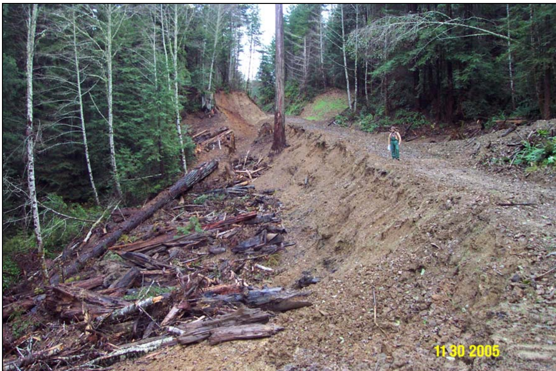
Photos 1A and 1B. R14 Road, site #142.9, landslide, pre- and post-treatment. The picture was taken from a landing on the left side of the site. Road fill, sidecast during road construction activities, was slumping and threatening to deliver to a large Class 2 stream directly down-slope. View is from the left side of the site. Site #143 stream crossing is located near the end of the site at the large Redwood tree in the top-center of the photos.
