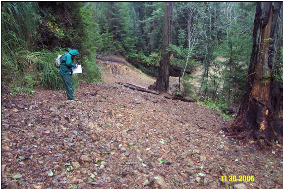
Photos 7A and 7B. R14 Road, site #144.1, landslide, pre- and post-treatment. View is from the right end of the site, looking back towards site #144 stream crossing in the distance. Note the site has been completely outsloped, by placing some of the spoils against the cutbank.
