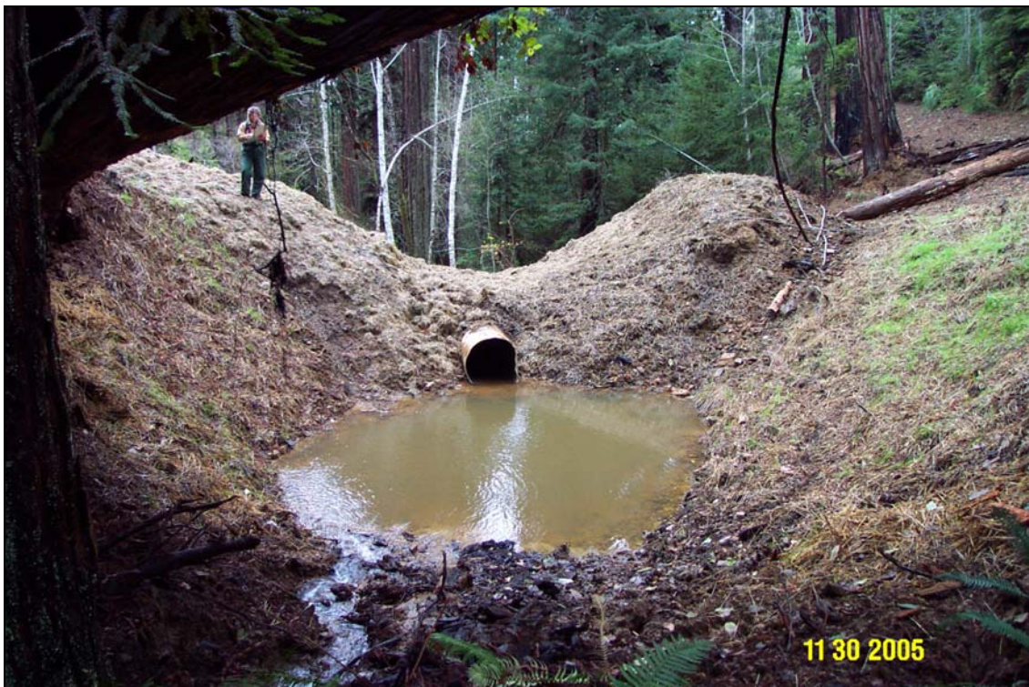
Photos 6A and 6B. R14 Road, site #144, pre and post treatment. View is approximately from the top of the excavation. Note the right road approach has been completely re-contoured in the lower photo. The entire road prism beyond this site was completely re-contoured between sediment delivery sites, funded by the BLM. All sites and road reaches from this site to the beginning of the road, is slated for completion in summer 2006.
