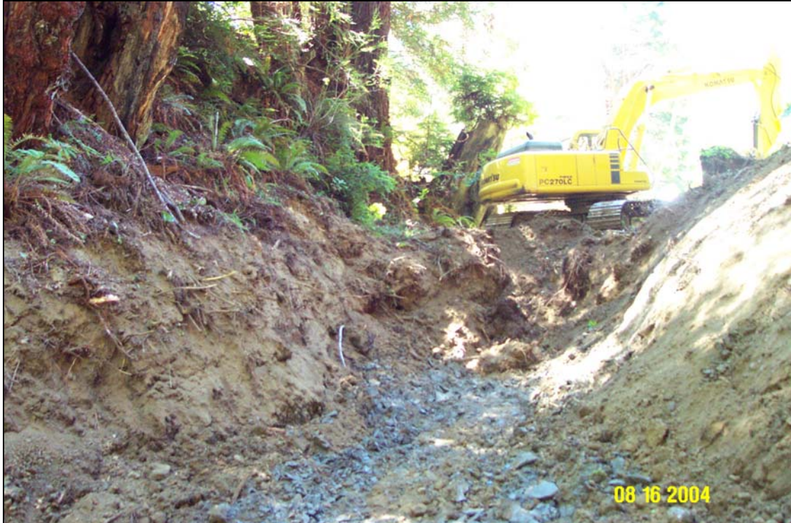
Photo 2. The same stream crossing during treatment. The photo was taken from just downstream of the top, looking downstream. The excavator is sitting just upstream of the inboard side of the crossing, cleaning out stored sediment from the stream valley. The gray material in the new channel bottom is siltstone bedrock of the Wildcat Formation, a rather soft but indurated material.
