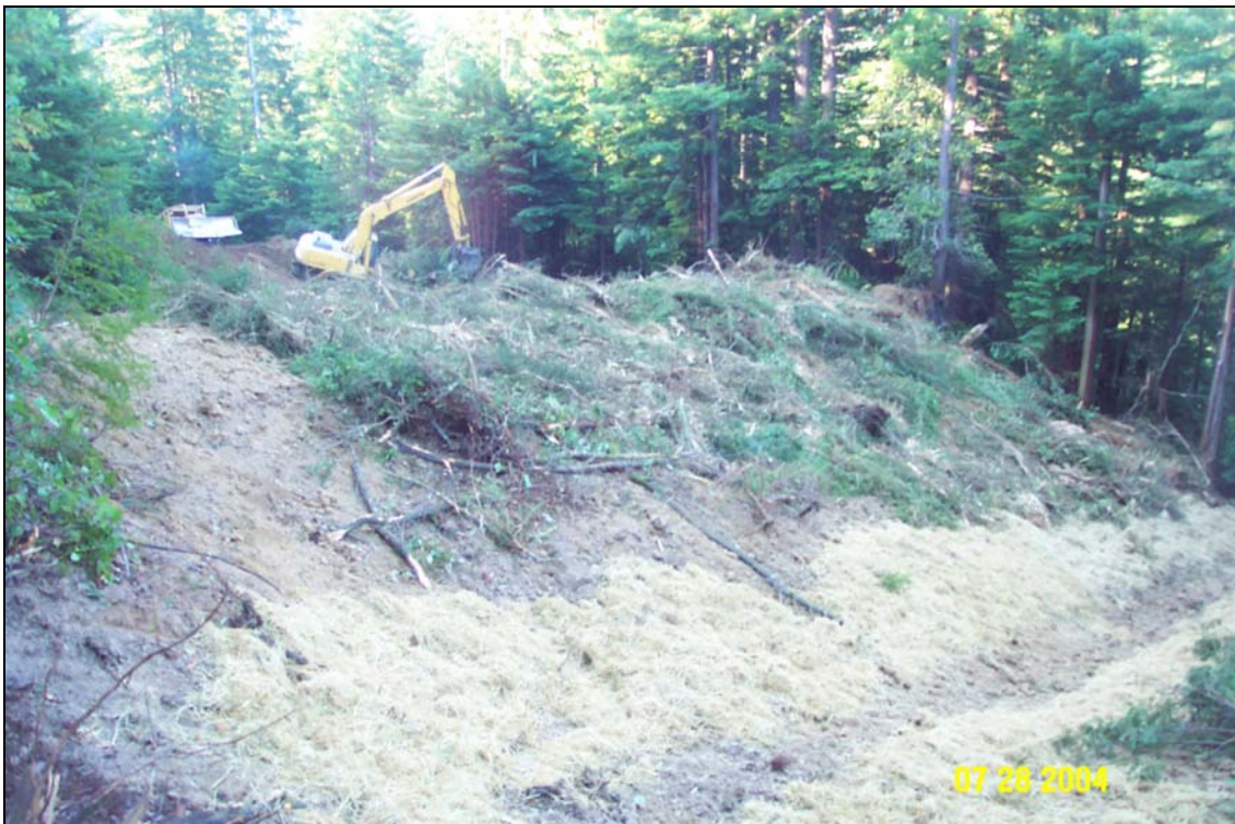
Photo #2. Site #1, U06.6966 Road, post-treatment. Spoils were stockpiled on the left side of the crossing and covered with slash to protect the surface from rain-splash. Straw mulch was placed along the sides of the excavated channel to help catch fines generated from the fresh surface. The excavator and dozer are working on site #2, in the upper left of the photo.
