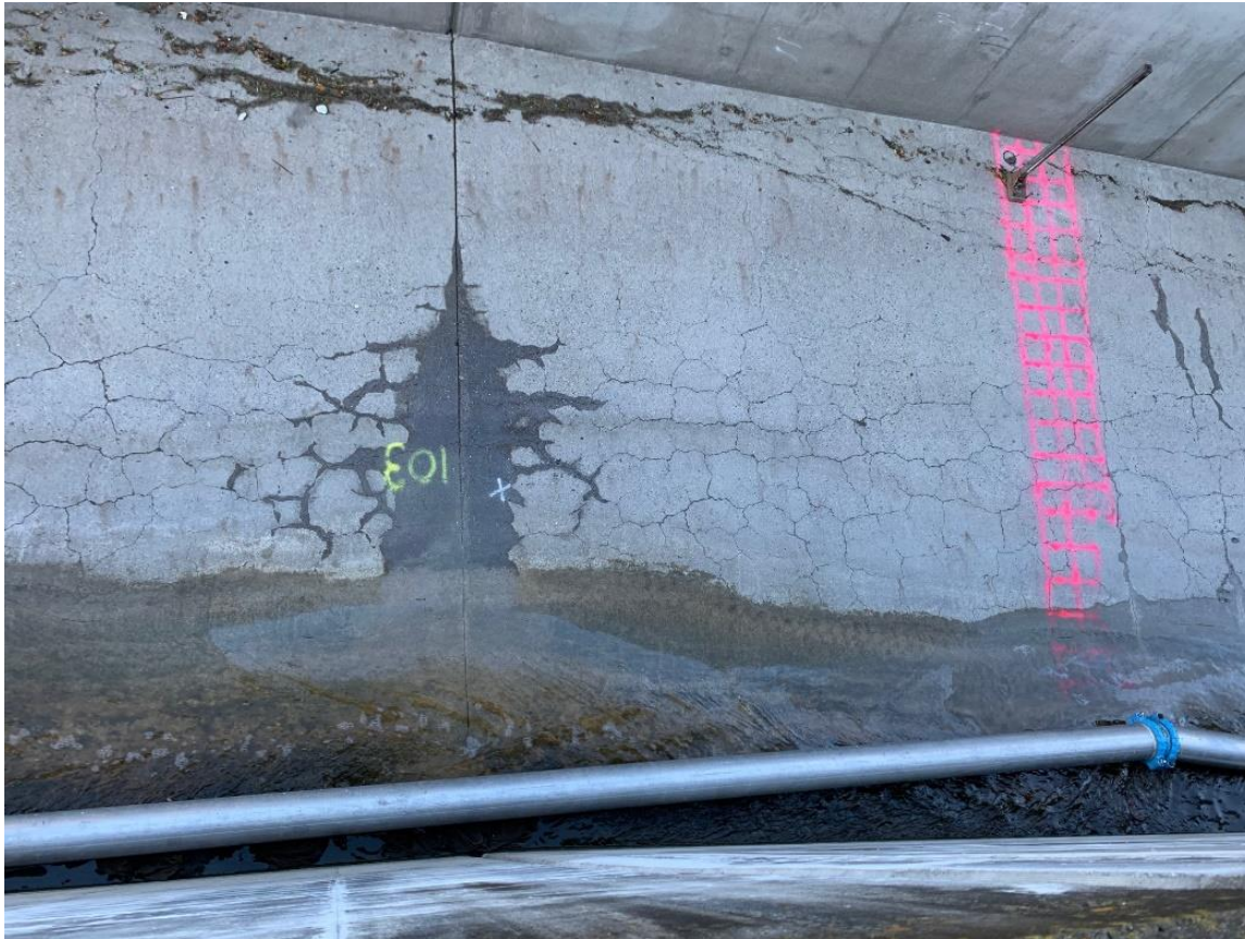
Figure 5. Photo from top view of the concrete channel at Bypass Area where product sheen is observed discharging into the surface water.
