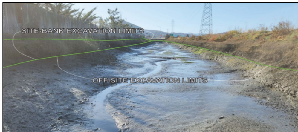
Figure 2: Offsite Ditch Prior to Remediation
