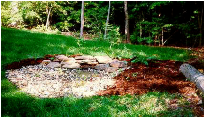
Newly planted rain garden. Note the water in the depression.
