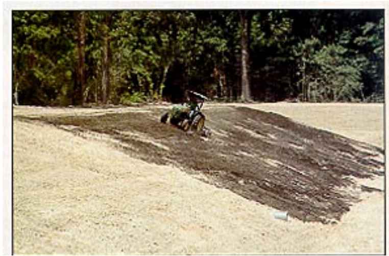
Compost being incorporated on an embankment of the Oaks of Terra Nova West subdivision detention basin.
