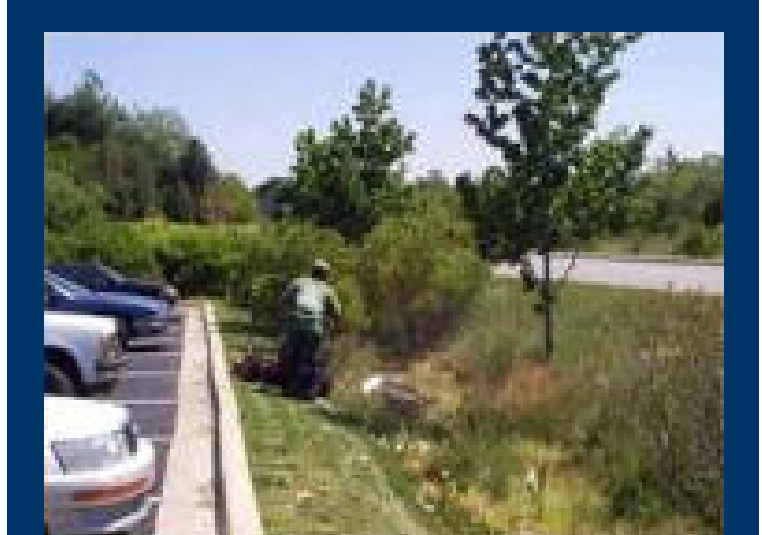
Bioswale Maintenance Source: LID Center
