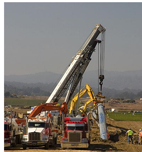
In September 2007 a 1,400-foot horizontal directional drill (HDD) was used to install a 36-inch diameter steel pipe under the Pajaro River to deliver irrigation supplies to Monterey County.
