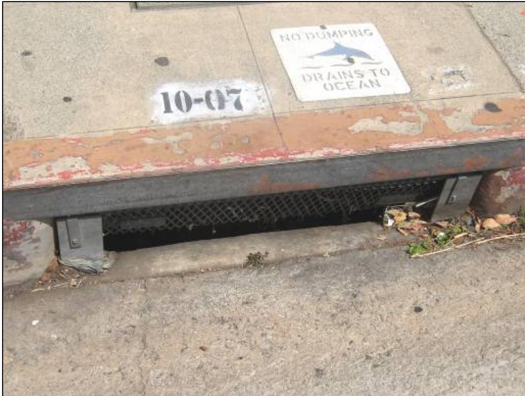
Excluder stuck partially open apparently not due to trash wedged in the opening.
