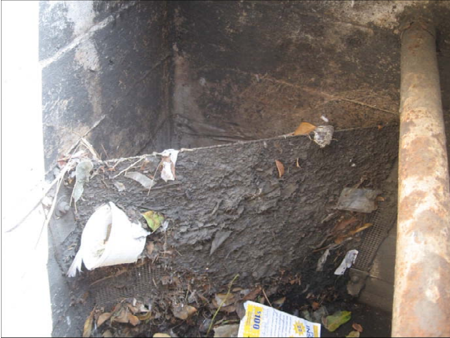
Vertical insert with sediment and debris stapled to the surface. About 10% of the screen area is visible. Materials clearly passing downstream. Less than 1" of material in the catch basin.
