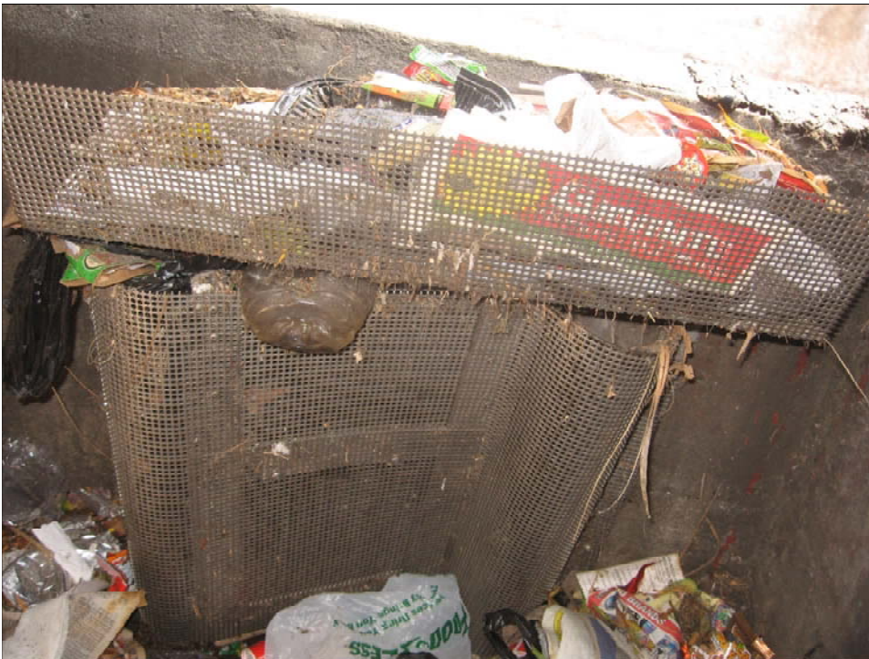
A vertical insert without much material in the screen, but it appears to have buckled under pressure from water pooled in the catch basin. Debris tray is installed under inlet because pipe exits toward street. About 2" of material on the floor of the catch basin.
