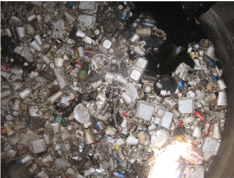
View of 10' diameter CDS separation chamber with a floating Styrofoam mat about 1' thick. Park Grove System.
