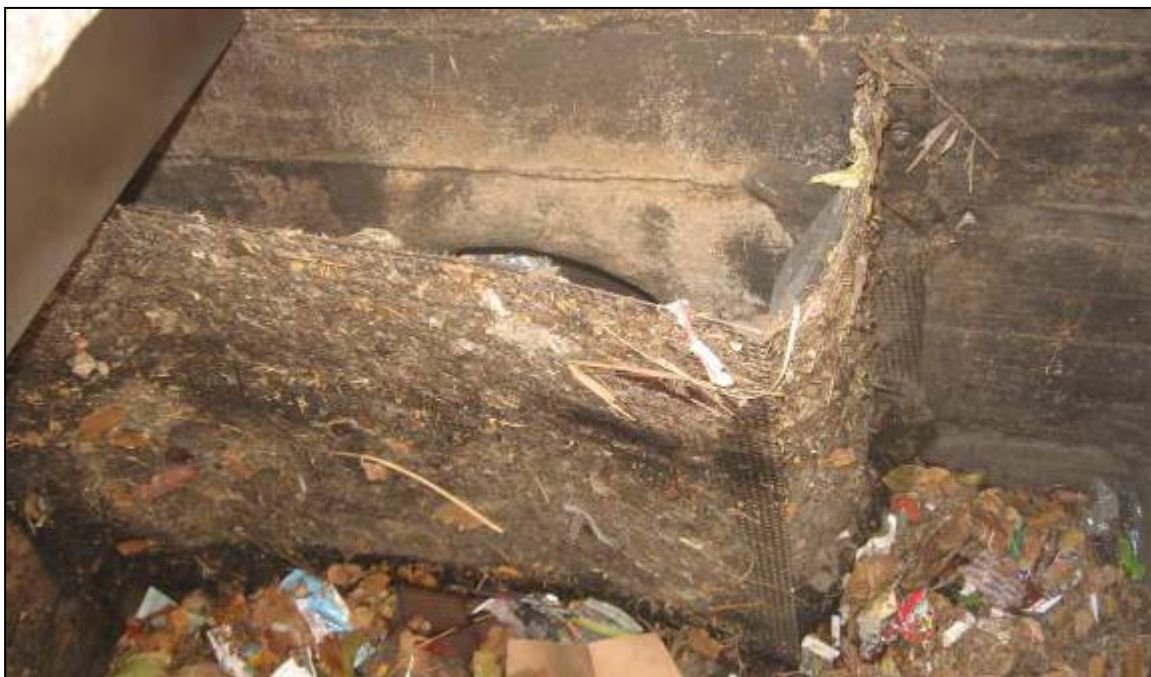
Vertical insert screen totally occluded with evidence of materials passing downstream. About 1"-2" of material on the floor of the catch basin.
