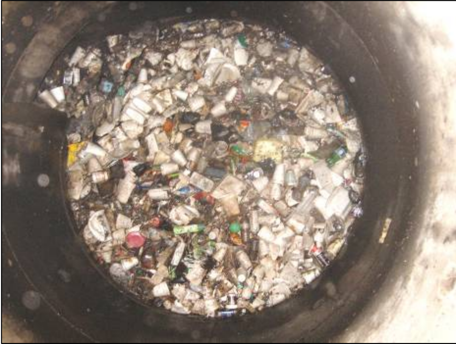
View of 7' diameter CDS separation chamber with a floating Styrofoam mat about 1' thick. Westlake System.
