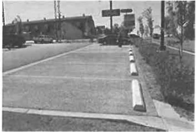
Permeable pavement – parking stalls
