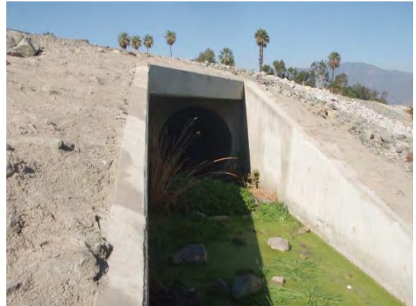
2. 15 feet from outfall
