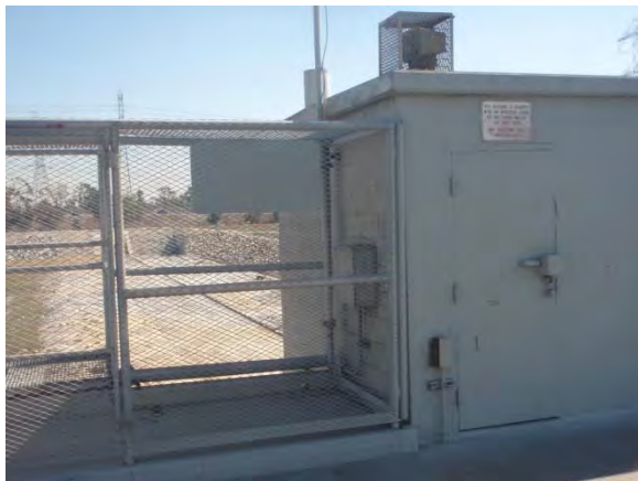
1. Unit connected to outfall from bike path
