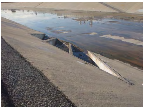
5. View of outfalls from bike path
