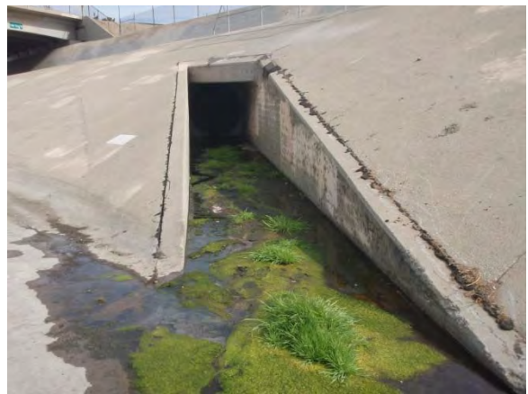
4. 15 feet from outfall
