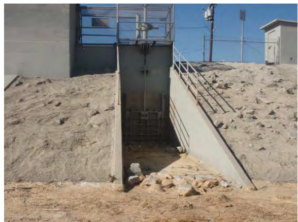
4. 15 feet from outfall
