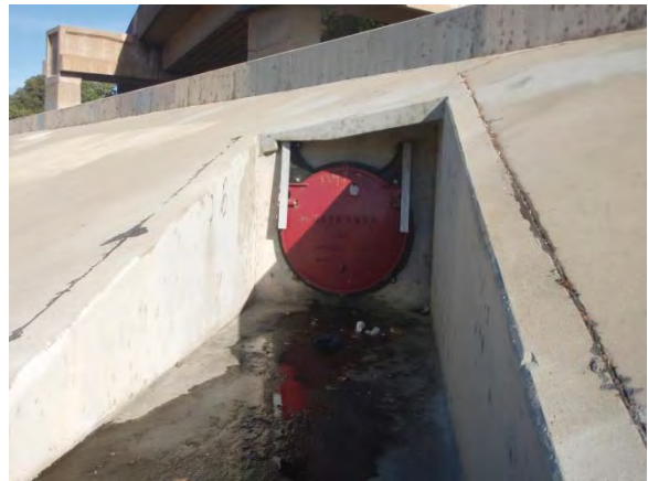
2. 15 feet from outfall
