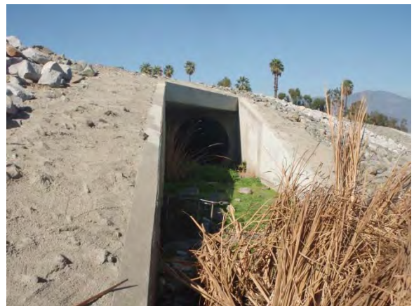
4. 20 feet from outfall
