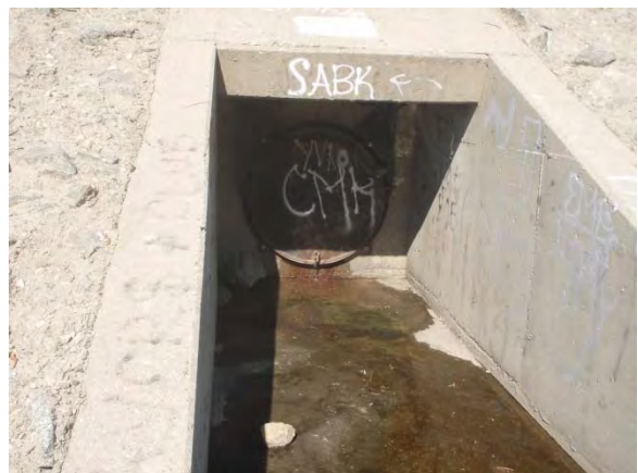
4. 15 feet from outfall
