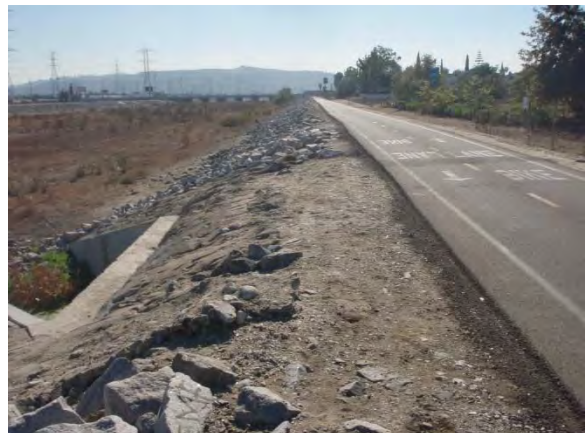
4. 15 feet from outfall
