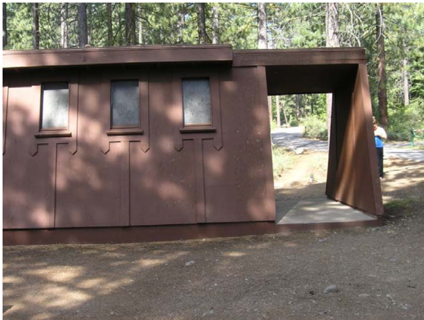
Figure 1-6. Non-universally accessible restroom facility with extensive deferred maintenance.
