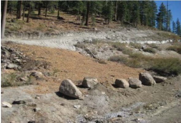
Photo taken on October 5, 2016 prior to placement of Water Board required temporary BMPs to prevent soil from leaving the construction area.
