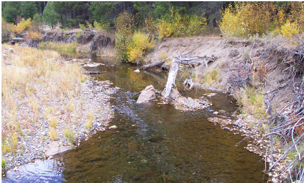
Figure 4-21. Typical failing outside bend along the lower 4 km of Blackwood Creek. This site is rated “high” in fine-sediment availability due to the bank height and length of reach failing. Similar sites, with lower banks, are rated “moderate.”
